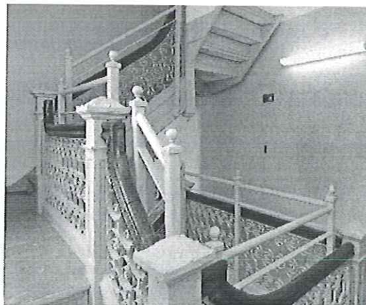
Right: Revised railing that better relates to historic design and meets the Standards.
