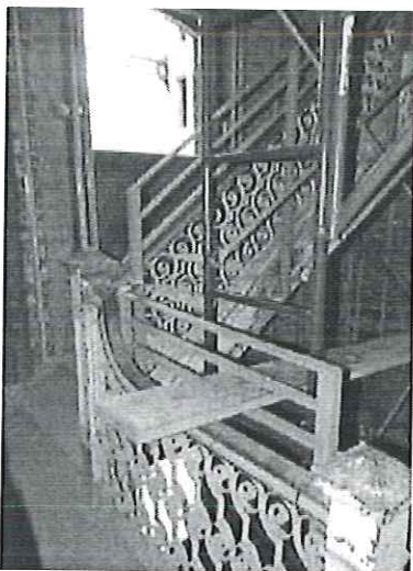
Left: Sample installation of railing modification first proposed did not meet the Secretary's Standards.
