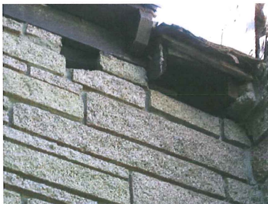
Rot and noticeable openings in eaves
