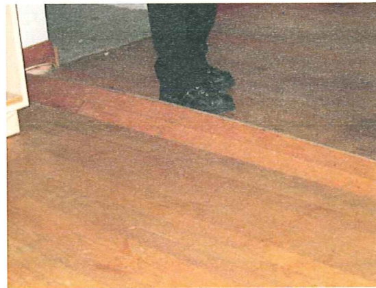
Swollen hardwood floors in main room
