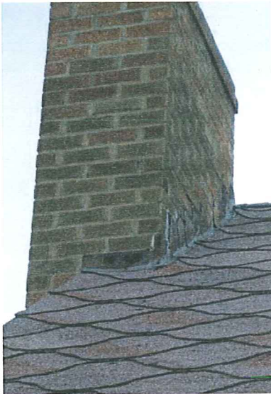
Caulk failing between flashing and masonry and flashing and asphalt shingles
