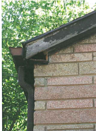
Rot and noticeable openings in eaves
