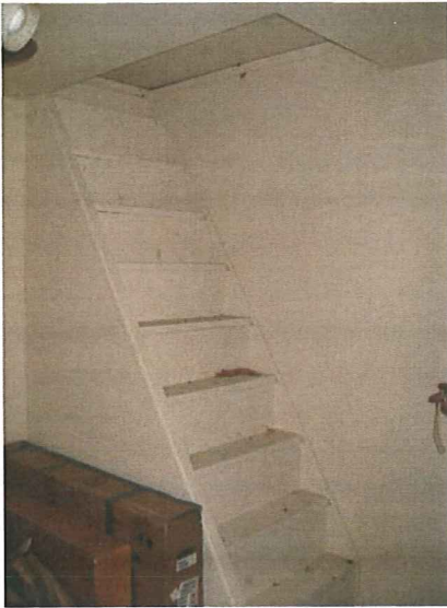
Non-code compliant stair to attic; would have to be removed or renovated
