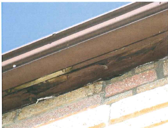
Rot at wood eave/masonry interface
