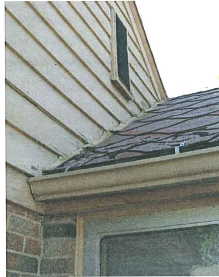
Deterioration of caulking and missing flashing at front porch roof interface with exterior wall
