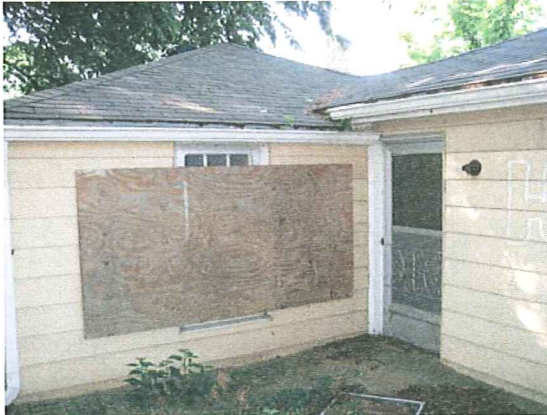
Damage to metal siding and detail of siding continuing below grade
