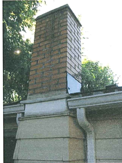
Water staining and attempts to correct at masonry chimney and metal siding interface
