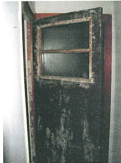
Mold on door leading to basement
