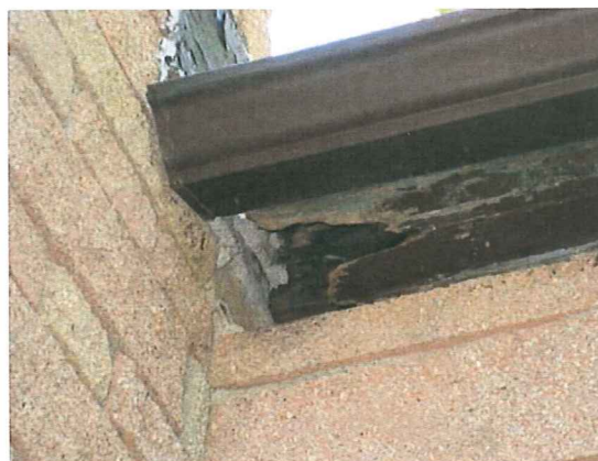
Rot at wood eave/masonry interface
