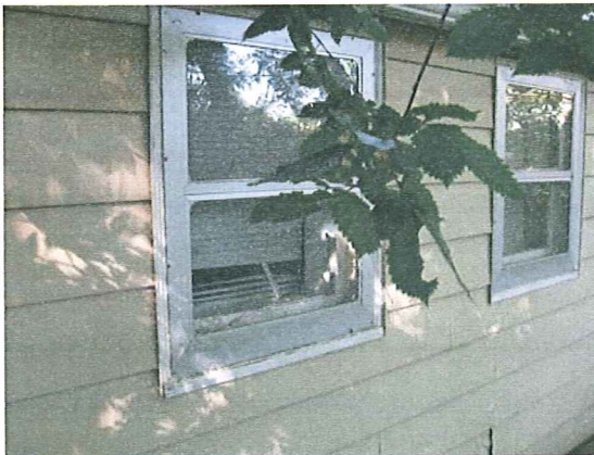
Broken/non-operable single pane window and storm
