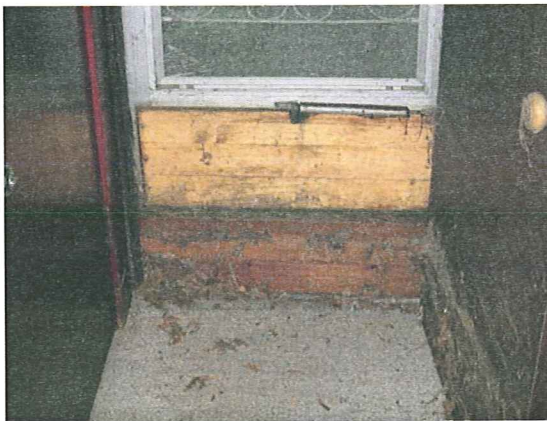
Floor elevation in home is 10" below outside grade
