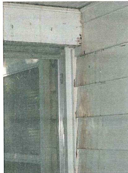
Water staining at back porch
