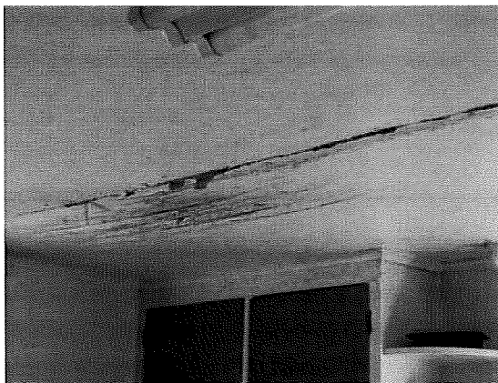
Water damage in kitchen ceiling
