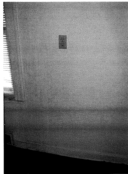
Water staining on wall around window
