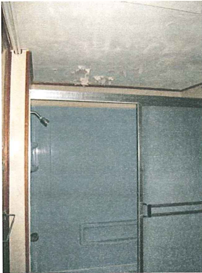
Peeling paint on bathroom ceiling
