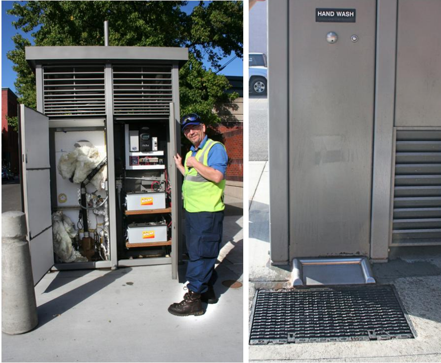
Picture of insulation around water pipe and of exterior hand wash area
