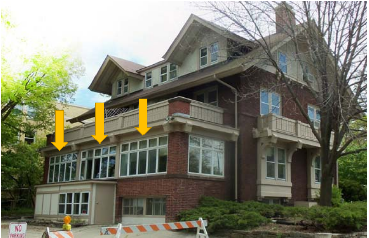
Back of house, replace 3 bays of main level porch windows, current mix of fixed and casement and fixed transom.
