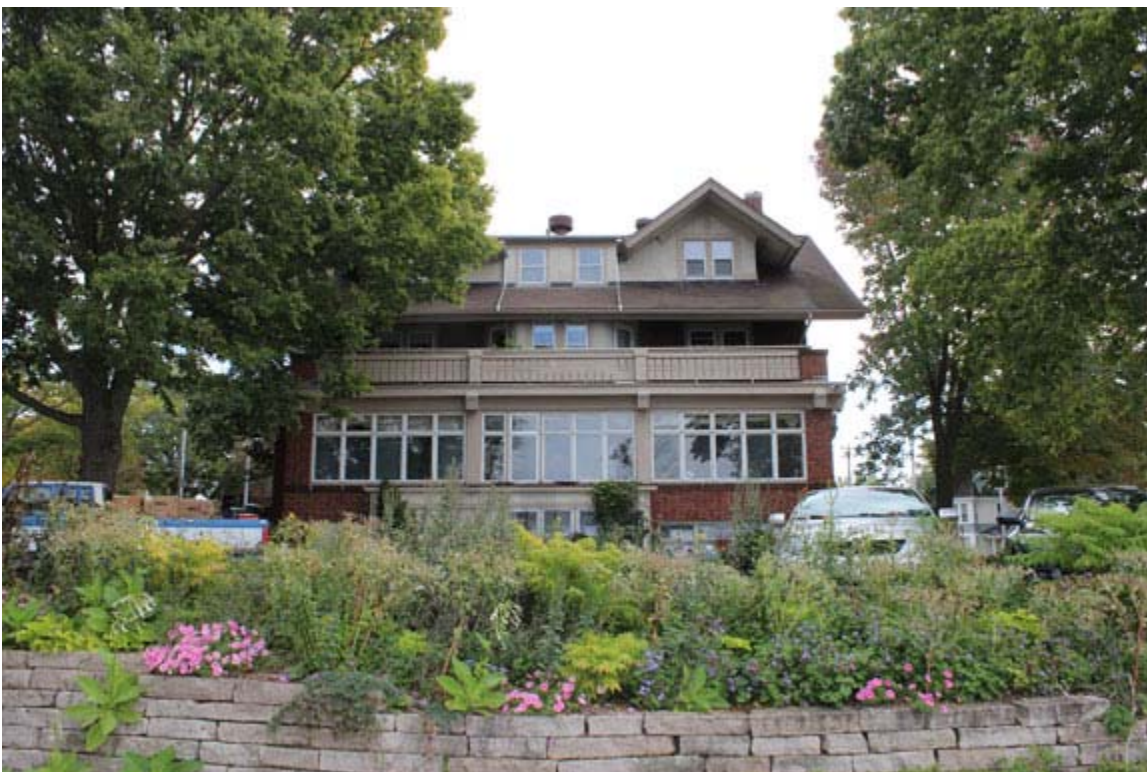
Back of house, top floor center dormer showing proposed configuration of 2 double hung.
