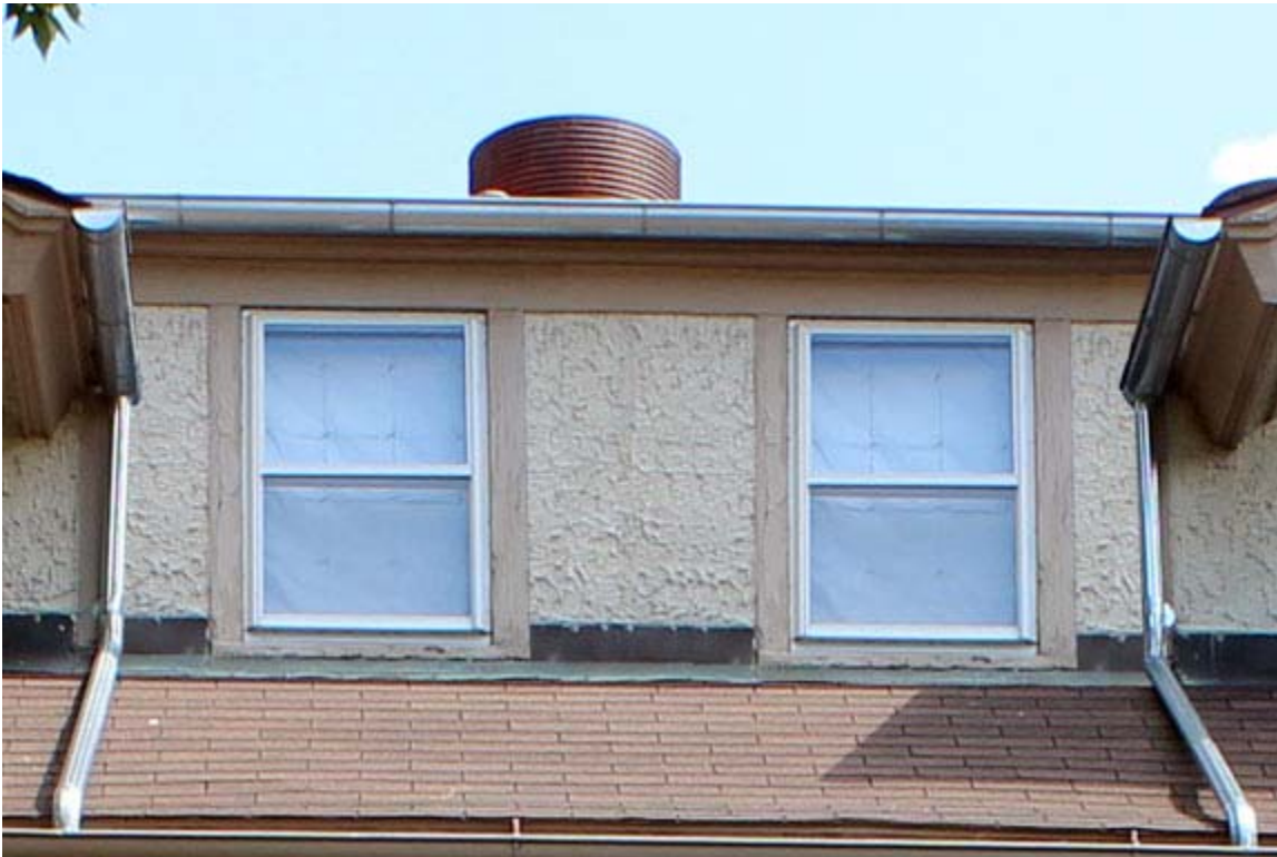
Proposed configuration using the existing windows as an example. Actual windows will be replaced with new Marvin double hung and be a few inches shorter to get
