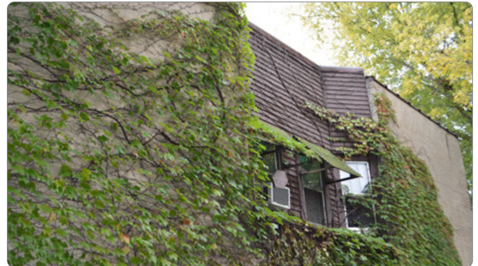
Figure 21: Growing vegetation that should be removed (41.23.3.d.2).
