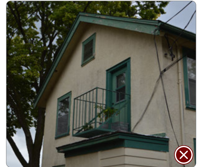
Figure 114: Incompatible balcony addition on the side of a building (41.26.6.b).
