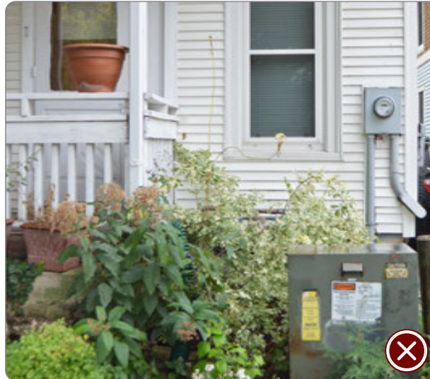
Figure 82: Utilities at the front of a building, in this placement, it should be screened with fencing or landscaping (41.25.7.a.2).
