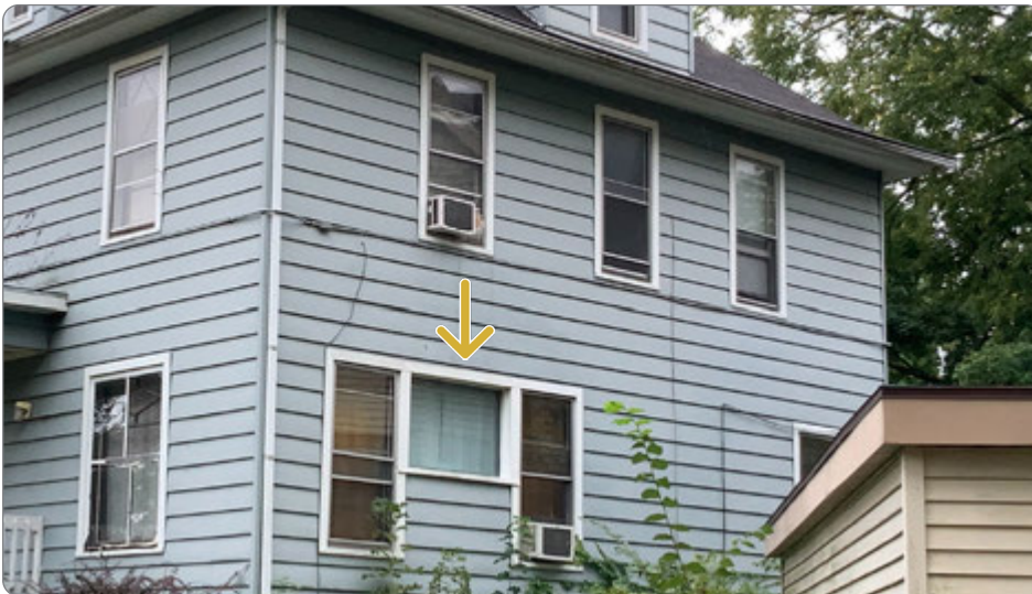
Figure 61: Incompatible window opening, visible from the right-of-way, not in keeping with existing visual qualities (41.25.5.a.1).
