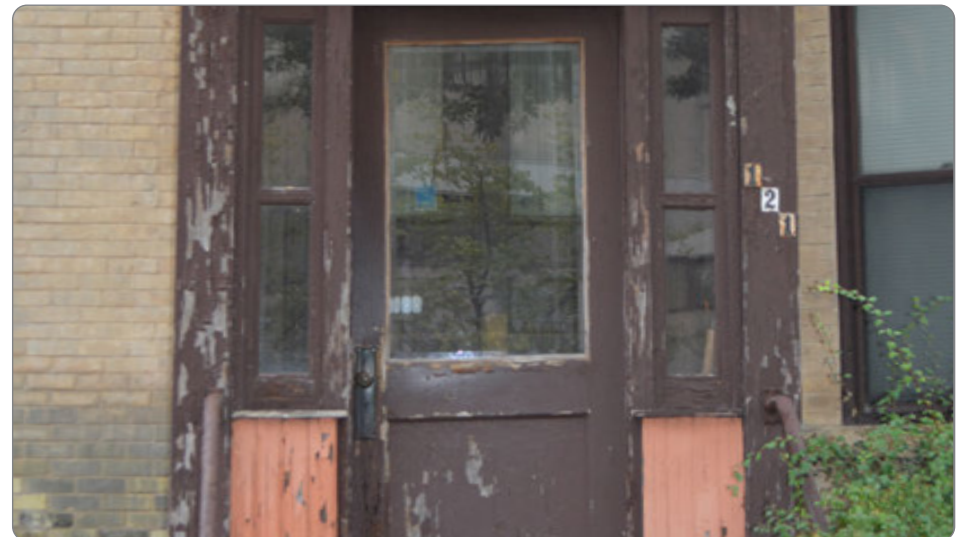
Figure 42: Example of windows and door in need of repair (41.24.5).
