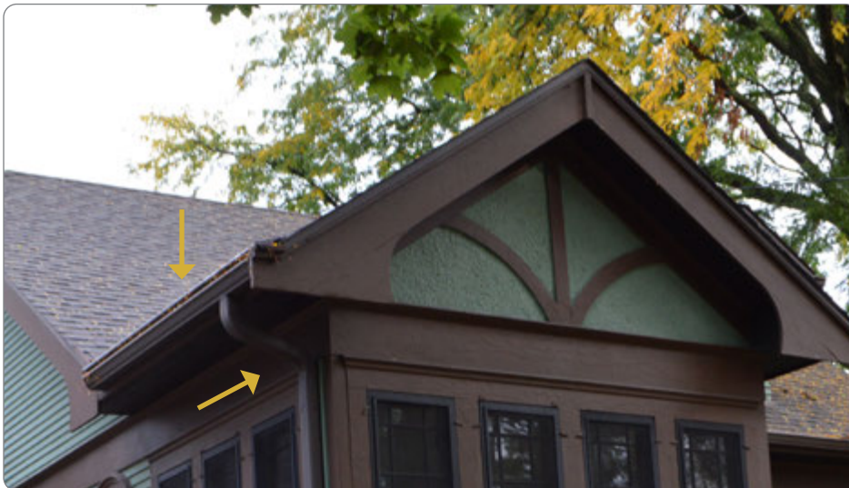
Figure 23: Example of a gutter guard protecting gutter system at 1520 Rutledge Street (41.23.4.a.1).
