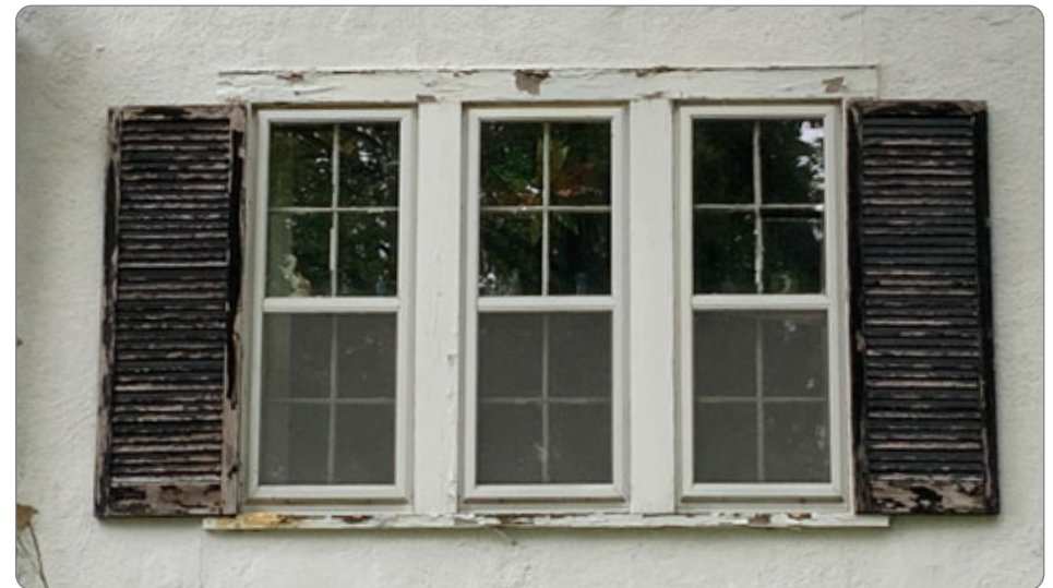
Figure 18: Example of wood shutters and window framing needing to be appropriately re-painted (41.23.3.b.1).
