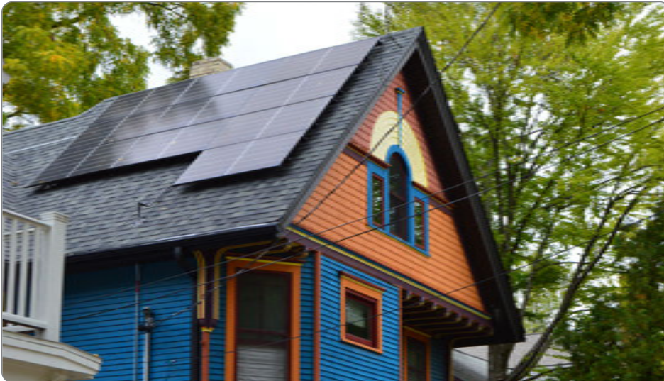
Figure 84: Example of solar panel roof installation (41.25. 7.b).
