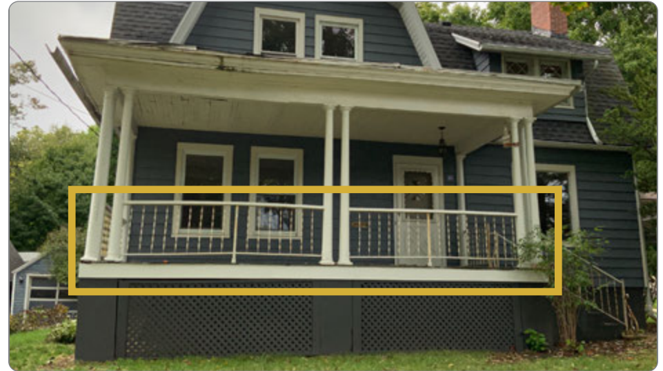
Figure 73: Example of a replacement railing that is out of character for the style house (41.25. 6.a.1).
