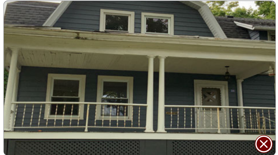
Figure 57: Incompatible substitute metal replacement (41.25.3.c.1).
