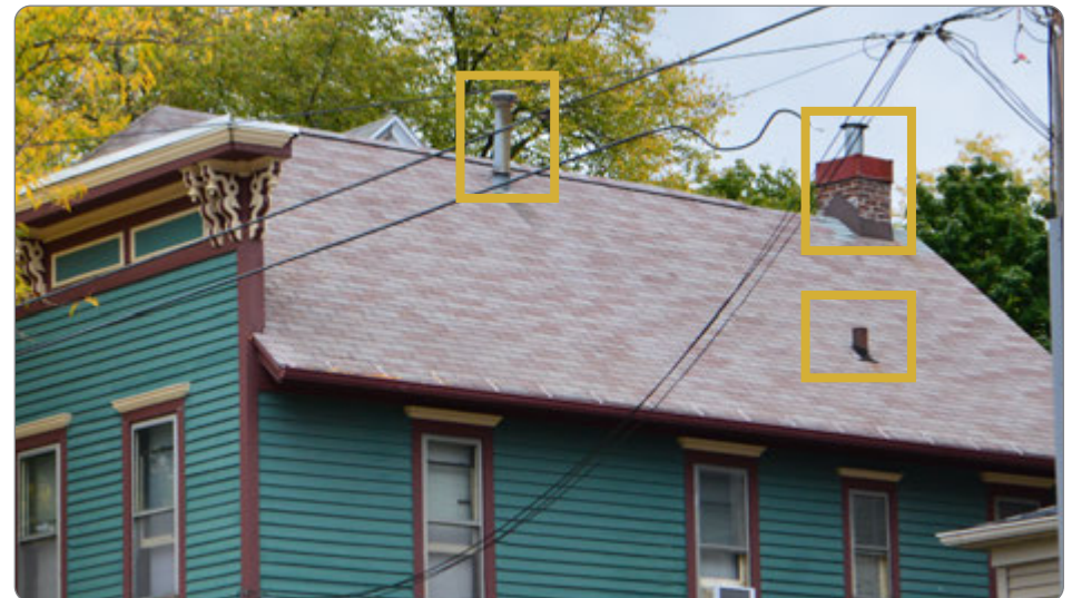
Figure 60: Example of ridge vent and a prohibited electric vent visible from the developed public right-of-way (41.25.4.e).
