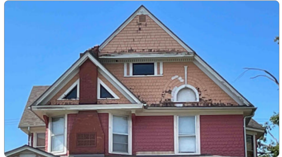
Figure 17: Example of wood siding needing to be re-painted on a residence that is otherwise in good condition (41.23.3.b.1).
