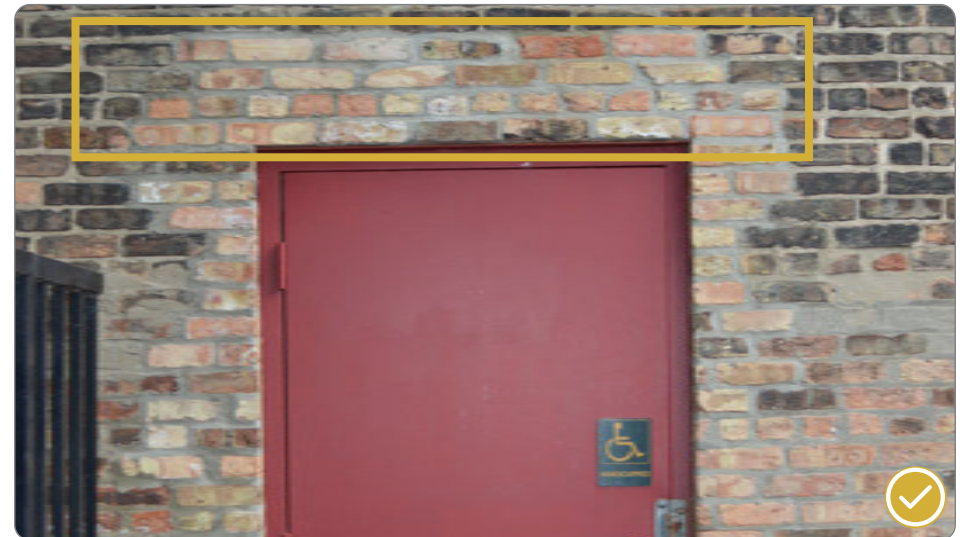
Figure 53: Brick masonry units installed around new accessibility door; the new bricks are currently cleaner than the original (41.25.3.a.3).
