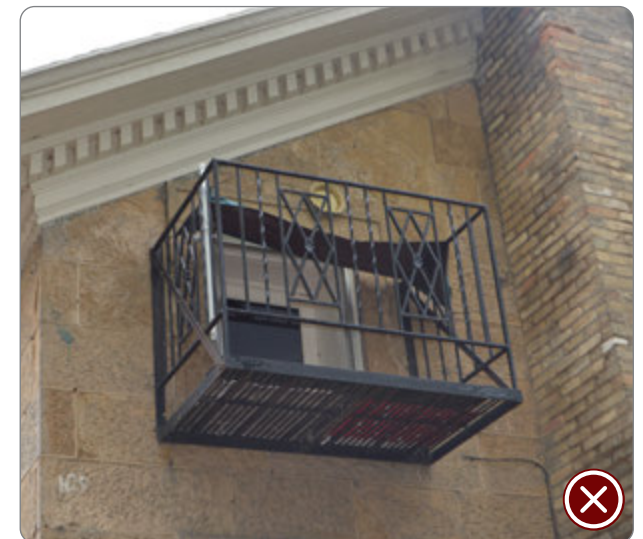
Figure 115: Incompatible balcony addition on front elevation (41.26.6.b).
