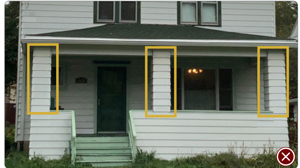
Figure 54: Incompatible wrapped wood columns (41.25.3.b.4).
