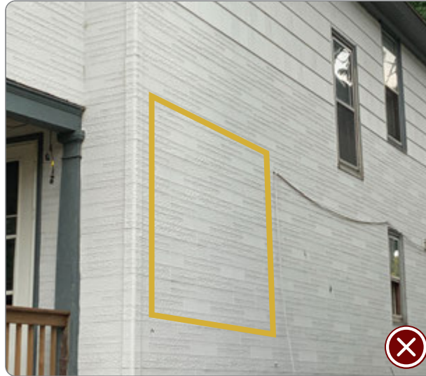
Figure 45: Incompatible replacement of historic siding (41.25.1.b.1).
