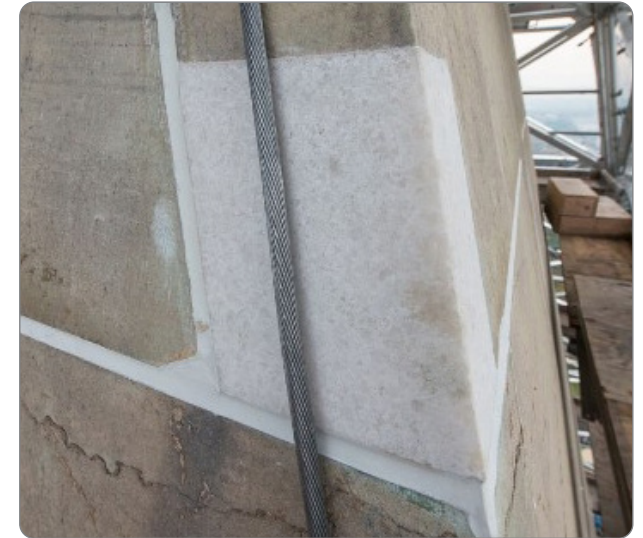
Figure 34: Example of a dutchman repair.
