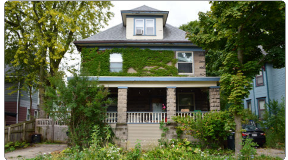
Figure 20: Vegetation on a masonry building can damage the masonry and mortar (41.23.3.d.2).
