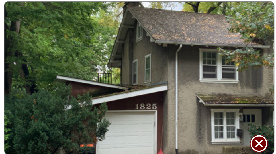
Figure 95: Incompatible side addition on a residential building (41.26.3.a.1).
