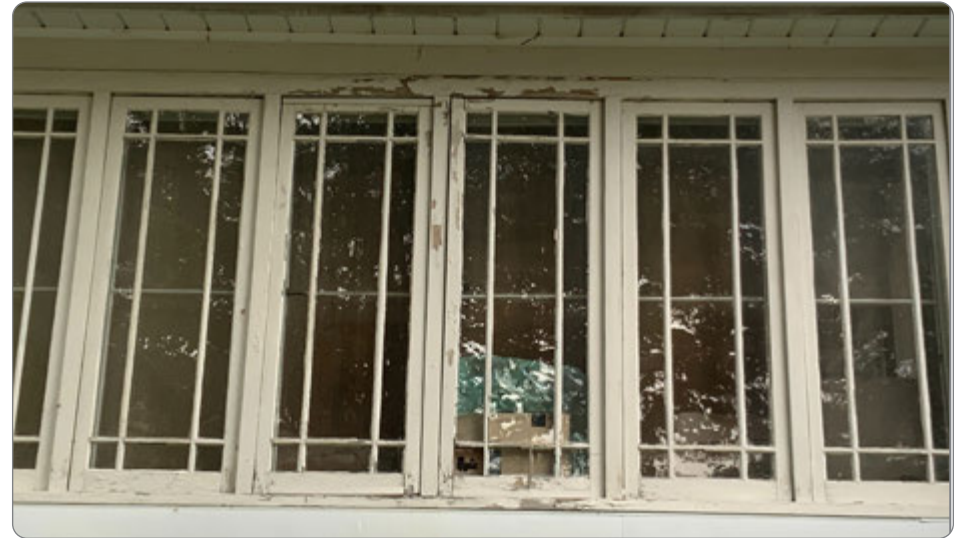
Figure 41: Example of windows in need of repair (41.24.5).
