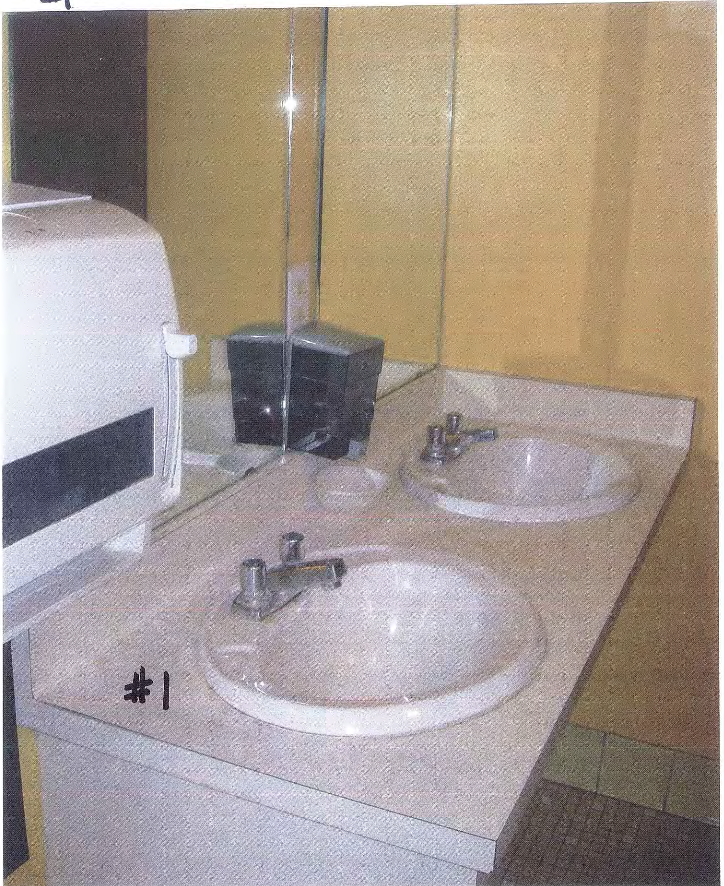
PHOTO # 21 MAIN TOILET. WOMEN #1 OUTDATED & NON-FUNCTIONING FIXTURES.
