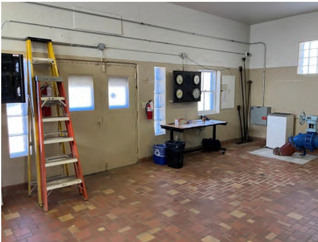
Interior of existing Wellhouse.
