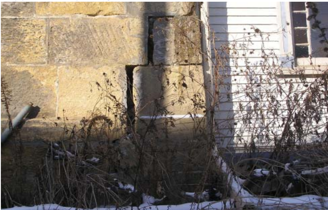
CRACKED WALL FOUNDATION
