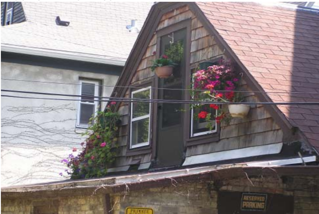
SLANTED PORCH FLOOR WITH NO RAILINGS
