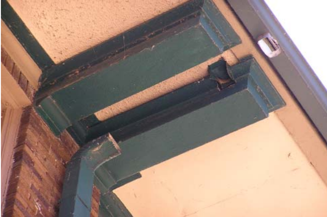
MISSING PART OF DOWN SPOUT
