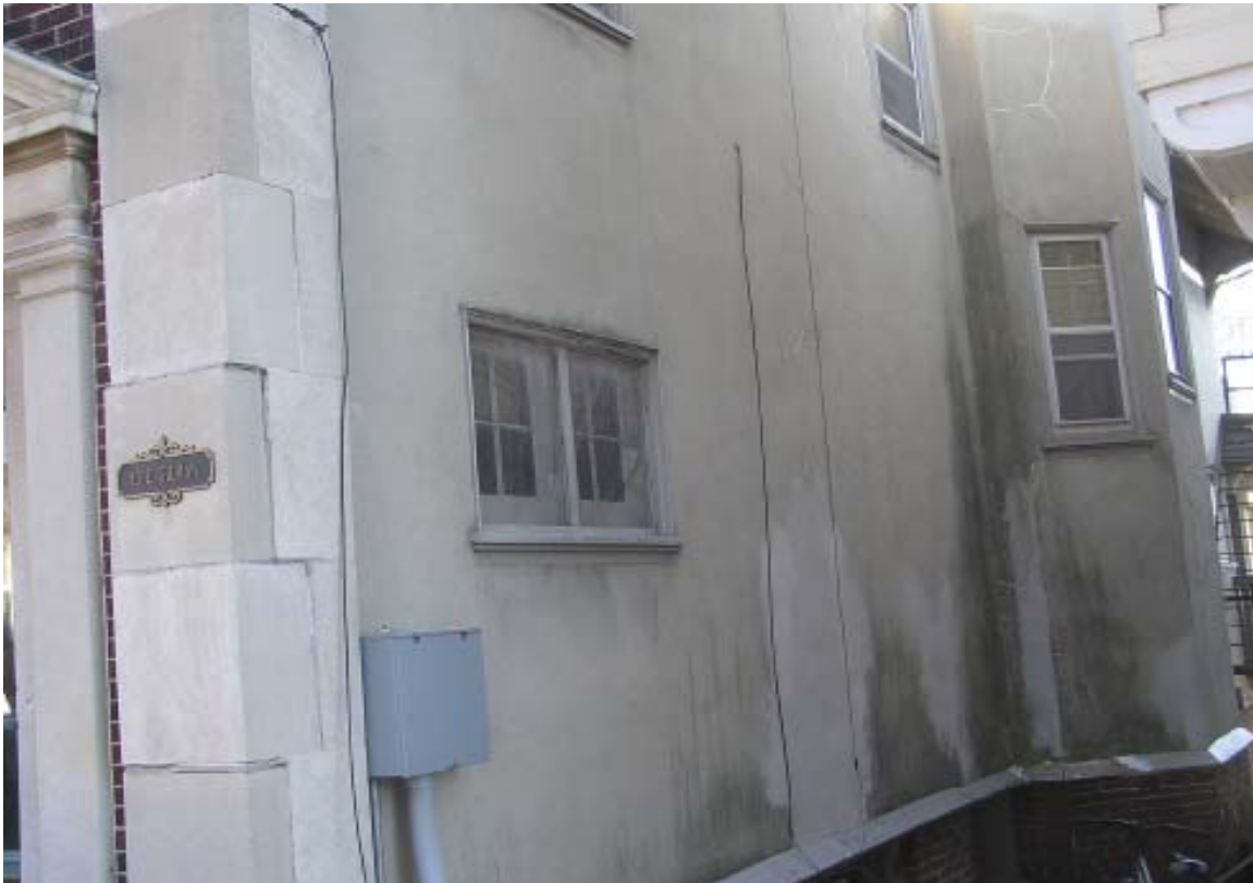
WALL CRACKS, WATER DAMAGED AND BLOCKS OFF SET
