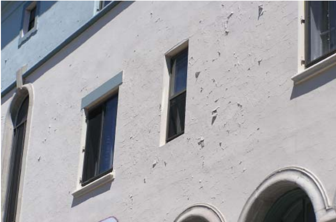
DETERIORATING STUCCO (2of2)
