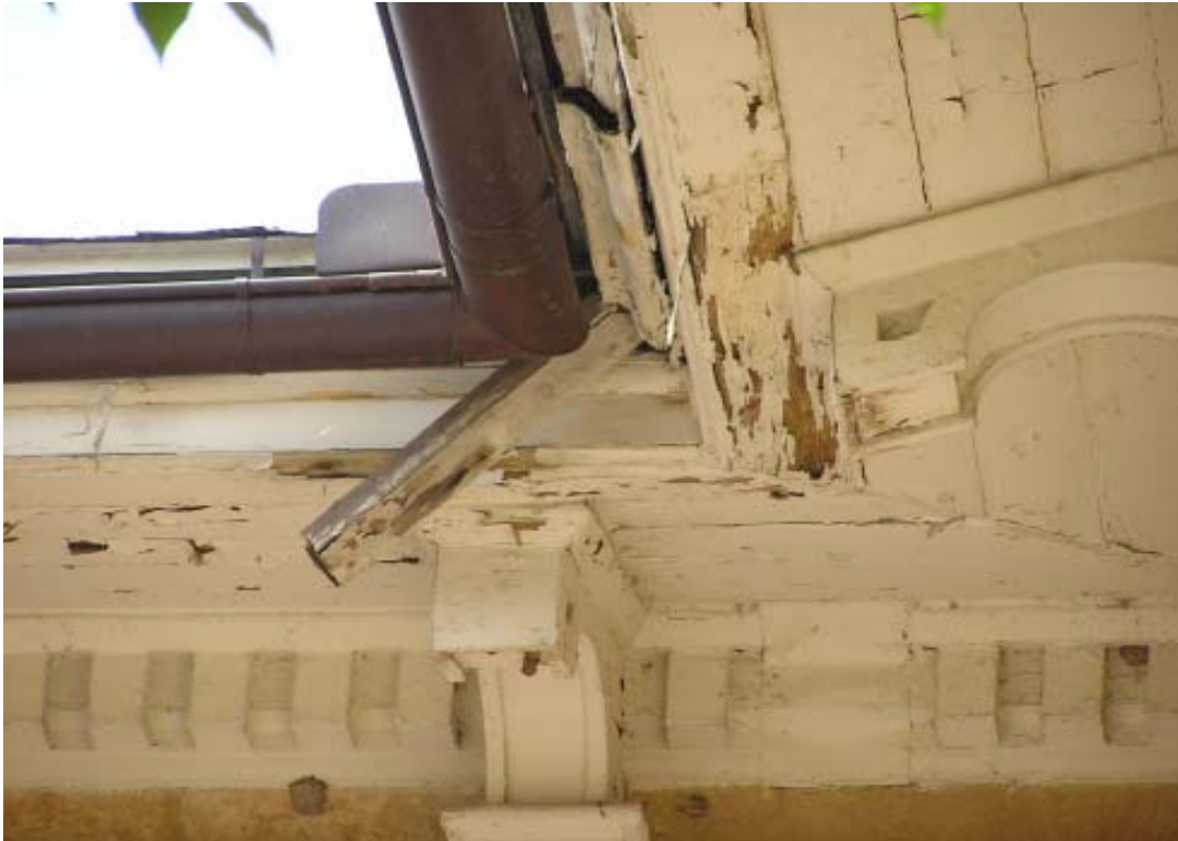
DETERIORATED FASCIA & SOFFIT
