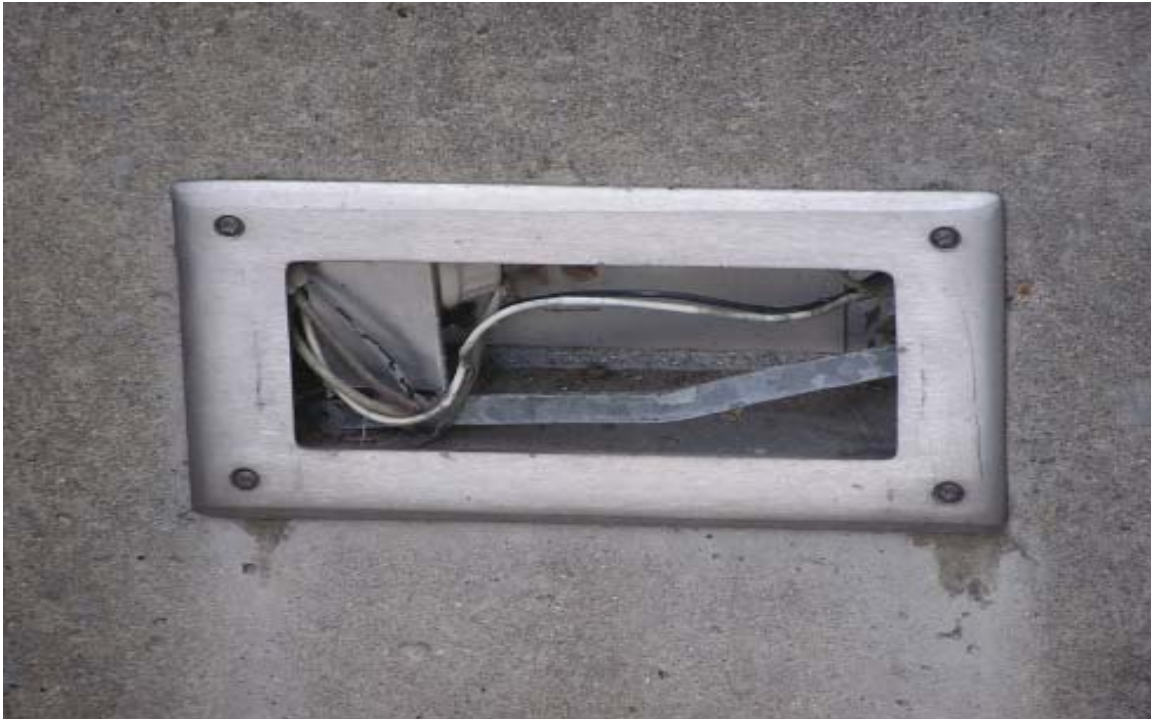
LIGHT BOX WITH EXPOSED WIRES
