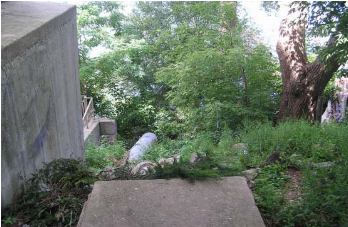
OPEN ENDED SIDEWALK LEADING TO A DANGEROUS DROP OFF
