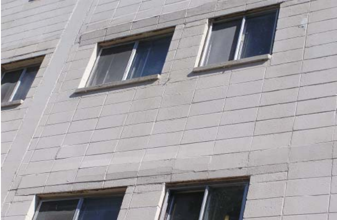
CONCRETE WALL BLOCKS BLUDGING =====
