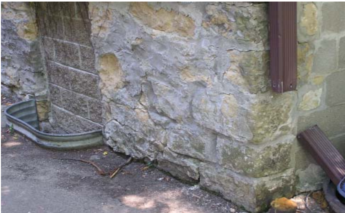
FOUNDATION WITH DETERIORATED STONE AND BROKEN PARGET, WINDOW BLOCKED UP AND DISCONNECTED DOWN SPOUT
