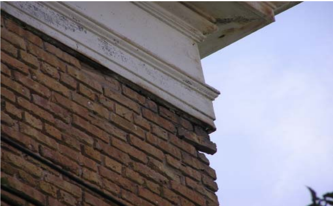
LOOSE BRICKS & WATER DAMAGED FASCIA AND SOFFIT
