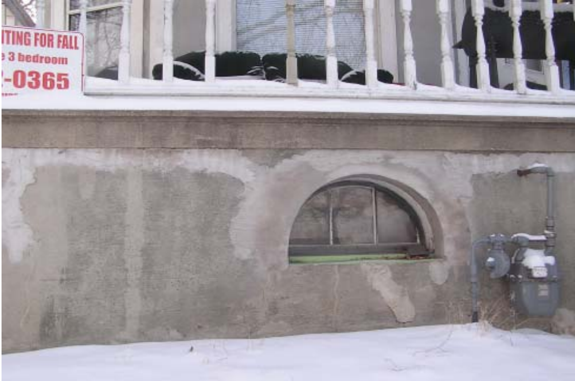
CRACKED PORCH WALL, DETERIORATED WINDOW FRAMES AND RUNG MISSING FROM RAILING
