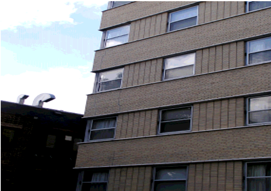
WALL CRACKS ON MULTIPLE LEVELS (1of2)
