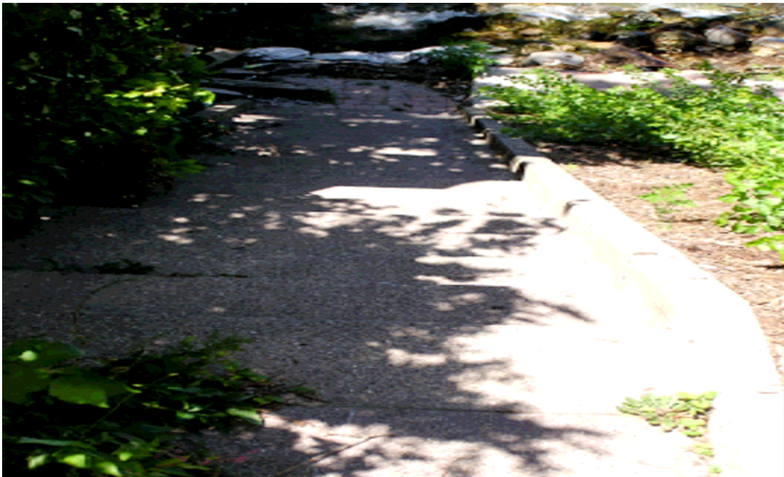
MULTIPLE STEPS WITHOUT RAILING, BROKEN SIDEWALK, WEEDS AND GRAVEL IN SIDEWALK
