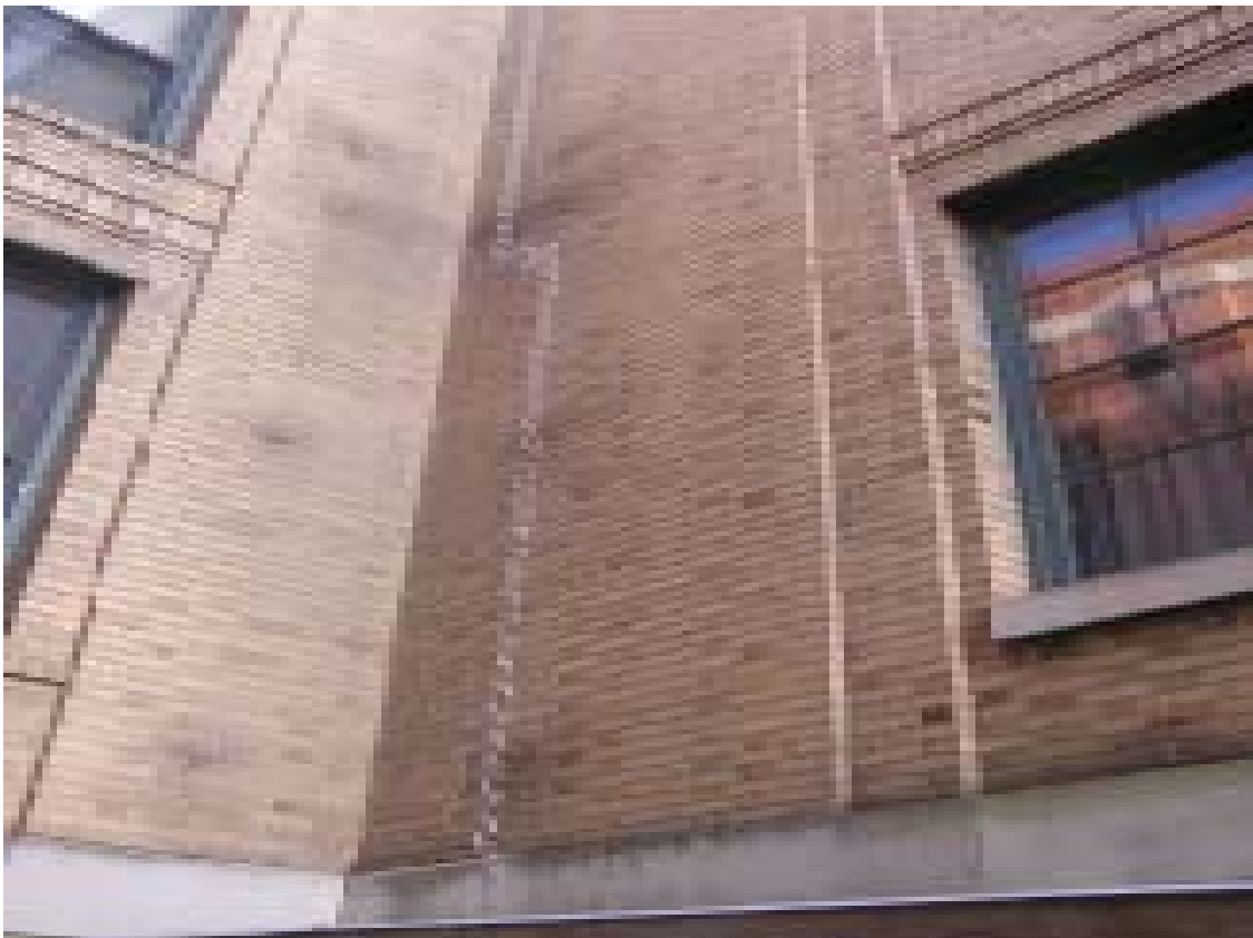
WALL CRACKS (2of2)
