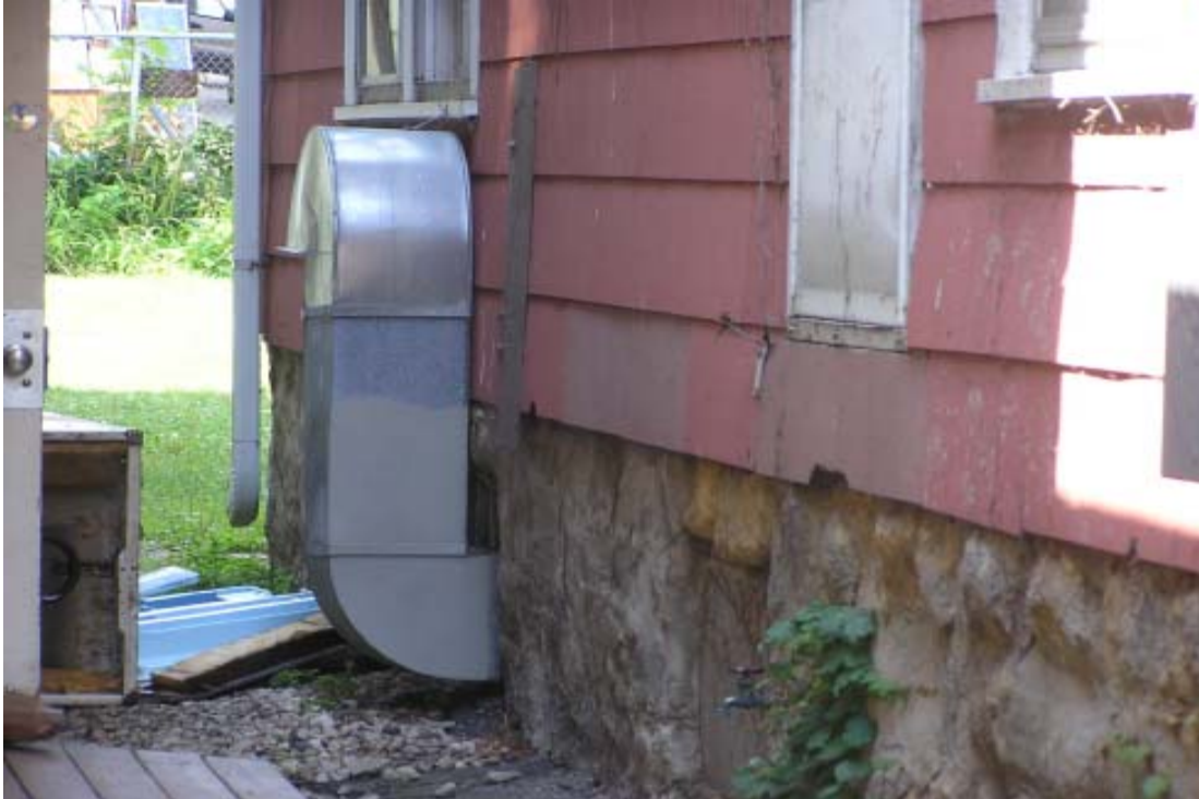
EXIT DOOR WITH NO STEPS, DETERIORATED STONE FOUNDATION, DETERIORATED WINDOW FRAMES, CHIPPED SIDING, & BOARDED UP WINDOWS
