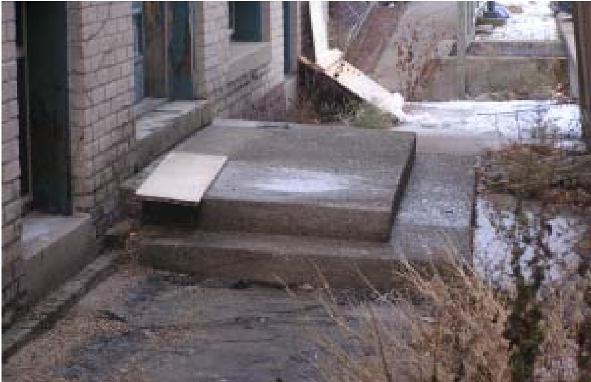
SLANTED PORCH, 3 STEPS WITH NO RAILING AND WATER DAMAGED BRICK
