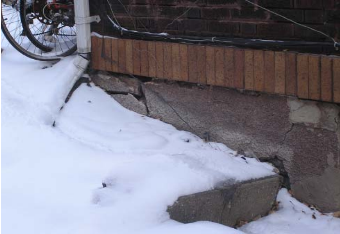
BROKEN, CRACKED FOUNDATION AND DISCONNECTED DOWN SPOUT
