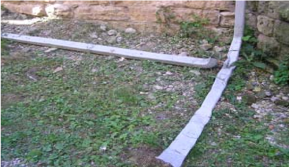
DETERIORATED FOUNDATION, DOWN SPOUT LYING ON THE GROUND AND SMASHED DOWN SPOUT LEAD
