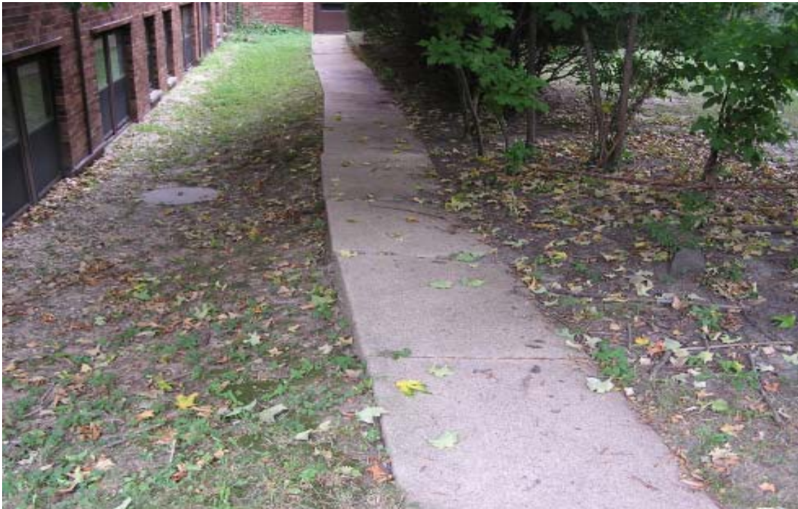
UNEVEN SIDEWALK WITH DROP OFF ON ONE SIDE
