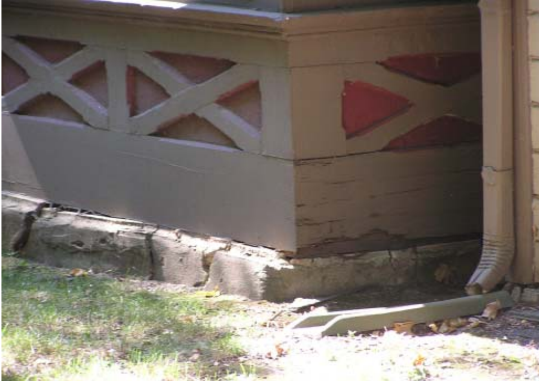
CRACKED BROKEN FOUNDATION AND DETERIORATED CLAP BOARD
