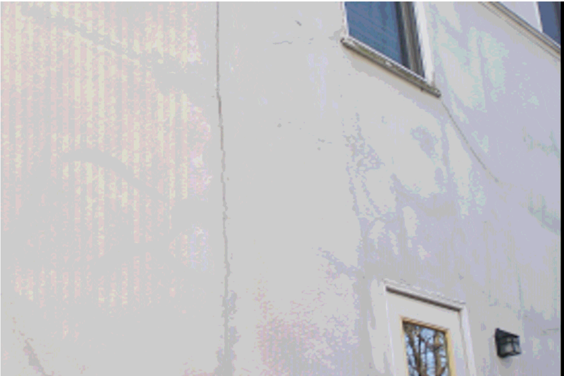
WALL CRACKS, DETERIORATED WINDOW SILL
