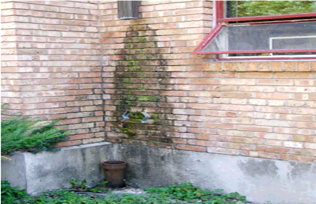
DOWNSPOUT MISSING CAUSING DAMAGE (2of2)
