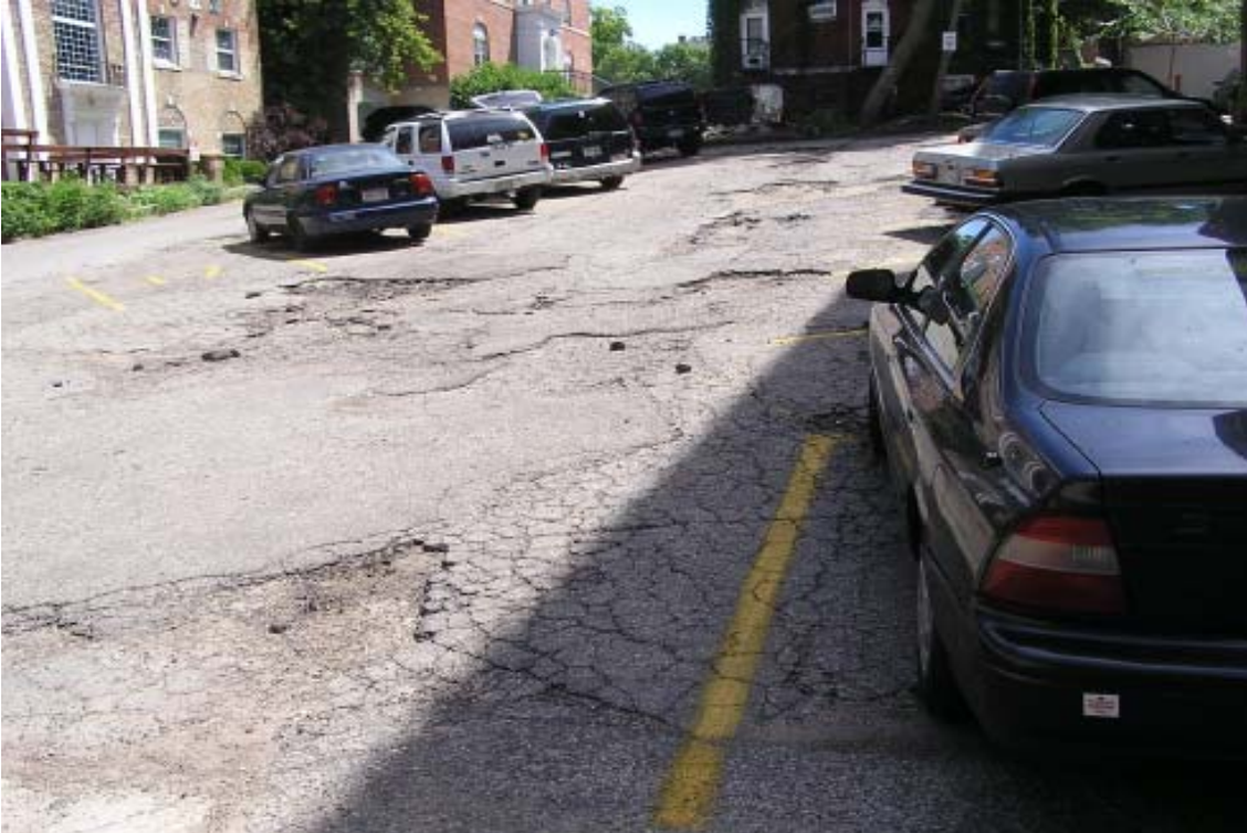
BLIGHTED PARKING LOT WITH PAVEMENT IN POOR CONDITION
