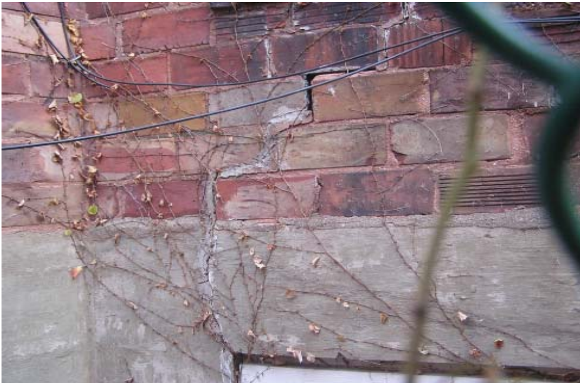
CRACKED FOUNDATION / CRACKED WALL
