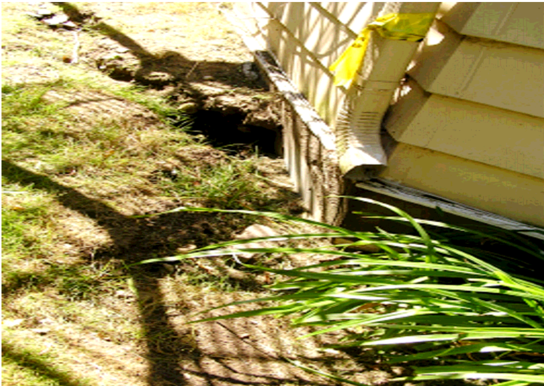
YARD EROSION, FOUNDATION DETERIORATED FROM DOWN SPOUT WATER FLOW
