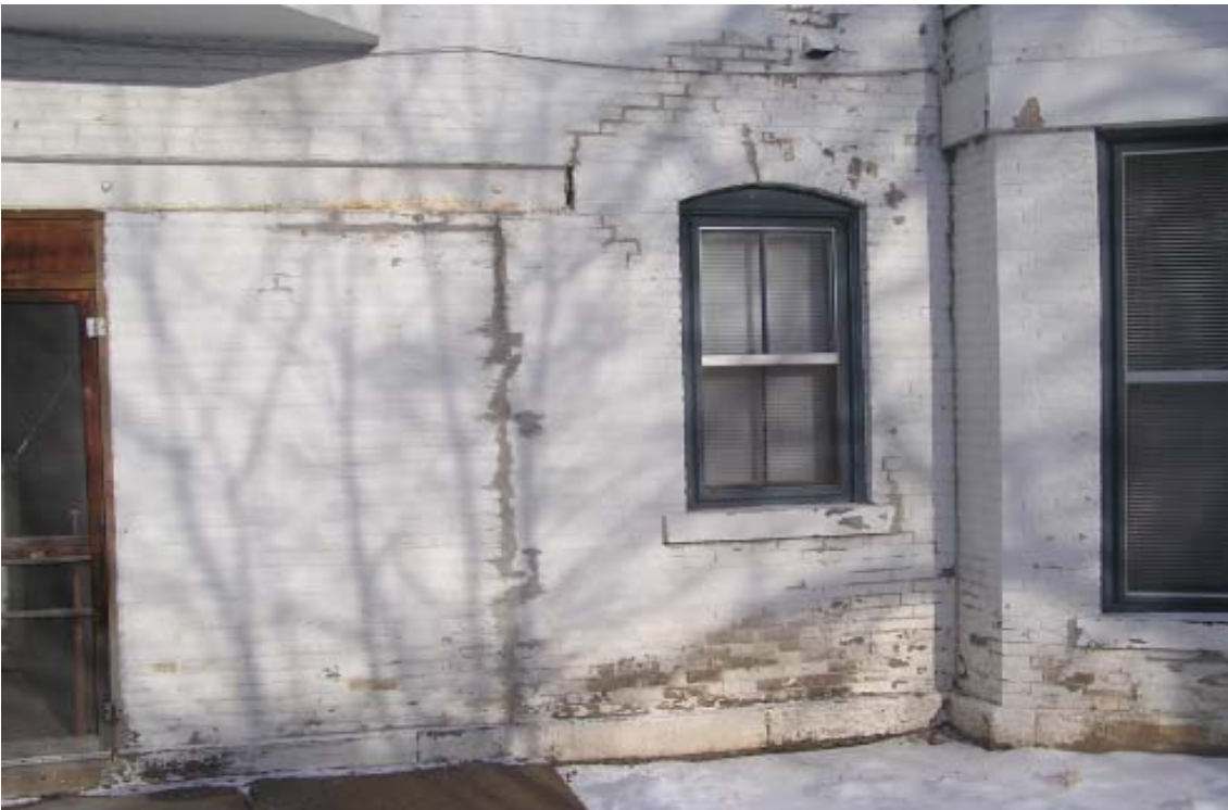
MORE WALL CRACKS AND WINDOW FRAMES DETERIORATED (2of2)
