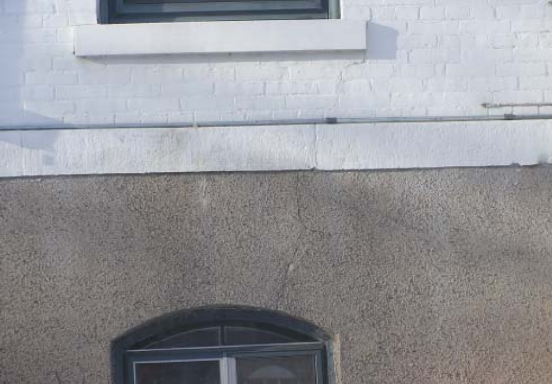
WALL AND FOUNDATION CRACKS (1of2)
