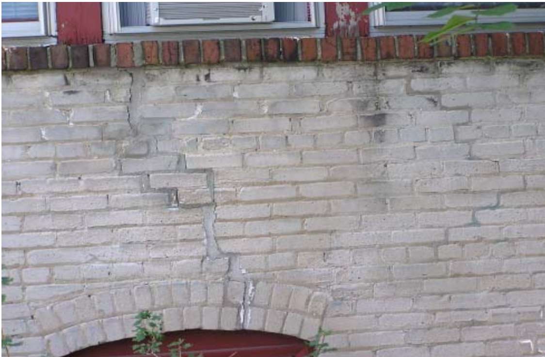
WALL CRACKS AND DETERIORATED WINDOW FRAME
