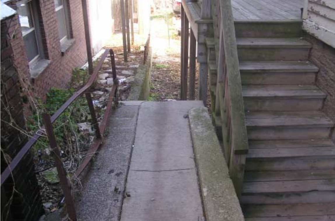
DANGEROUS DROP OFF OF SIDEWALK, BROKEN AND RUSTED RAILING AND DETERIORATED STEPS
