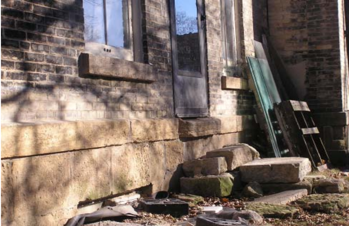
DOORWAY WITHOUT ADEQUATE PORCH OR STEPS, DETERIORATED WINDOW FRAMES
