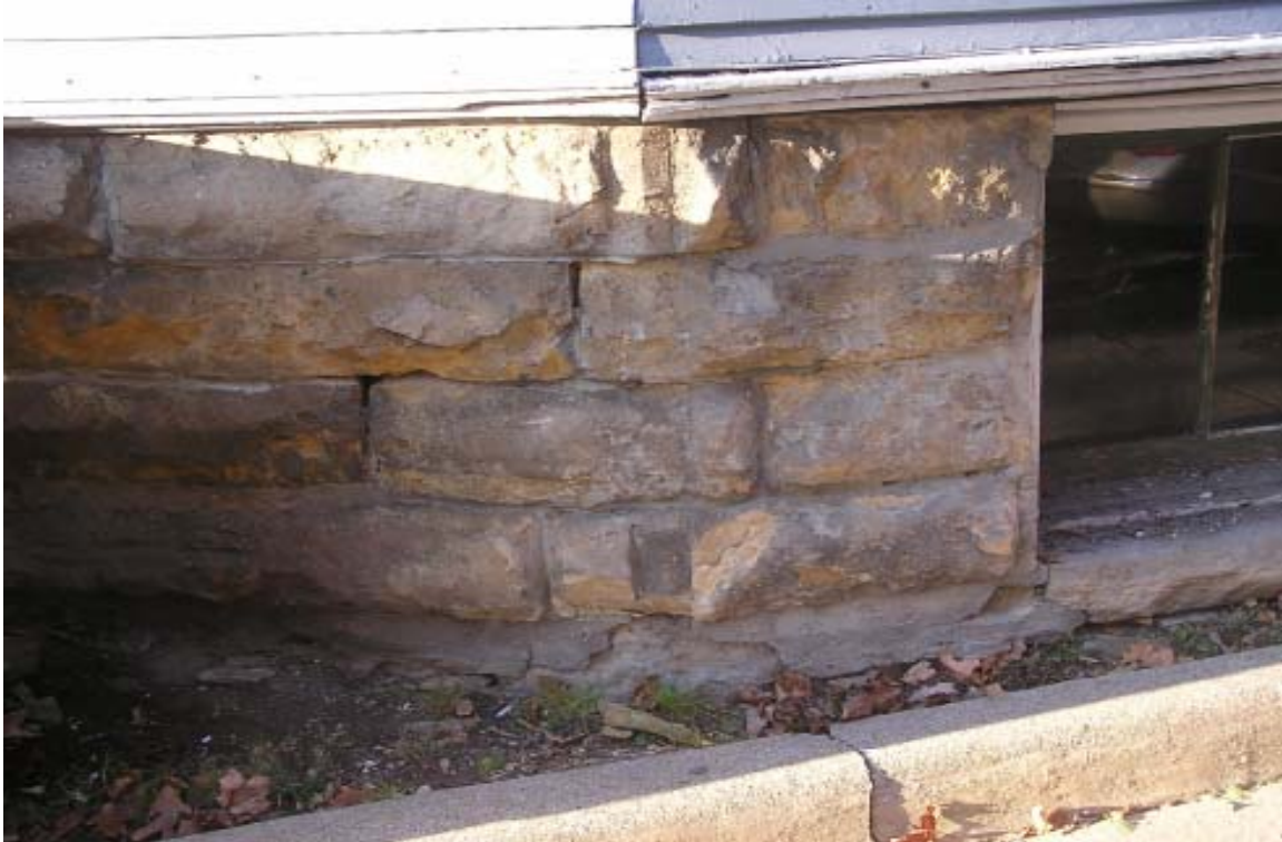
ROTTEN TRIM, DETERIORATED CRACKED STONE WITH CHIPS OF STONE ON THE GROUND
