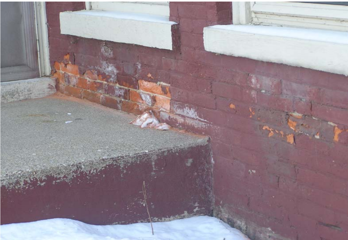
WALL CRACKS AND DETERIORATED BRICK LYING ON PORCH
