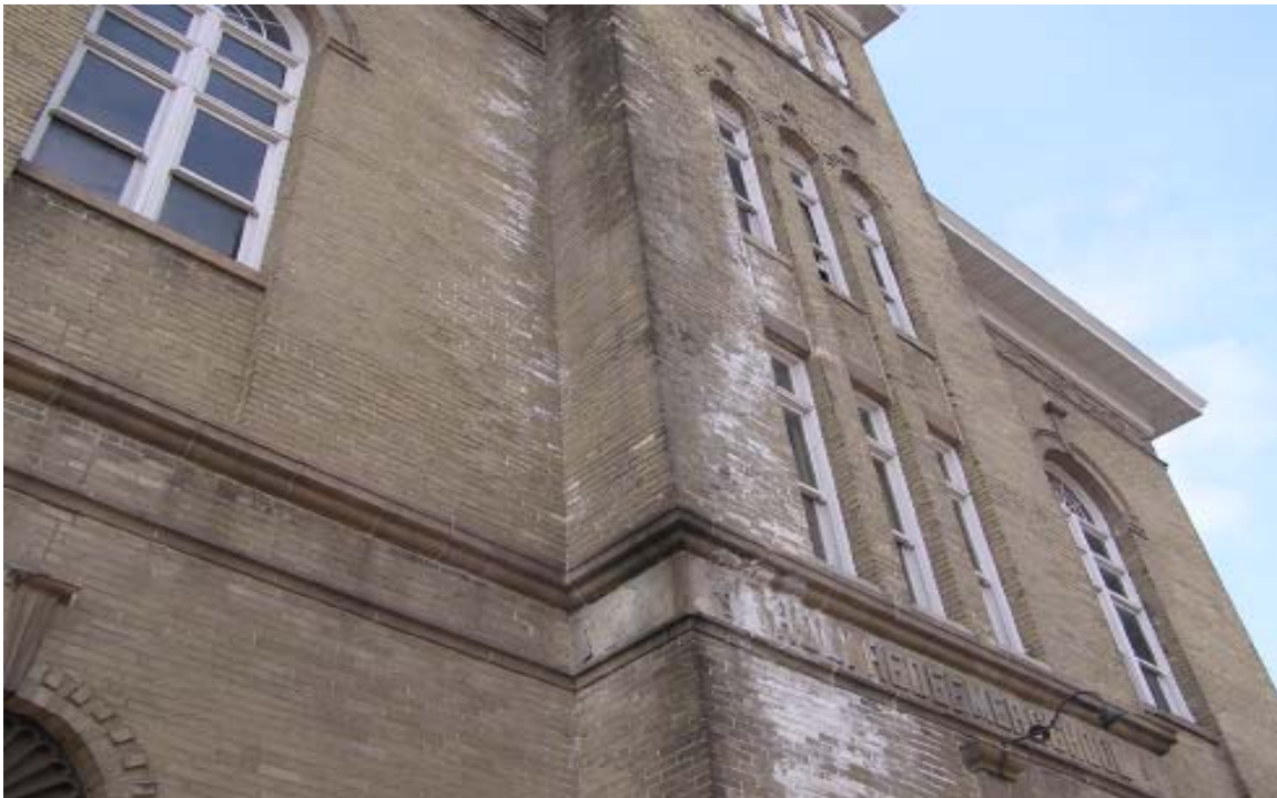
WATER DAMAGED BRICKS
