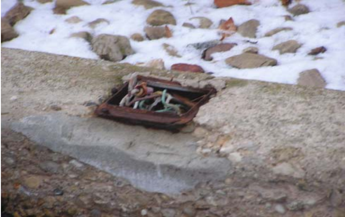
EXPOSED ELECTRIC WIRES IN THE PARKING LOT
