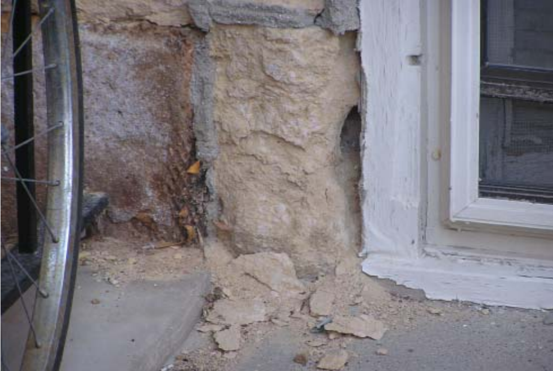
DETERIORATED FOUNDATION STONE WITH CHIPS AND DUST ON THE SIDEWALK
