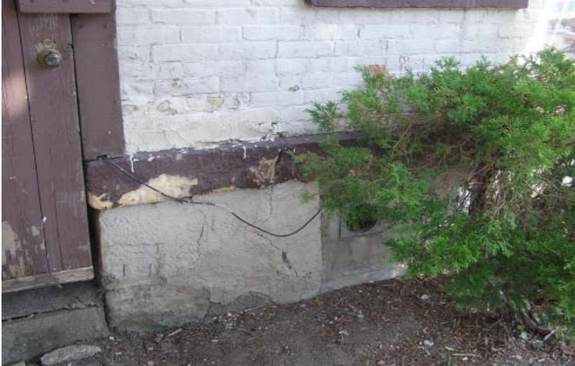
BLOCKED UP WINDOW, CRACKED PARGET, SILL, AND WALL, DETERIORATED BRICK, DOOR AND DOOR FRAME
