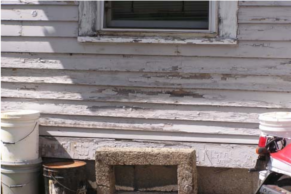
DETERIORATED CLAP BOARD AND WINDOW FRAME, STORED RUSTING PAILS OUTSIDE
