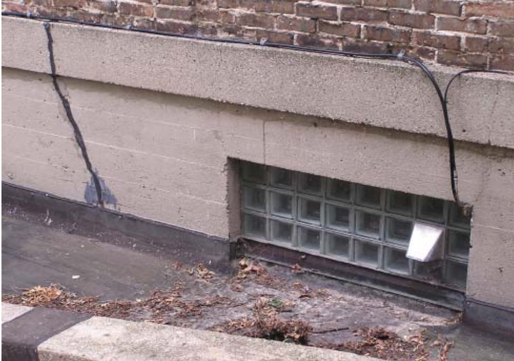
CRACKED FOUNDATION AND BLOCKED UP WINDOWS
