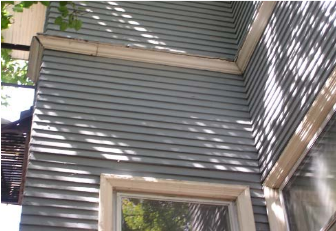
DETERIORATED WALL TRIM, WINDOW FRAME AND CLAP BOARD (2of2)
