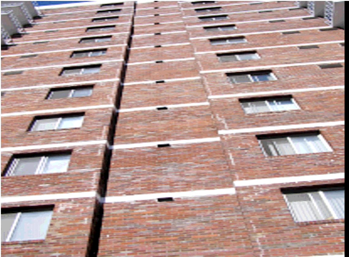
MANY CRACKS ON MULTI FLOOR BUILDING
