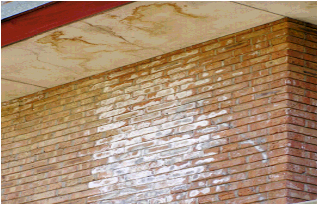
WATER DAMAGE TO WALL AND SOFFIT (1of 2)
