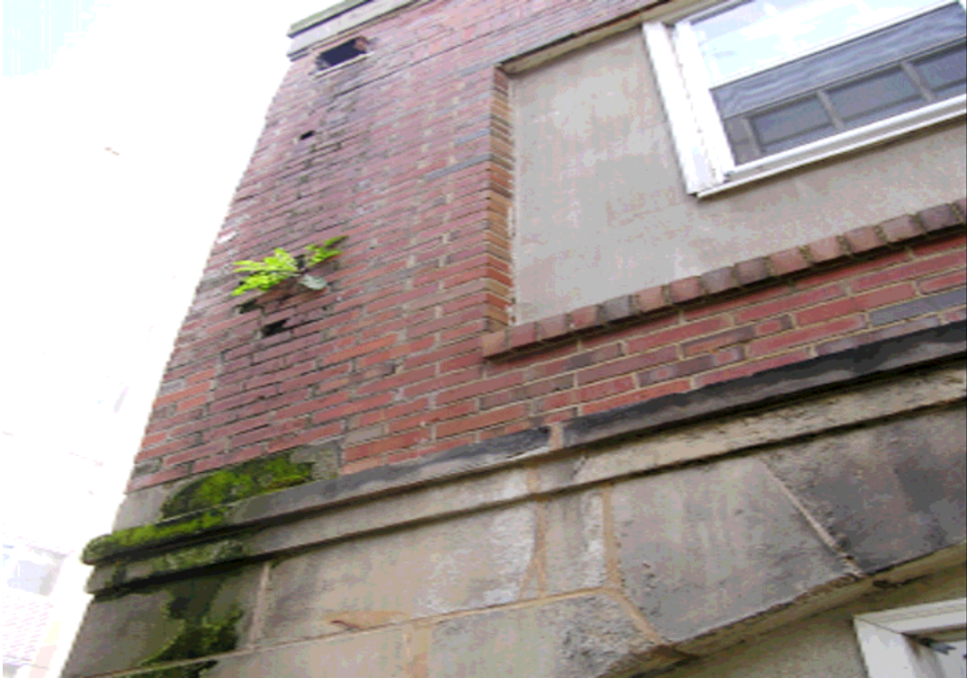
WATER DAMAGE TO BRICK WALL WITH DANDILION GROWING ON THE WALL
