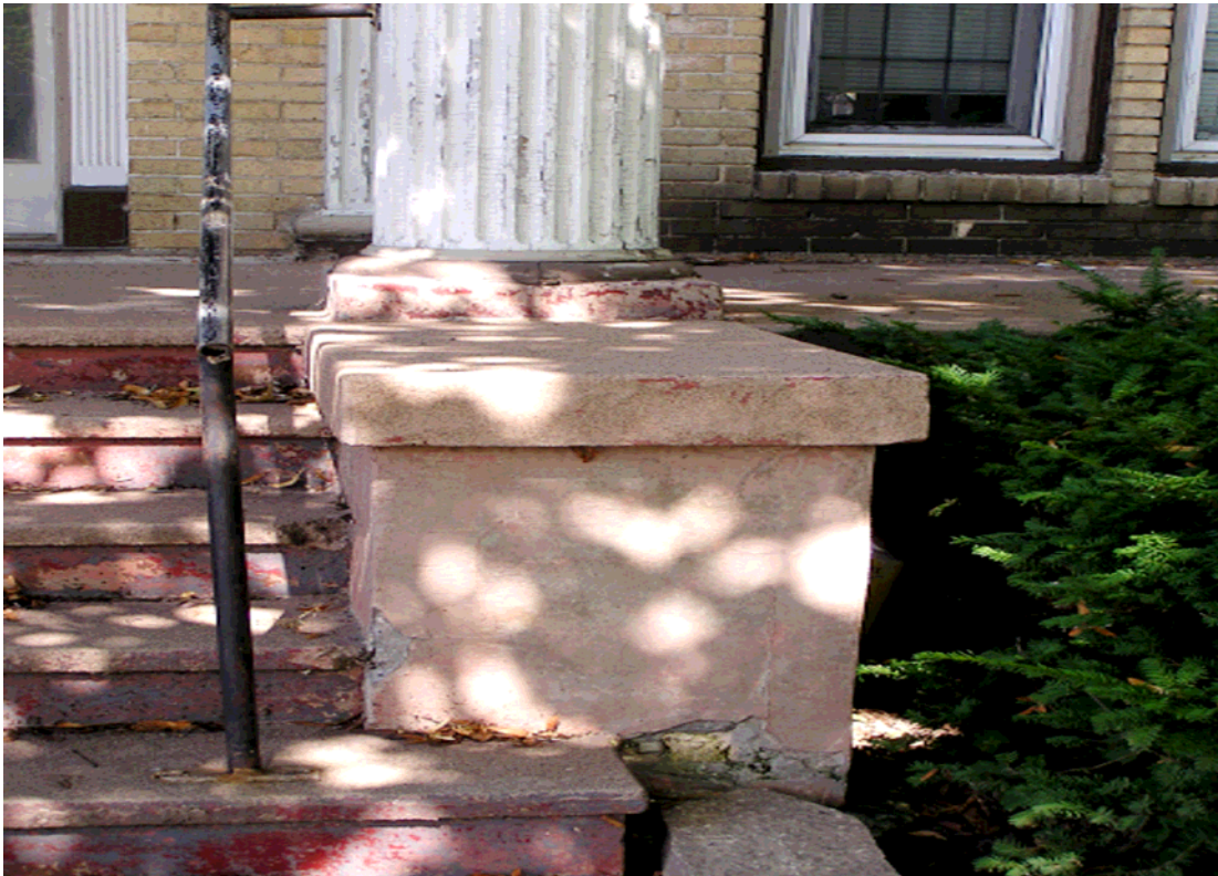
CEMENT AND WOOD POSTS DETERIORATED
