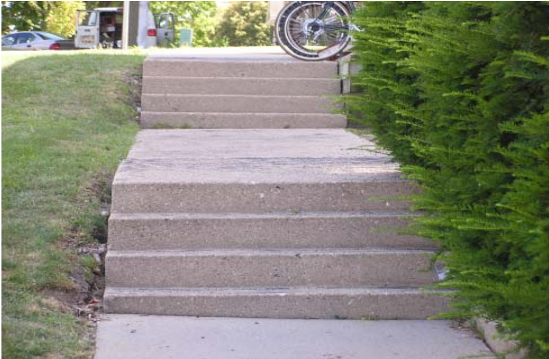
MULTIPLE STEPS WITH NO RAILING (2of2)
