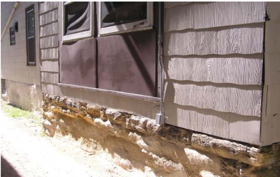
DETERIORATED FOUNDATION STONE AND WINDOW FRAME BOARDED UP WINDOW
