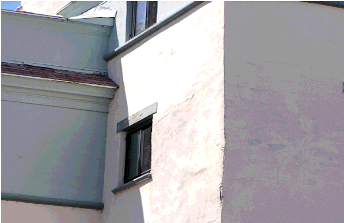
DETERIORATING STUCCO (1of2)
