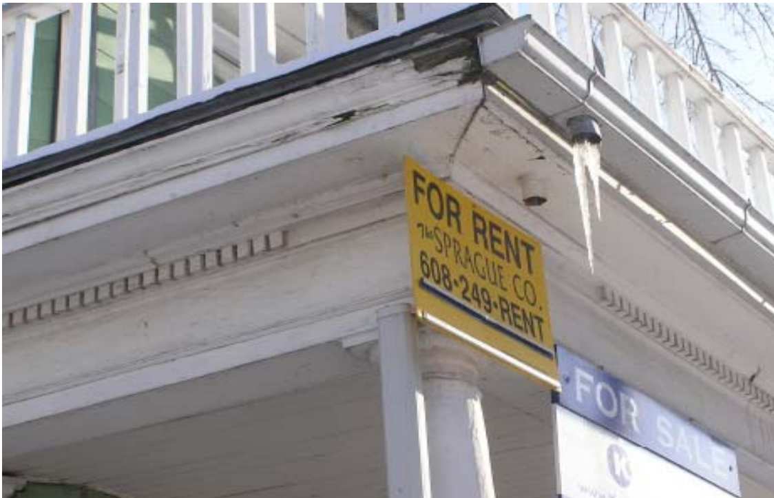
DOWN SPOUT NOT CONNECTED, DETERIORATED PORCH ROOF /FLOOR AND POST
