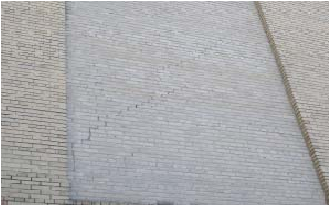
WALL CRACKS (1of2)
