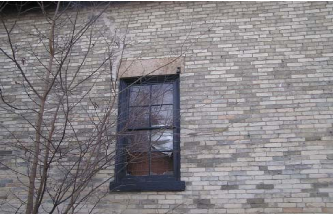
CRACKED WALL, BROKEN WINDOW AND DETERIORATED WINDOW FRAME
