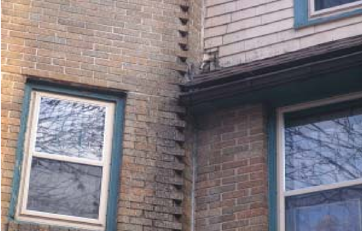
DETERIORATED WOOD, WINDOW FRAMES AND WATER DAMAGED BRICKS
