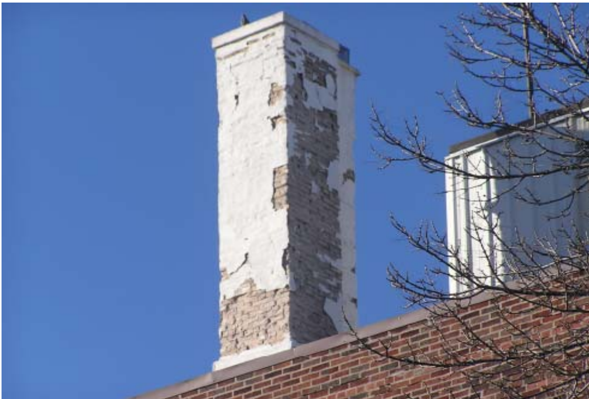
CHIMNEY BRICK DETERIORATED, CRACKED AND MISSING MORTAR
