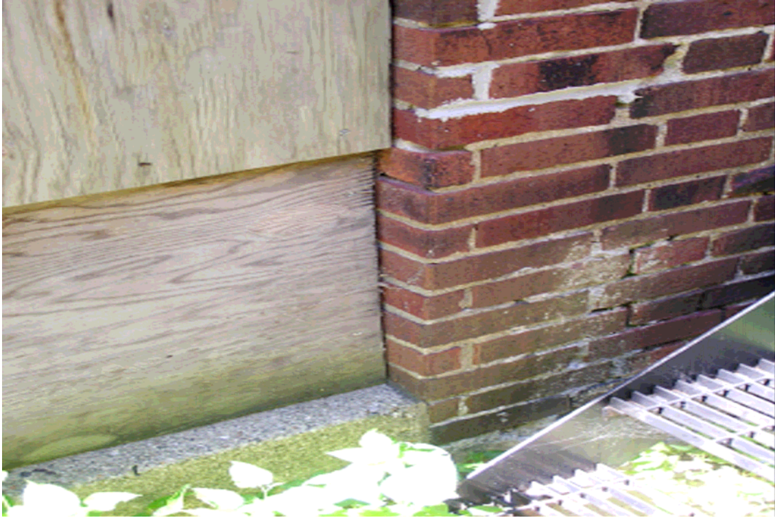
BOARDED UP WINDOW AND MORTAR MISSING IN BRICK FOUNDATION =====
