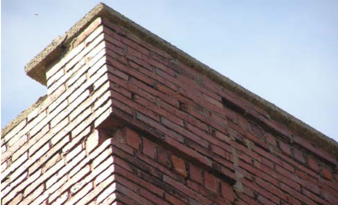
CORNER CORNICE PROTRUDING AND BROKEN BRICKS
