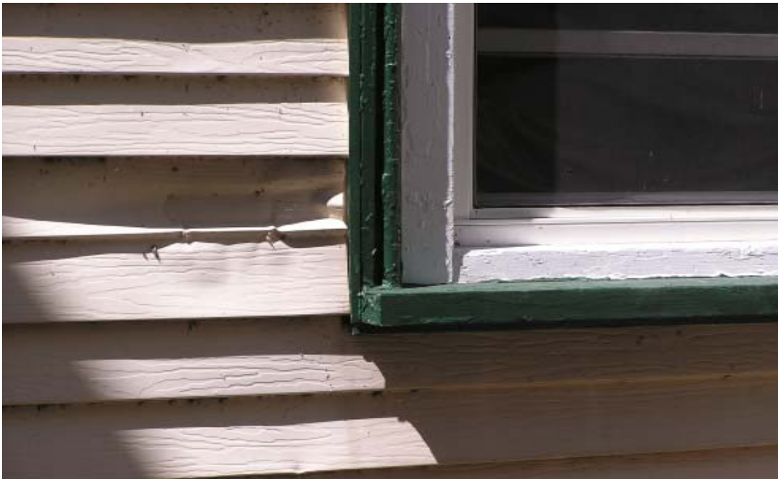
DETERIORATING WINDOW FRAME & DENTED SIDING (1of 2)
