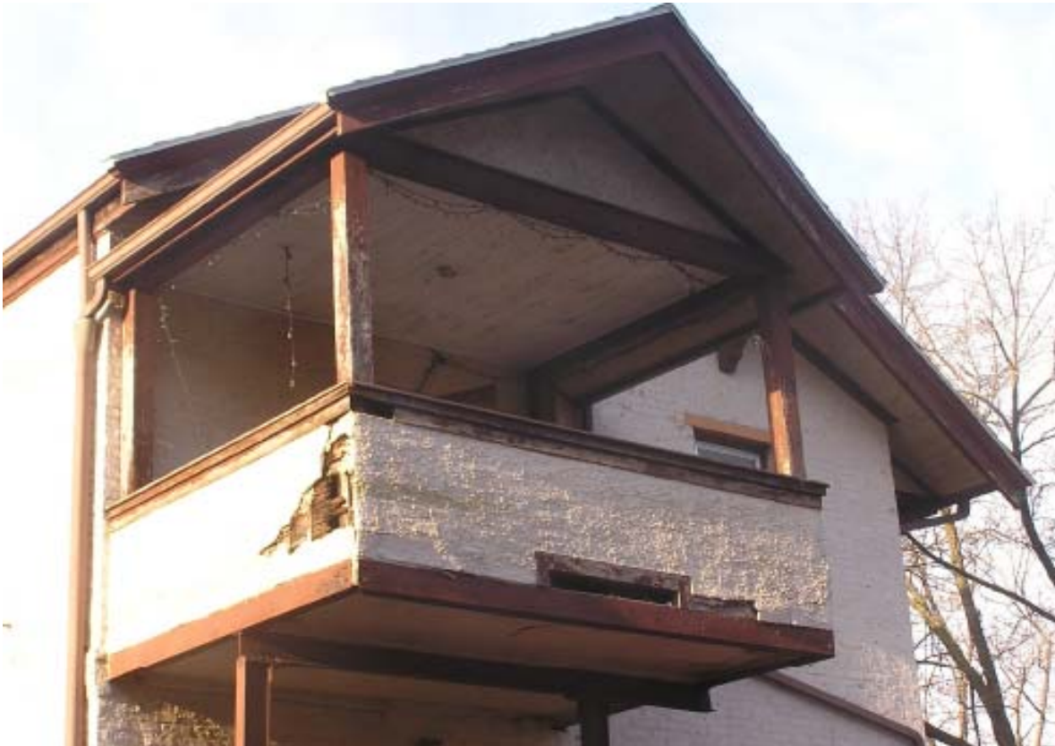
DETERIORATED SIDING, POST AND FASCIA
