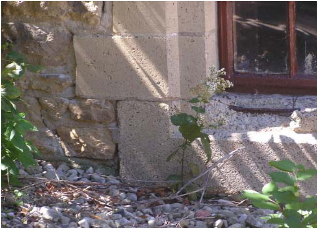
DETERIORATING WINDOW SILL AND CRACKED FOUNDATION
