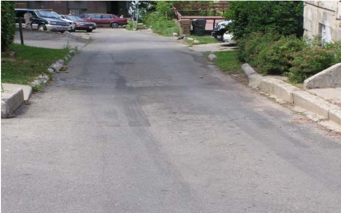
BLIGHTED ALLEY – PAVEMENT IN POOR CONDITION WITH CURB AND GUTTER MISSING
