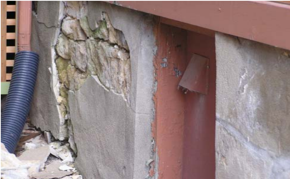
BOARDED UP WINDOW, BROKEN FOUNDATION AND CRACKED PARGET
