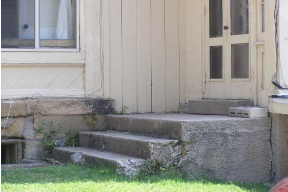
DETERIORATED STEPS, DOOR & WINDOW FRAMES, THREE STEPS WITH NO RAILING AND CRACKED FOUNDATION
