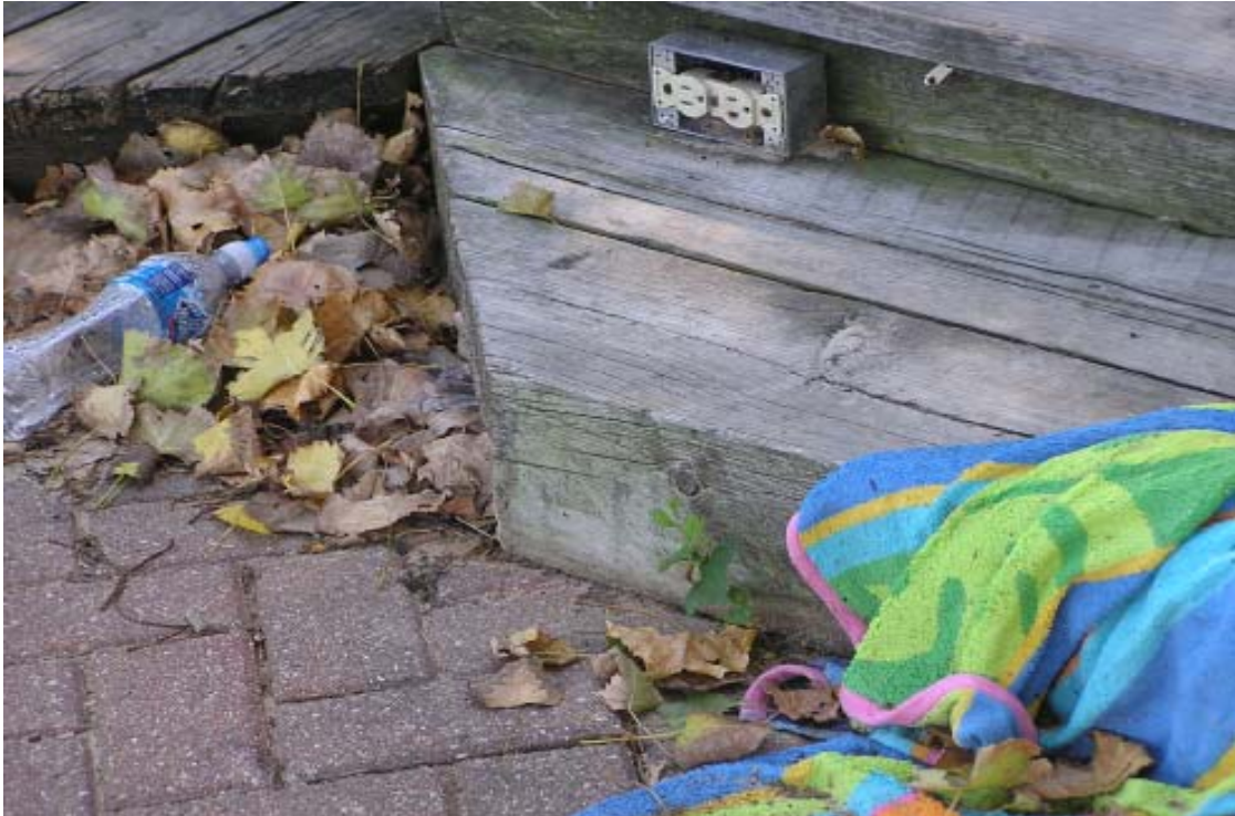
TRASH & EXPOSED ELECTRIC BOX (2of3)
