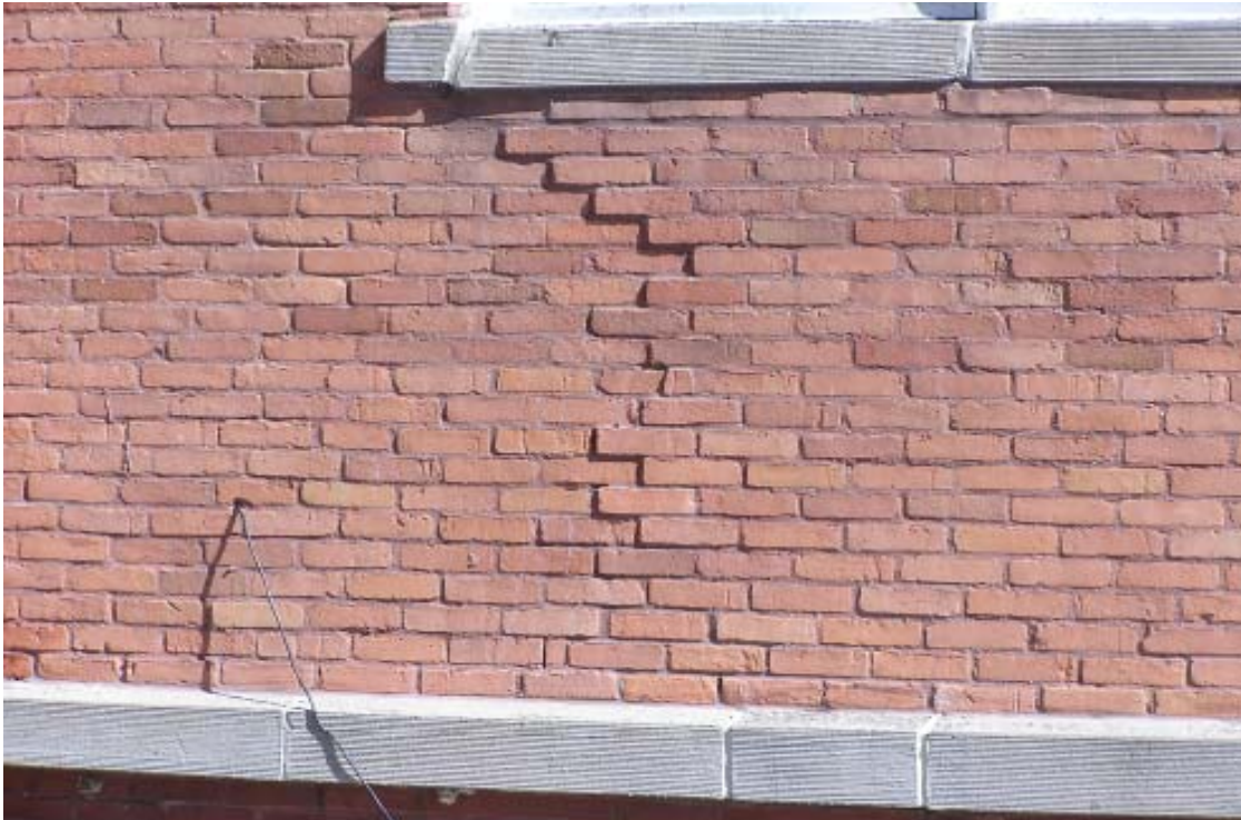
CRACKED WALL (1of3)
