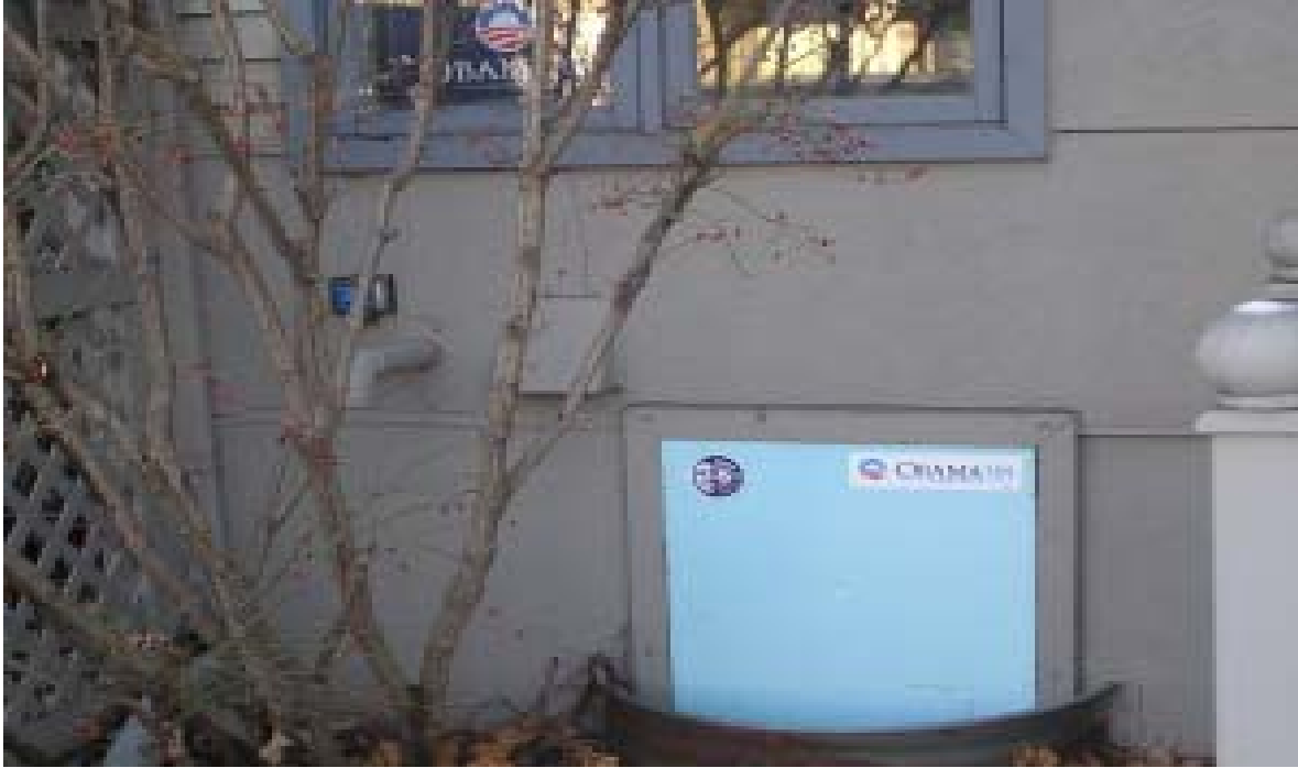
BOARDED UP BASEMENT WINDOW, CRACKED WALL AND DETERIORATED WINDOW FRAME
