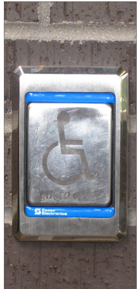
Automatic electronic door openers assist with wheelchair access.
