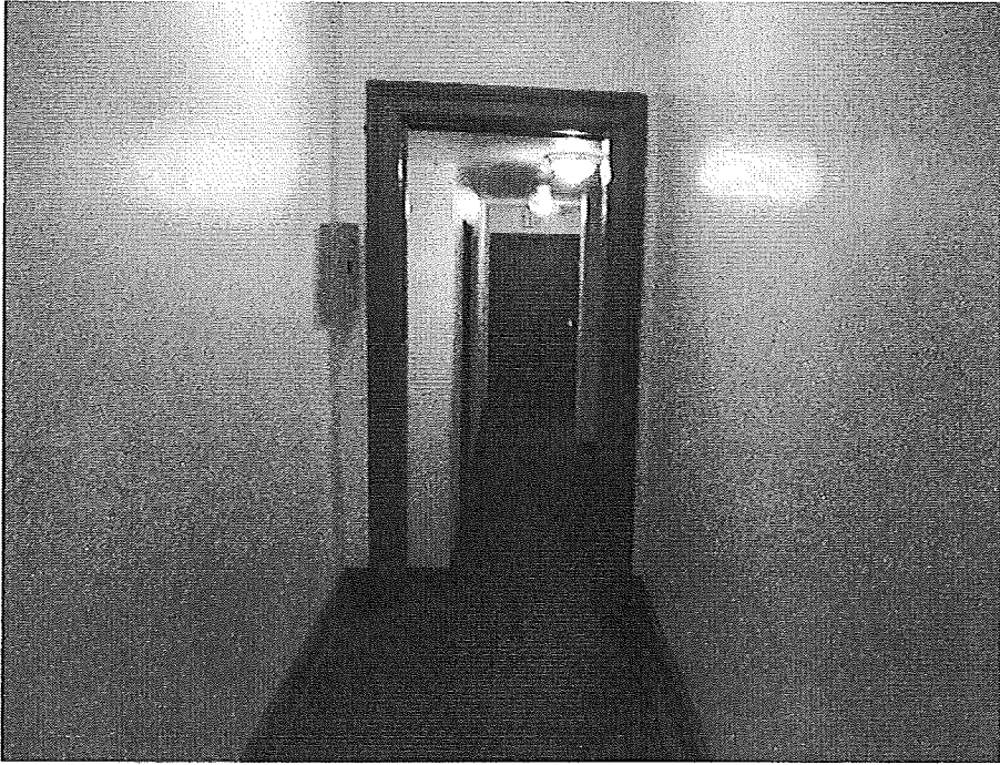
Image showing the sloping in the corridor of second floor from west downward to the east.
