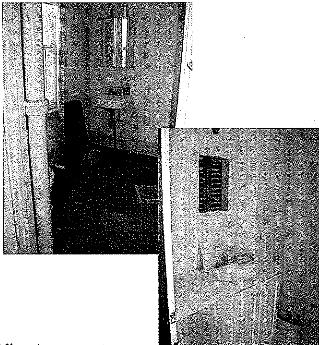
Sub-par bathrooms with out-of-date plumbing and missing toilet.
