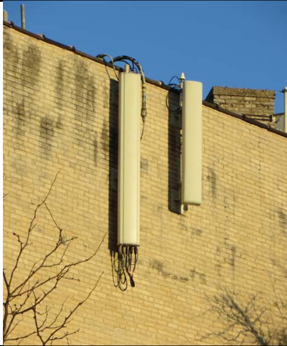
Photo 6 - ZOOM DETAIL OF ANTENNAS ON W WALL OF STRUCTURE
