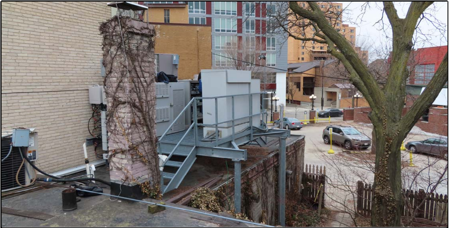
Photo 2 - EXISTING EQUIPMENT CABINETS NEAR REAR OF BUILDING (NOT VISIBLE FROM STREET)
