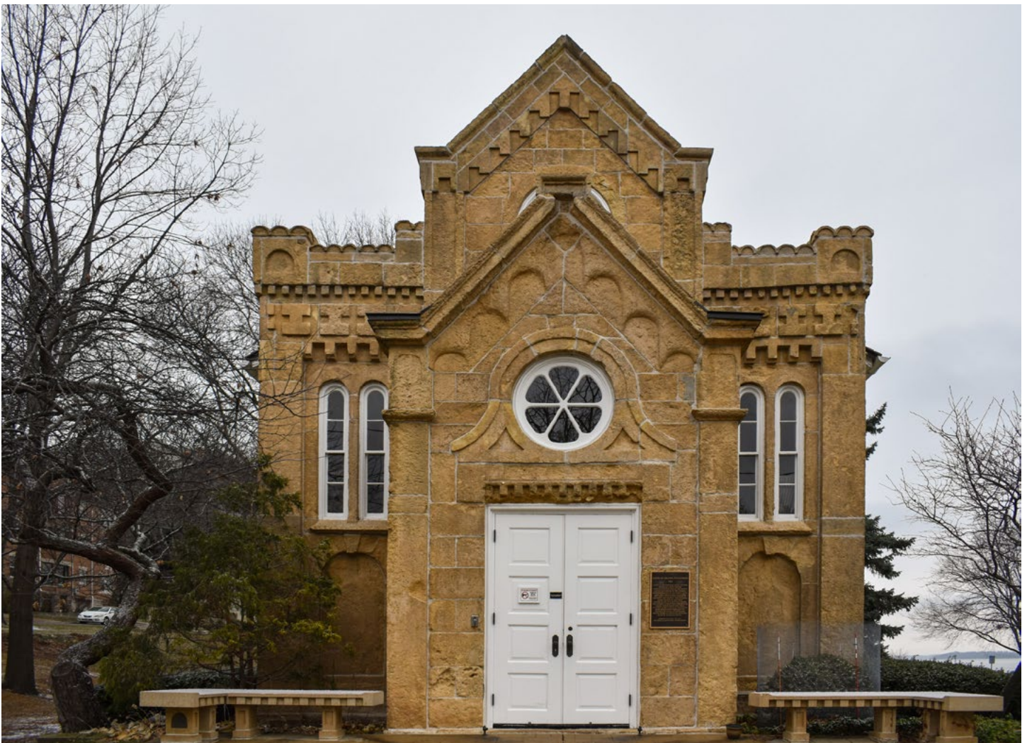
The Madison Branch of Building Restoration Corporation has been awarded the 2022 Historic Preservation Award from the Madison Trust for Historic Preservation. Our Madison branch won for their work on the 159-year-old Gates of Heaven Synagogue.
