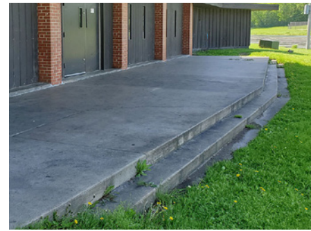
Figure 5.3. Steps at Shelter
