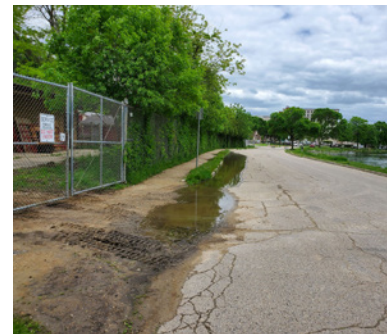
Figure 5.39. Slippage and Longitudinal
