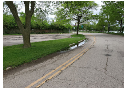
Figure 5.48. Drainage issues at South Lot
