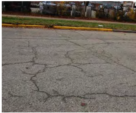
Paterson St at Main St (Fair condition)
