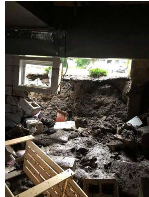
Basement collapse from 2018 flood
