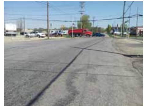
Dempsey Rd. Looking N (fading asphalt)
