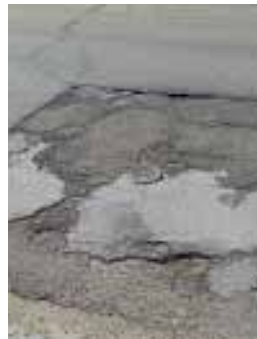
Cottage Grove Rd. (cracks, patched)
