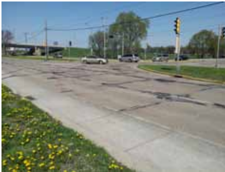
Cottage Grove Rd. at US 51 looking NW (cracks, large patched voids)
