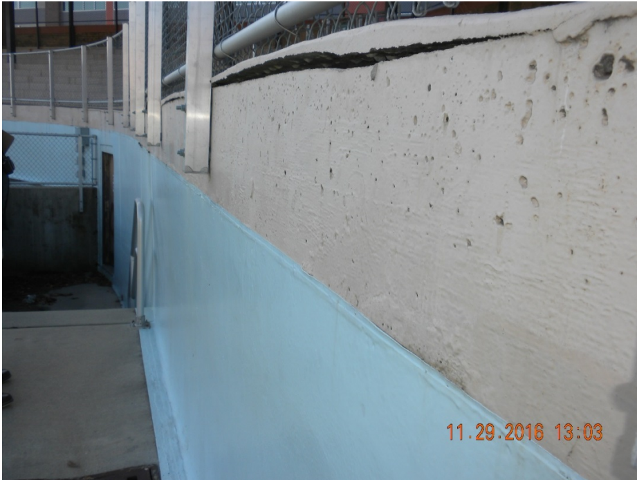
Showing Delamination of the overlay from the 1929 base concrete
