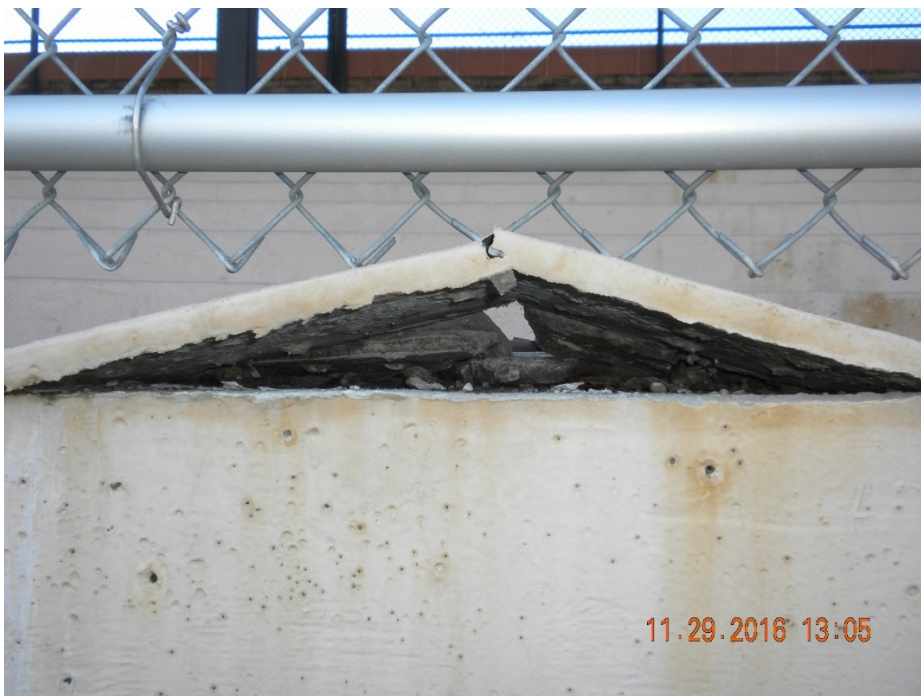
Delamination caused by moisture trapped under the walking surface membrane
