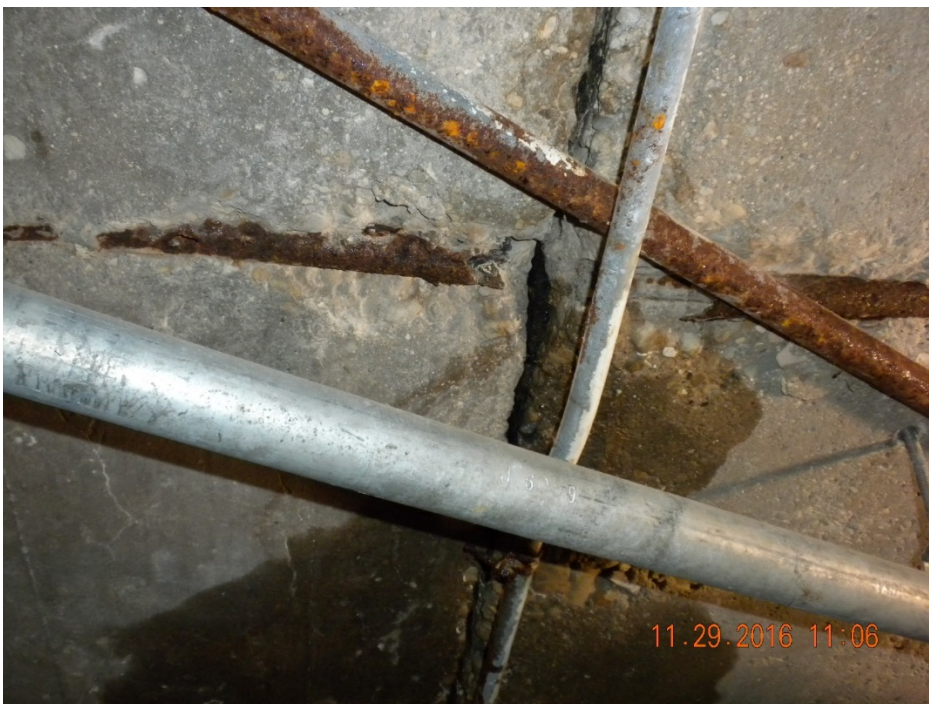
Water getting through the membrane at construction joint, causing damage to reinforcing steel and utility conduits.
