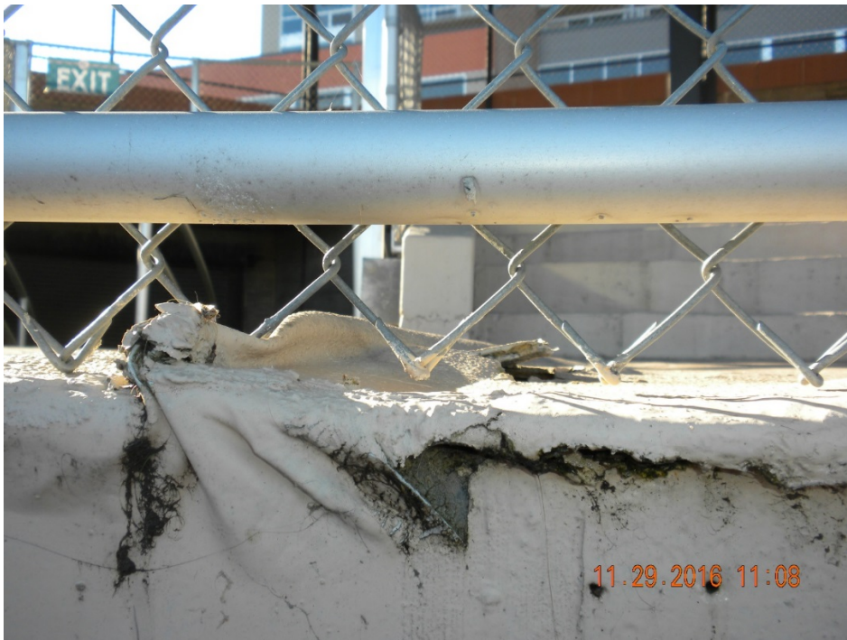
Membrane damage where membrane is placed over a construction joint.
