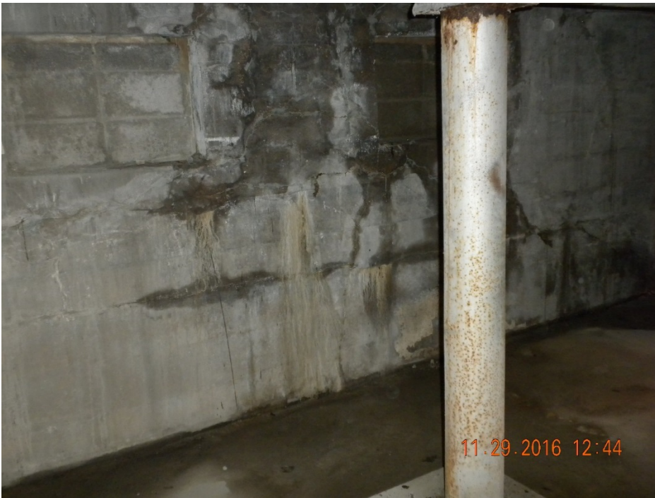
Moisture inside wall at North Dugout. Cracking in exterior wall membrane indicates this area is moving and is required to be stabilized once settlement cause is determined.
