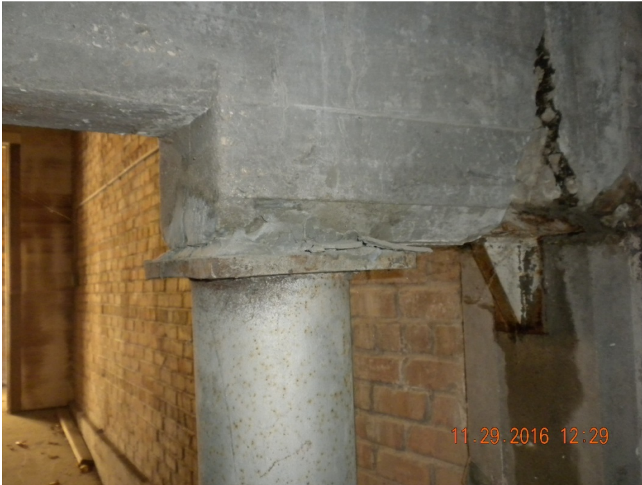
Previous damage to bearing end of concrete beam. Since supported. Support is adequate and in good condition.
