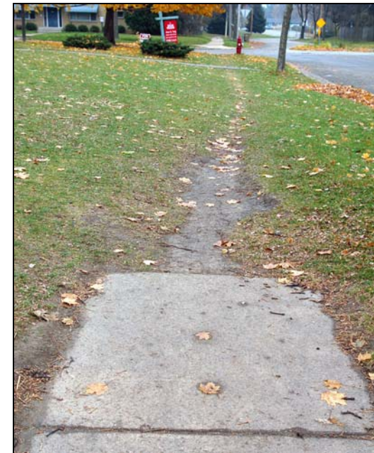
Some sidewalks in the neighborhood start and stop and the plan recommends that they be completed.
