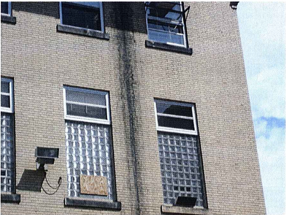
University Avenue & Charter Street Wooden board window patch & water damage April 30, 2007
