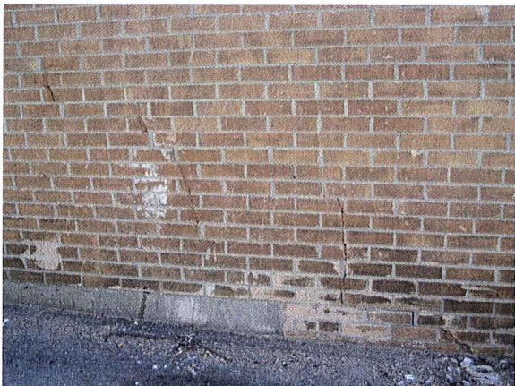
1202 Johnson Street & Charter Street Wall cracks April 30, 2007
