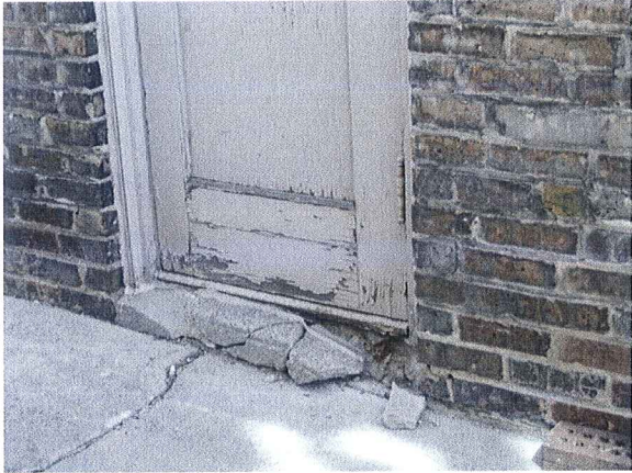
317 Randall Avenue & Johnson Street Deteriorated door & broken sill April 30, 2007
