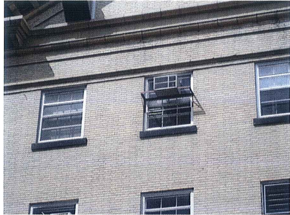
University Avenue & Charter Street Small wall cracks & retro-fitted air conditioning unit April 30, 2007
