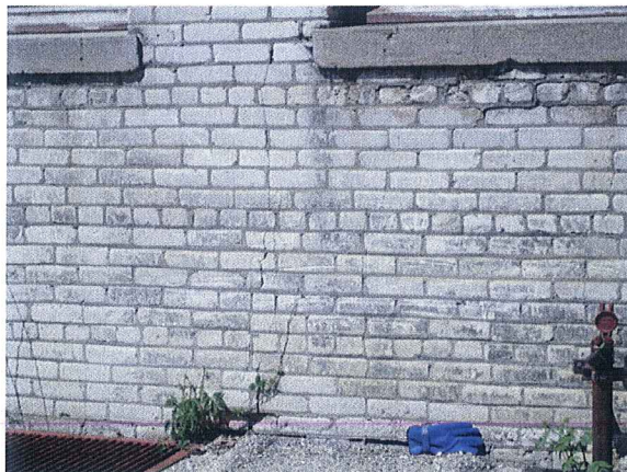
1307 University Avenue Cracked wall & deteriorated window frame April 30, 2007
