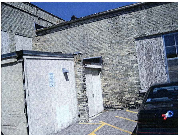
1327 University Avenue Boarded up window, deteriorated wood, wall cracks, broken bricks & rotted wood on the add-on structure April 30, 2007
