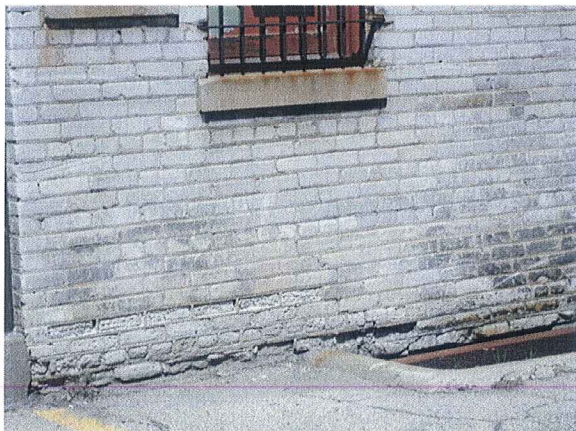
1301 University Avenue Deteriorated bricks, wall crack & barred windows April 30, 2007
