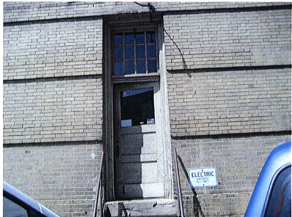
University Avenue & Orchard Street Deteriorated door, door frame and sill April 30, 2007
