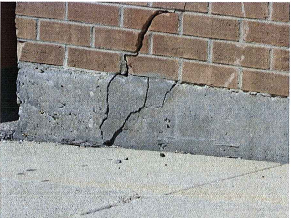
1202 Johnson Street & Charter Street Cracked foundation & walls; chipped brick April 30, 2007
