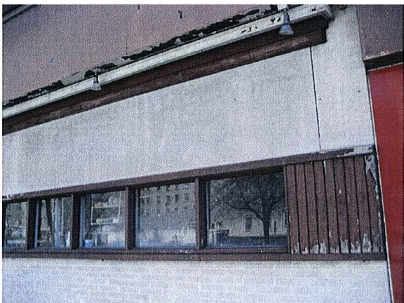
1313 University Avenue Deteriorated sign & deteriorated window frames April 30, 2007
