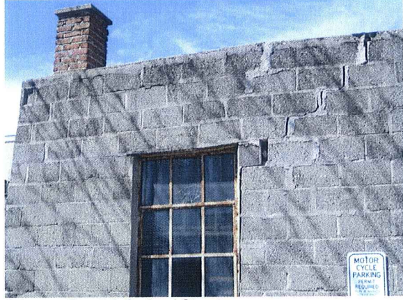
Johnson Street & Orchard Street Broken window & rusted window frame, deteriorated chimney and cracked wall April 30, 2007
