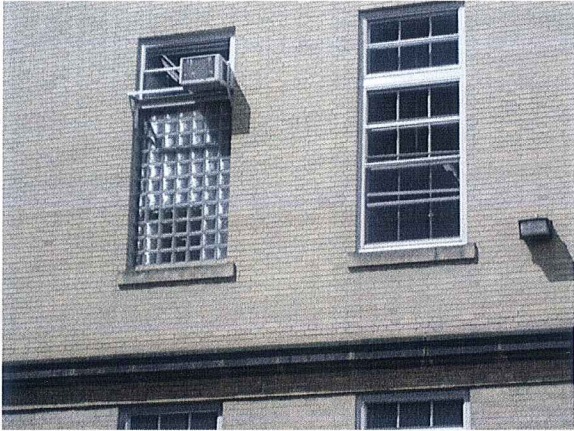
University Avenue & Charter Street Blocked up window & retro-fitted air conditioning unit April 30, 2007
