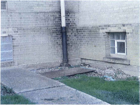
University Avenue & Orchard Street Blocked up windows & deteriorated foundation April 30, 2007
