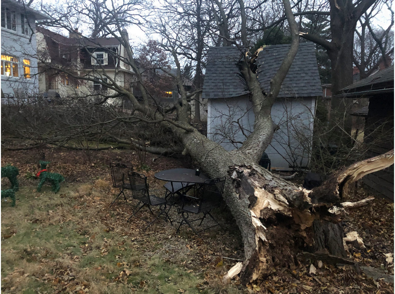
Exterior photo of the damaged gable shed (viewed from the west). The color of the new shed will match the old shed and therefore the house (left).
