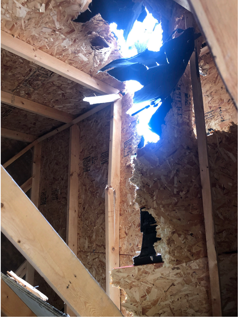
Interior photo of the damaged gable shed showing cracked wall and roof framing.
