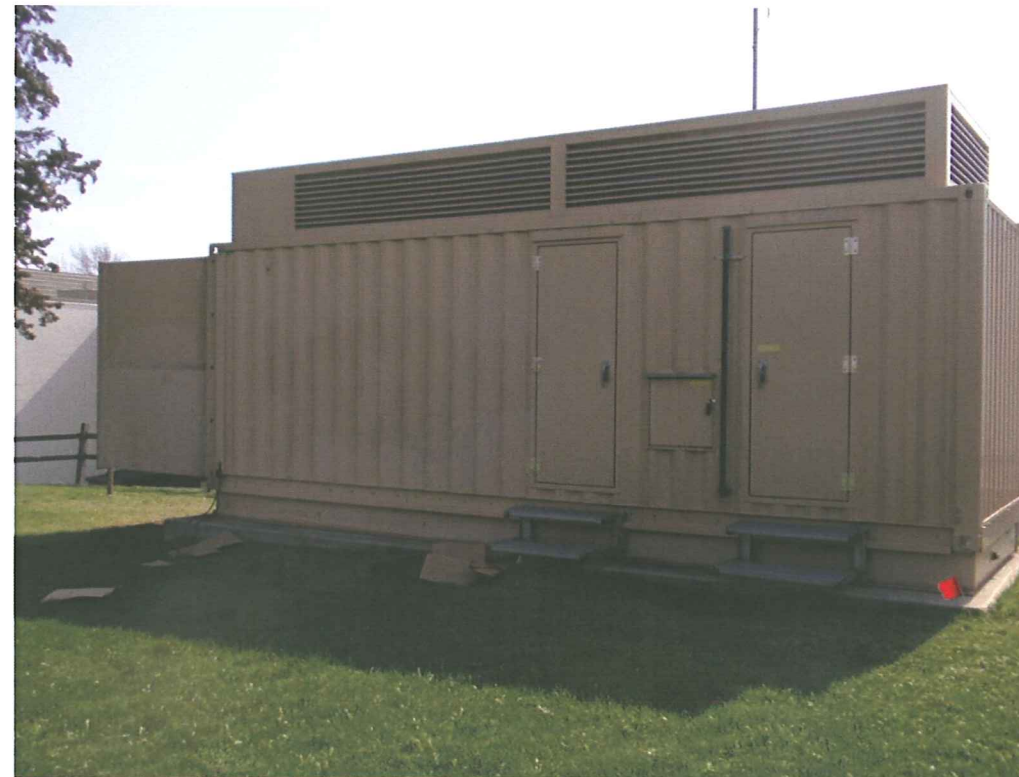
Picture 8 Generator set to south of existing buried reservoir.
