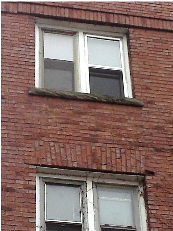
Image 1.55 Steel lintels (for windows) are in various forms of disrepair. The lintels are experiencing expansion from moisture-related corrosion, and in-turn, the surrounding brick unit masonry is damaged by its forces.
