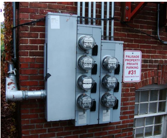
Image 1.36 Electrical entrance and meters.
