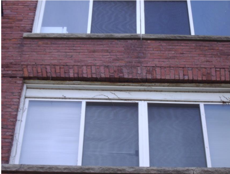
Image 1.54 Severe rust-jacking between the steel angle lintel and the brick flat arch above the window.
