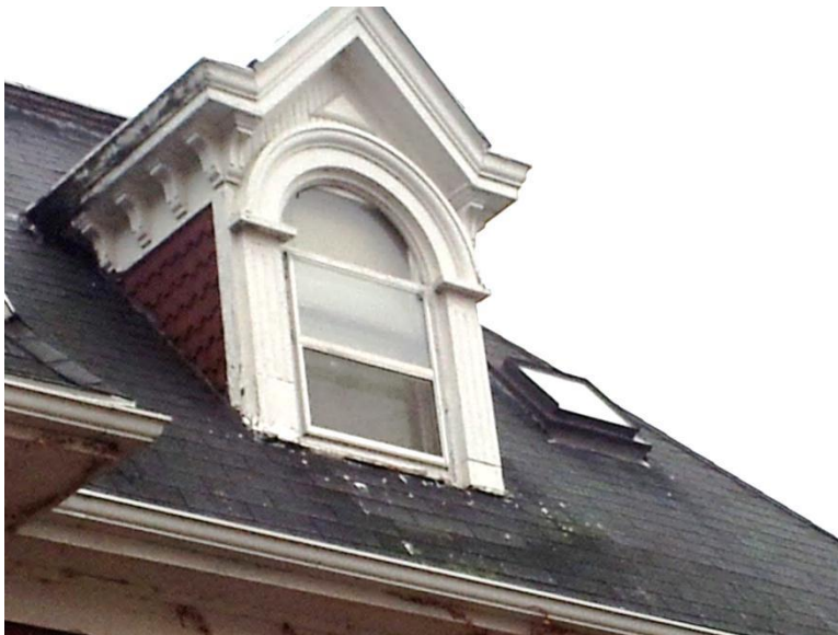
Image 1.4 The gables and dormer walls originally featured beaded board and shingle siding and major portions of these areas are presently exposed and functioning. Areas exposed to view appear to be rotting and otherwise deteriorating
