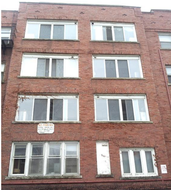
Image 1.53 The brick masonry is largely in good condition, but it contains evidence of instability including wall length expansion with associated vertical and horizontal cracking, deviating vertical wall plane, and protruding brick units.
