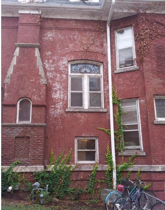
Image 1.3 The brick masonry observed is largely in good condition, but it contains evidence of minor instability in the form of step-cracking. There is also efflorescence at several locations indicating moisture penetration of the masonry.
