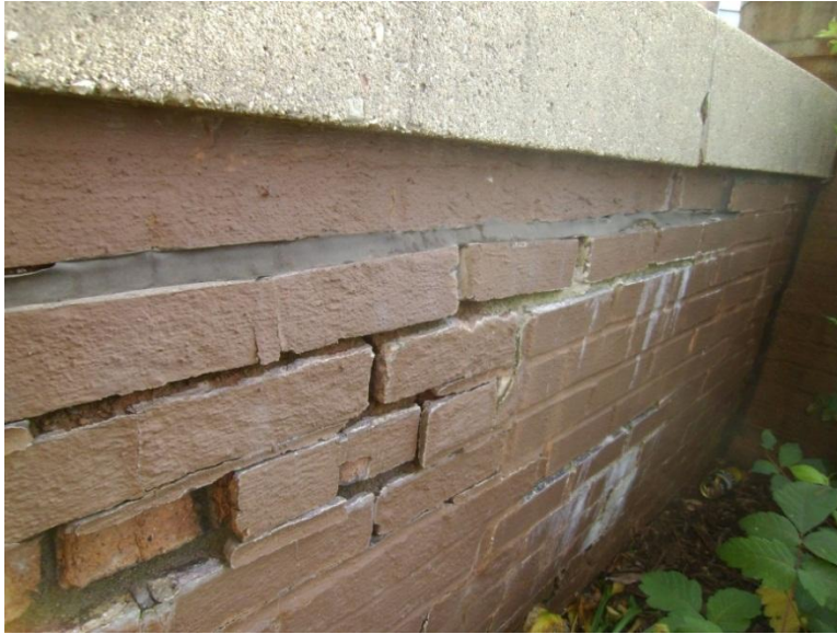
Image 1.45 Image showing the damaged and collapsing north side retaining wall of the front entry stoop.
