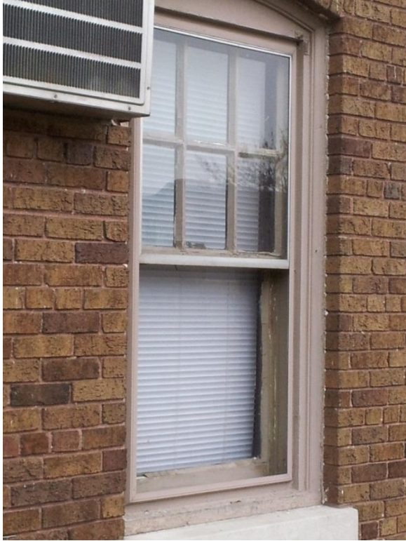
Image 1.42 View original wood windows are in place with modern-generation combination storms at their exterior exposure. The style of the original windows is single-hung.
