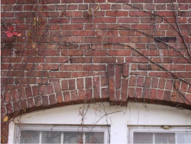
Image 1.30 View showing a failing masonry arch at an opening.
