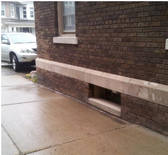
Image 1.39 View of concrete driveway pitched towards foundation wall allowing rain and snow melt water to enter basement area.
