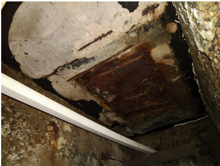
Image 1.13 View showing the exterior vault and steel cover connected to the basement. The steel framing embedded in the concrete foundations are corroded and damaged.
