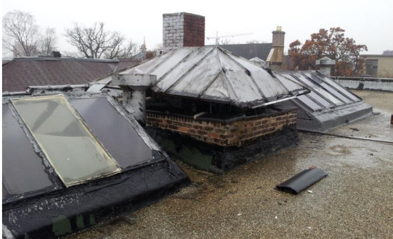
Image 1.28 Roof appurtenances and conditions. Glazing of the skylights is largely intact but fractured. Leaks to the interior were observed.
