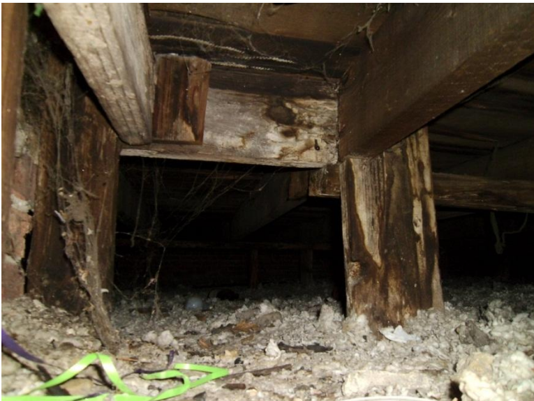
Image 1.31 showing heavily stained wood framing of the sloped roof. Portions of the framing are likely deteriorated.
