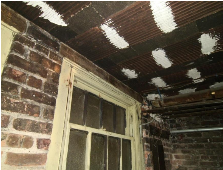
Image 1.19 View showing the exterior bearing wall from the interior. Note the concrete lintel construction over the opening and one way concrete joist with clay tile infill construction of the first floor.
