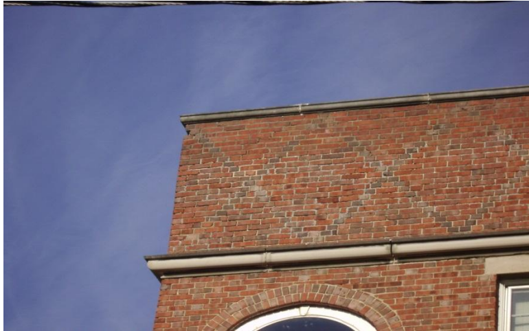
Image 1.20 View of the front parapet. The parapet was rebuilt yet still has deterioration occurring. Moisture is penetrating the perimeter walls at open joints in the parapet coping and in the limestone band trim.
