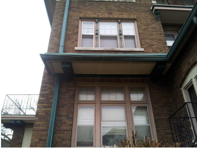
Image 1.44 Portions of the gutters and downspouts are deformed and/or detached from the substrate.
