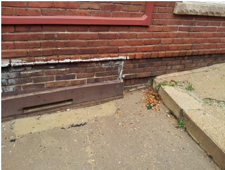
Image 1.52 Moisture is penetrating the perimeter walls below-grade. This is most noticeable at the southwest elevation walkway slab contour. Exterior Walls
