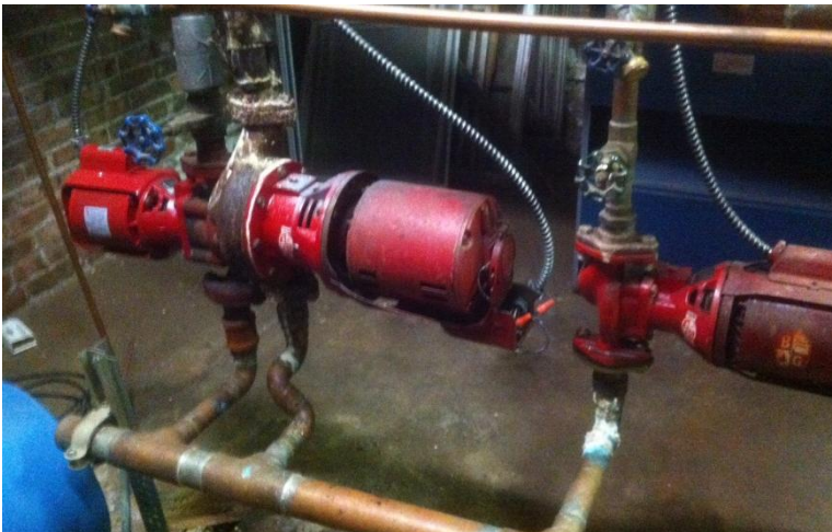
Image 1.50 View of boiler hot water circulating pumps in the mechanical room.
