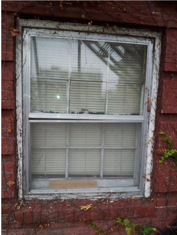
Image 1.5 Original wood windows are in place with modern-generation combination storms at their exterior exposure. The style of the original windows is single-hung.
