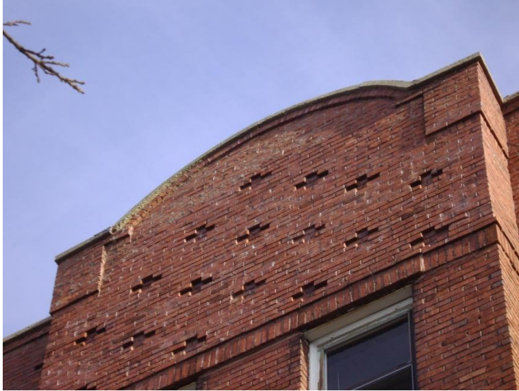
Image 1.60 View showing the top of the front of the building. Note the entire curved upper section is leaning backward.
