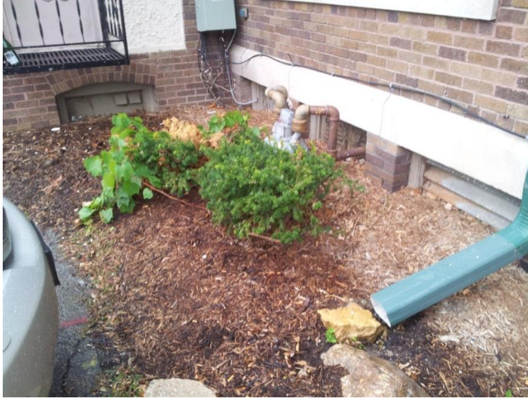
Image 1.40 View of small softscape area at the southwest corner of the building. Water is trapped here and percolates into the soil penetrating the perimeter walls below-grade.
