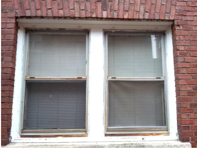
Image 1.58 Original wood windows are in place with modern-generation combination storms at their exterior exposure. The style of the original windows is single-hung. Original porches contain modern-generation window units.
