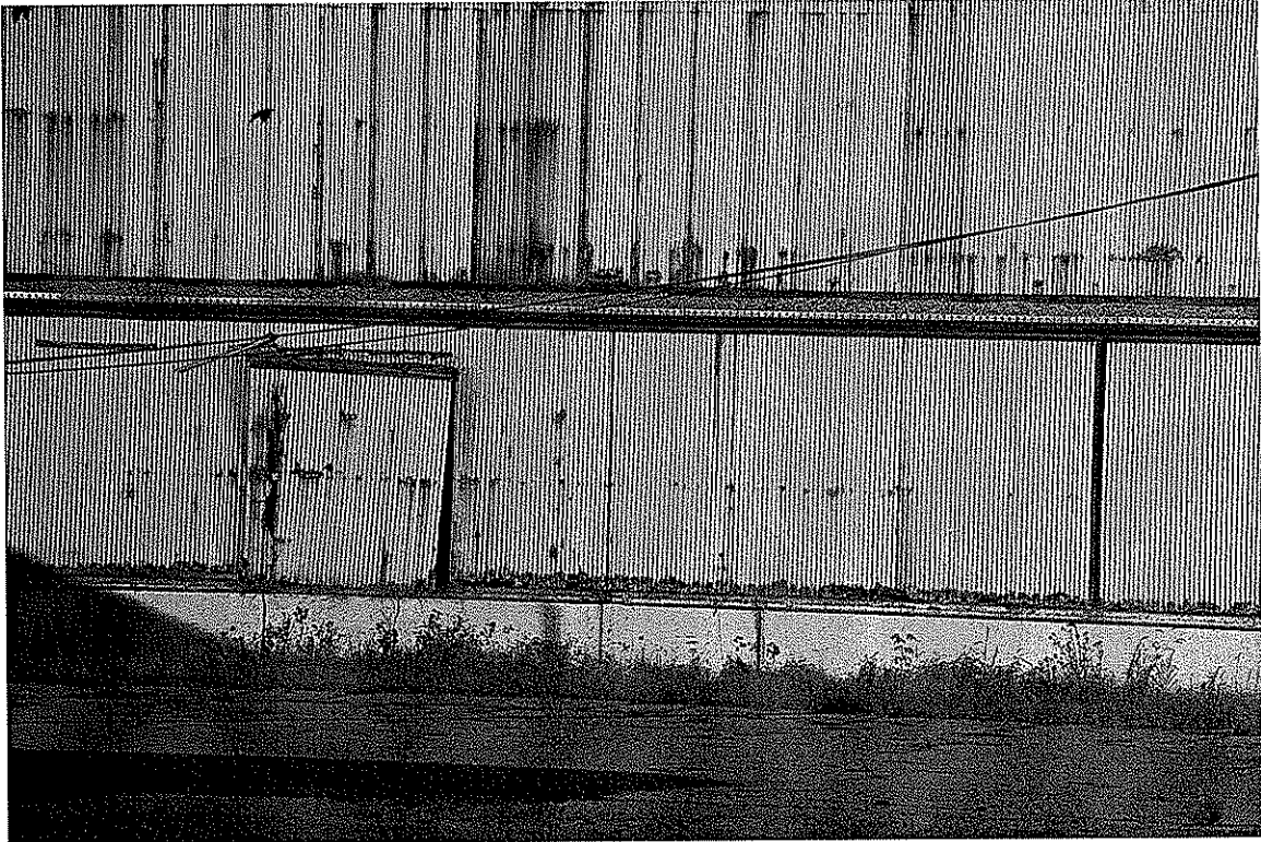
Condition of walls and doors on exterior of granulation building, October 2008
