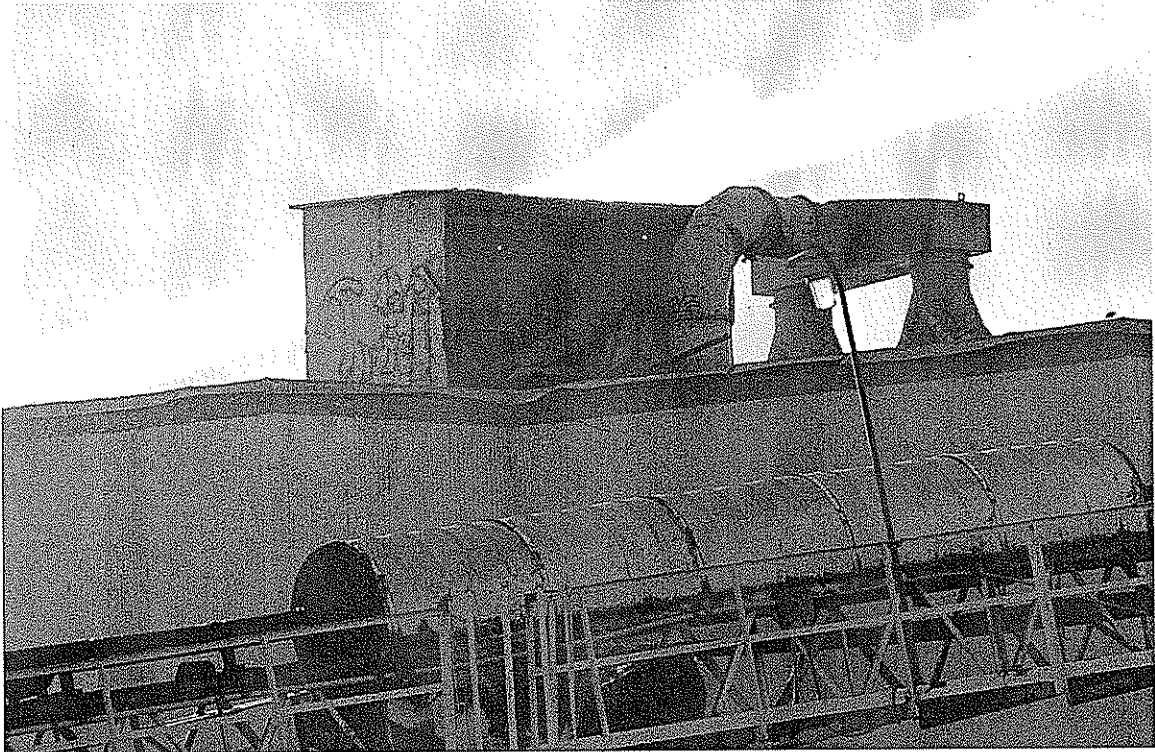
Top of granulation building with graffiti and missing siding, October 2008
