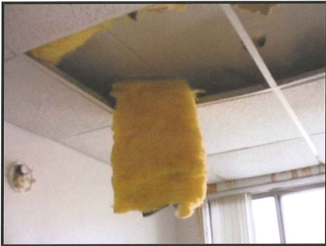
Additional water damage from leaking roof
