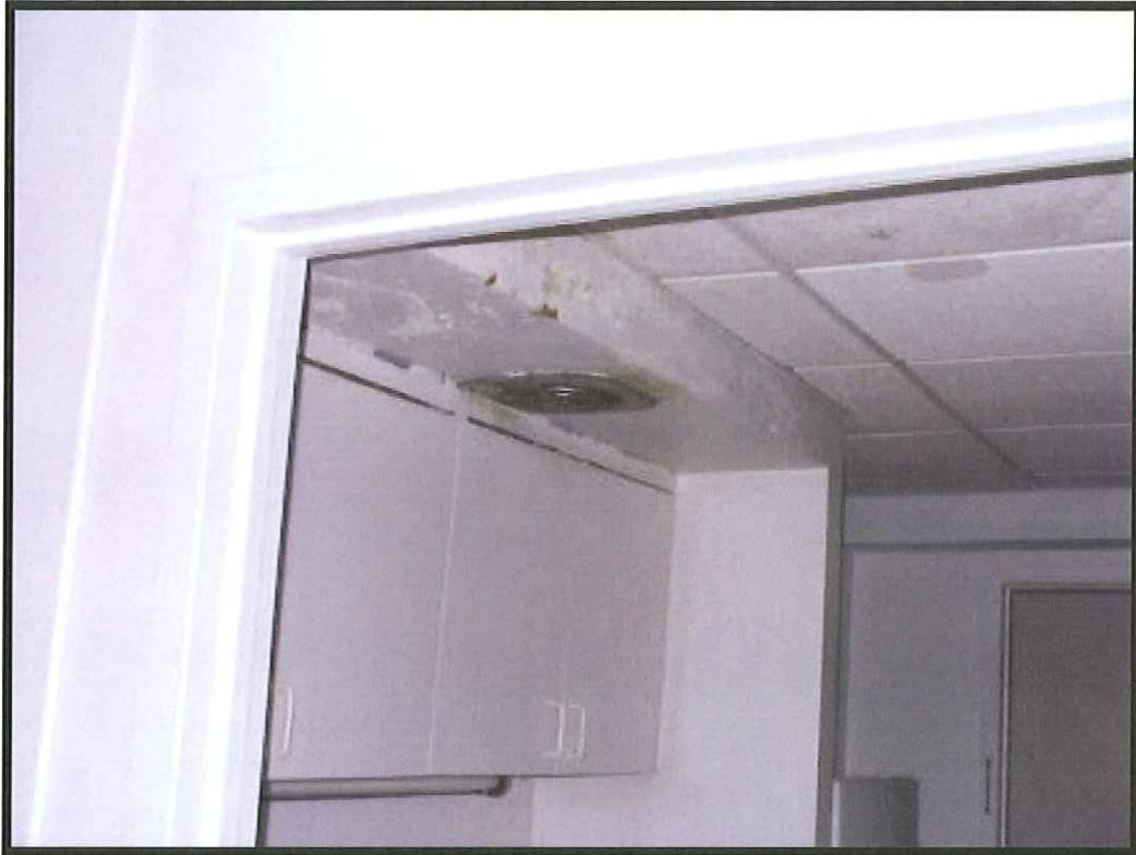
Water damage in kitchenette
