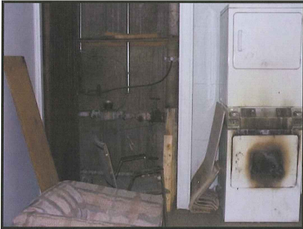
Fire damage in basement storage area
