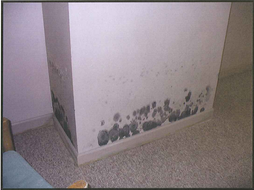
Water damage in TV lounge
