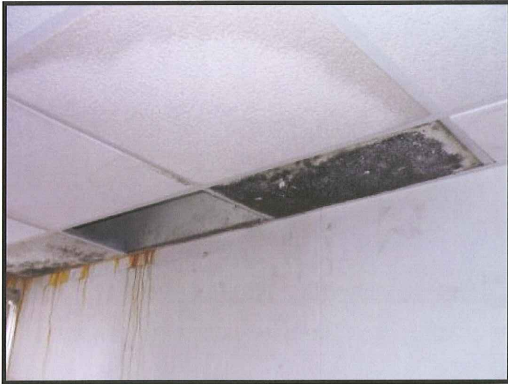
Water damage due to leaking roof
