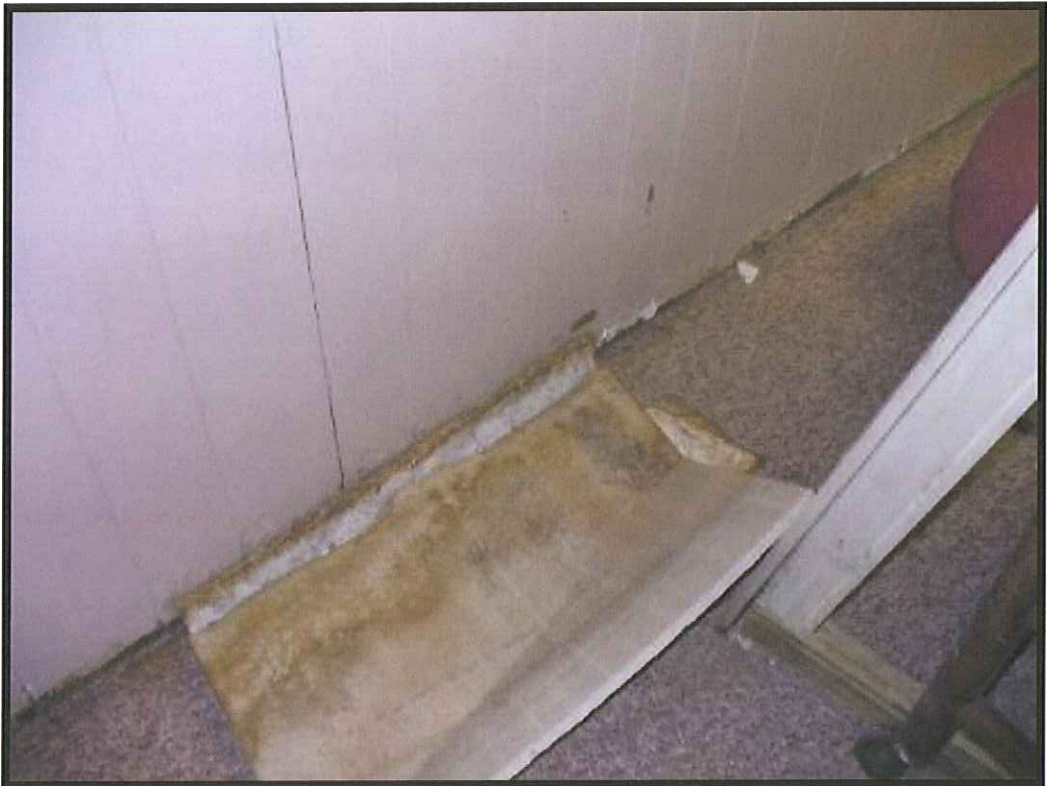
Additional water damage
