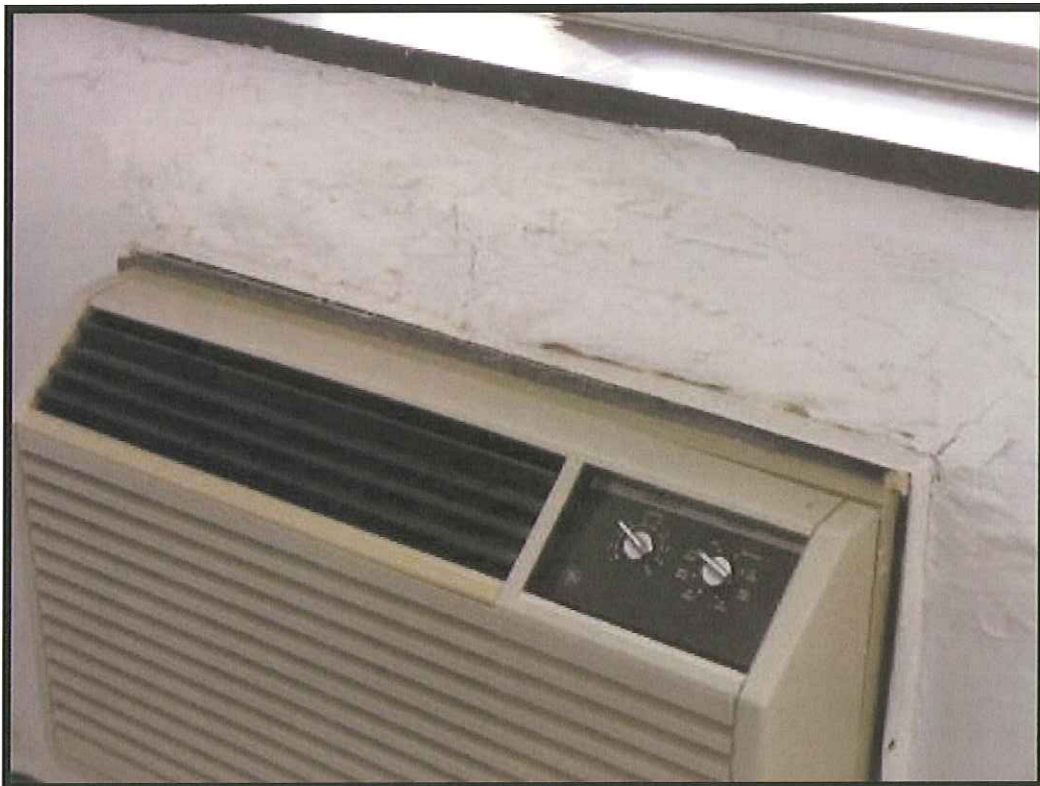
Apartment air conditioner
