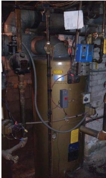
Hot water boiler
