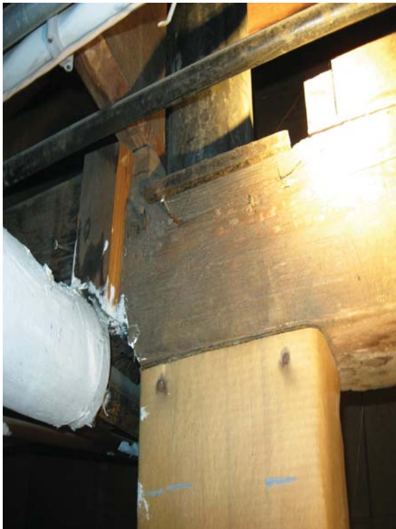
Photo 1 – Notched 1 st floor beam requiring replacement
