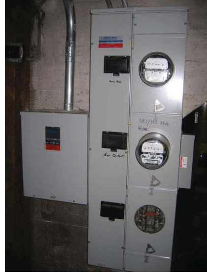
The newer electrical meters in the Basement.
