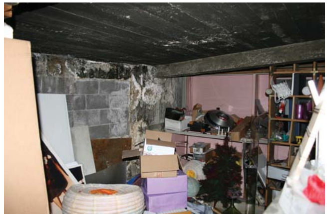
Basement: View of area below an entry ramp to the first floor retail
