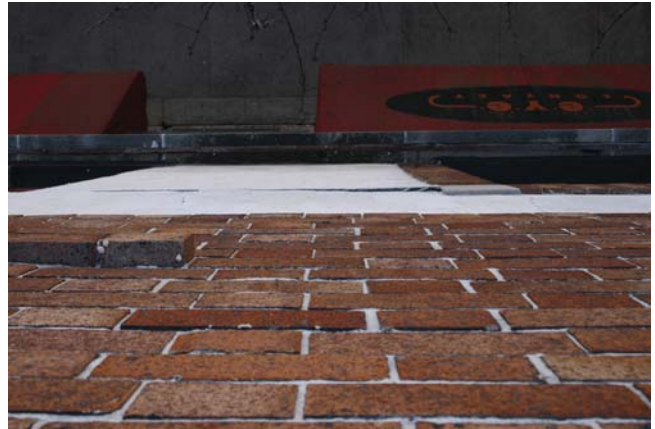
Exterior: View from roof of plaster-coated wall surface showing delamination of the plaster coating
