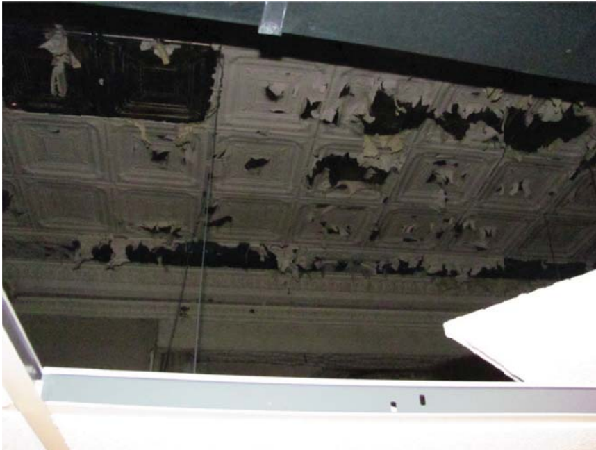
Figure 18. A suspended acoustic tile ceiling conceals other similar original pressed metal ceilings. The full extent of the pressed metal ceiling finish is not known.
