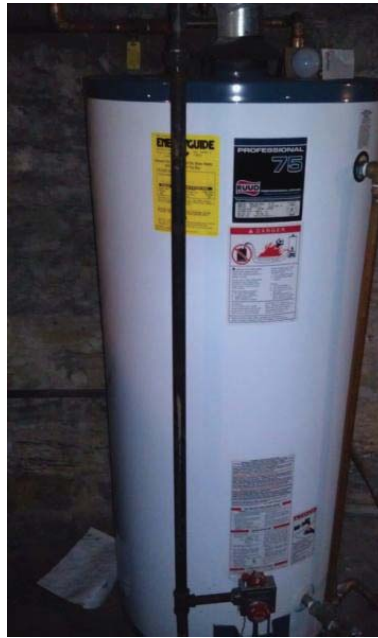
New water heater
