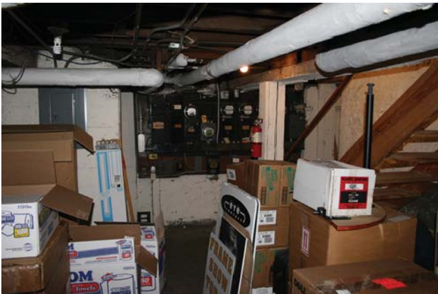
Basement: View of electrical
