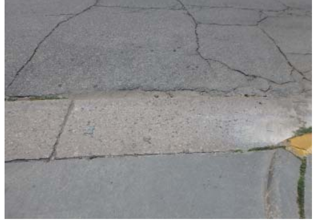
Ramp entry drive on Pinckney Street (Poor condition)
