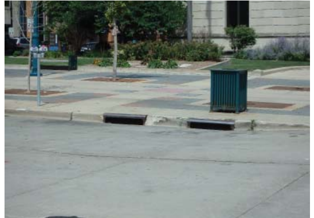
Martin Luther King Jr. Blvd, curbs missing chunks (Fair to Poor condition)
