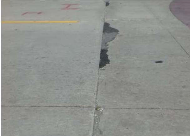
Martin Luther King Jr. Blvd, asphalt patches (Fair to Poor condition)
