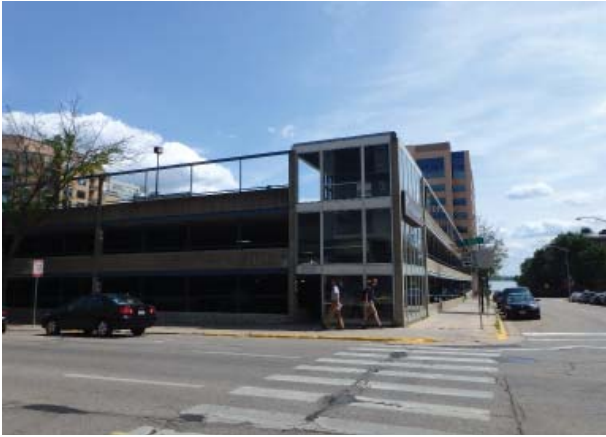
Intersection of Doty and Pinckney looking East (Fair to Poor condition)
