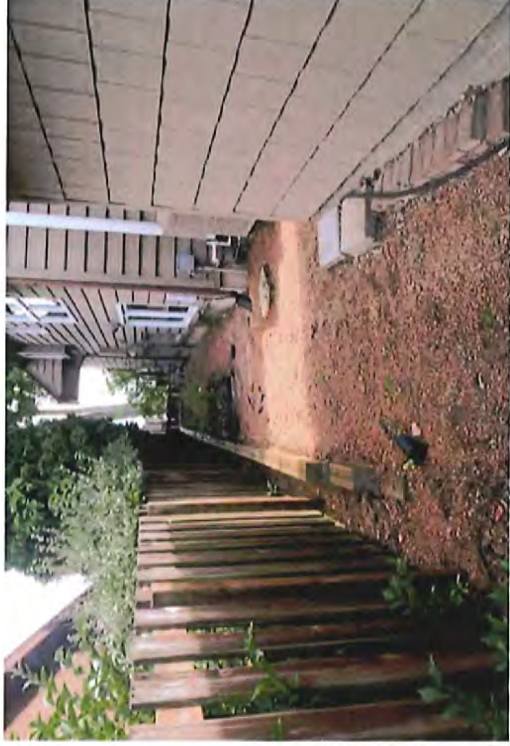
South property line looking towards lake (View of landscape timber wall, fence, and downspout discharge on adjacent property)
