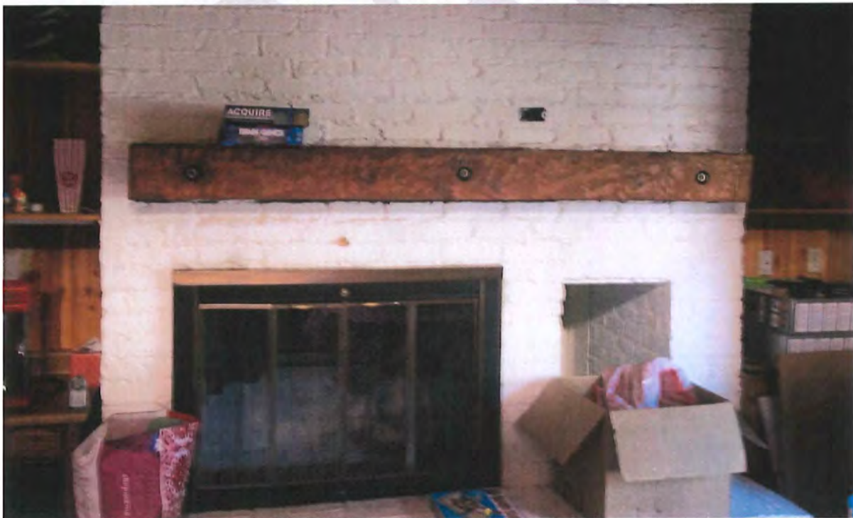
Item #18 Fireplace Timber Mantels.
