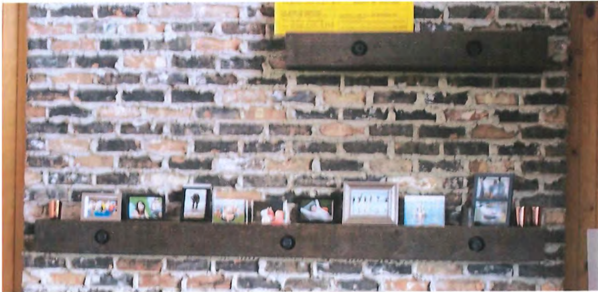
Item #18 Fireplace Timber Mantels.
