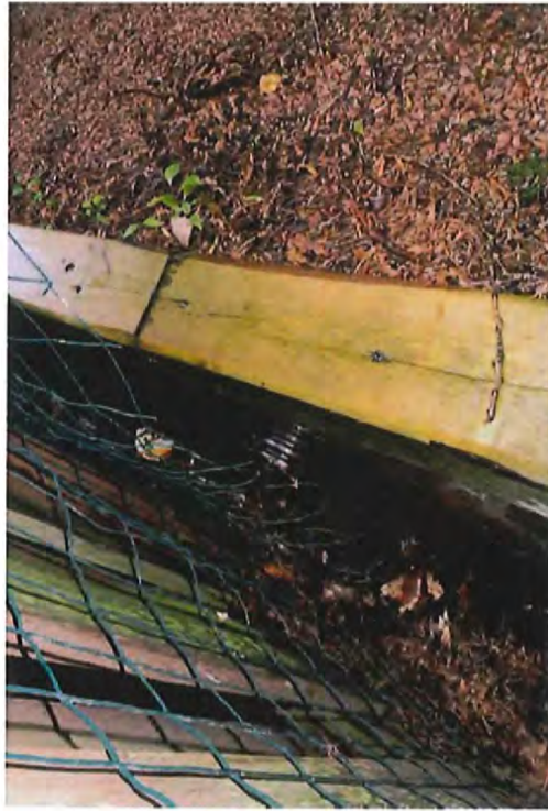
South property line looking towards lake (View of downspout discharge from adjacent property)
