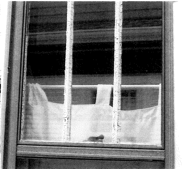
Dry Rot, Failed Glazing
