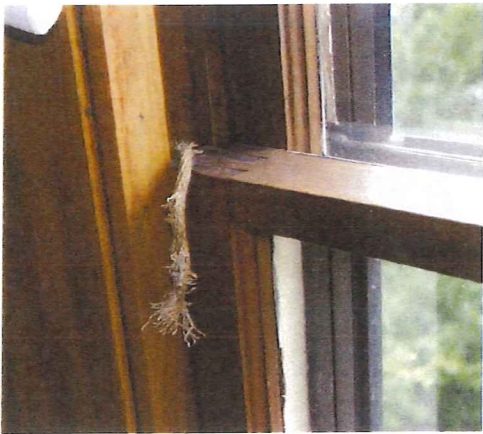
Pulleys and Weights Broken
