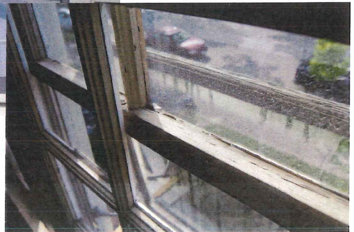
Dry Rot, Failed Glazing
