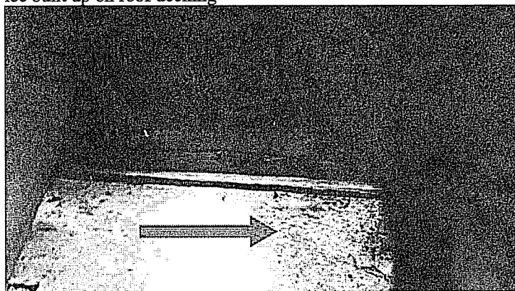
Mold on roof decking
