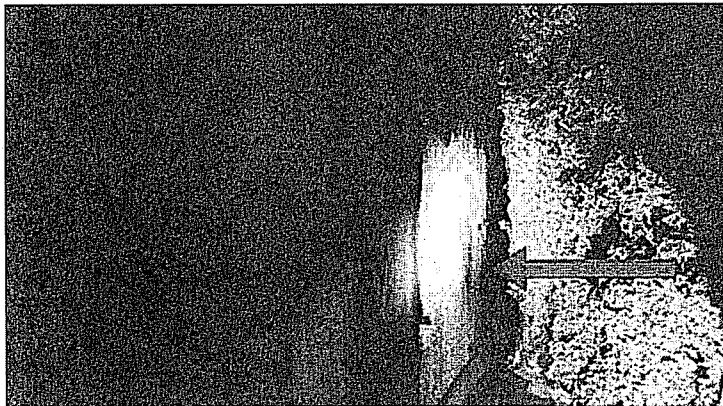
ice built up on roof decking
