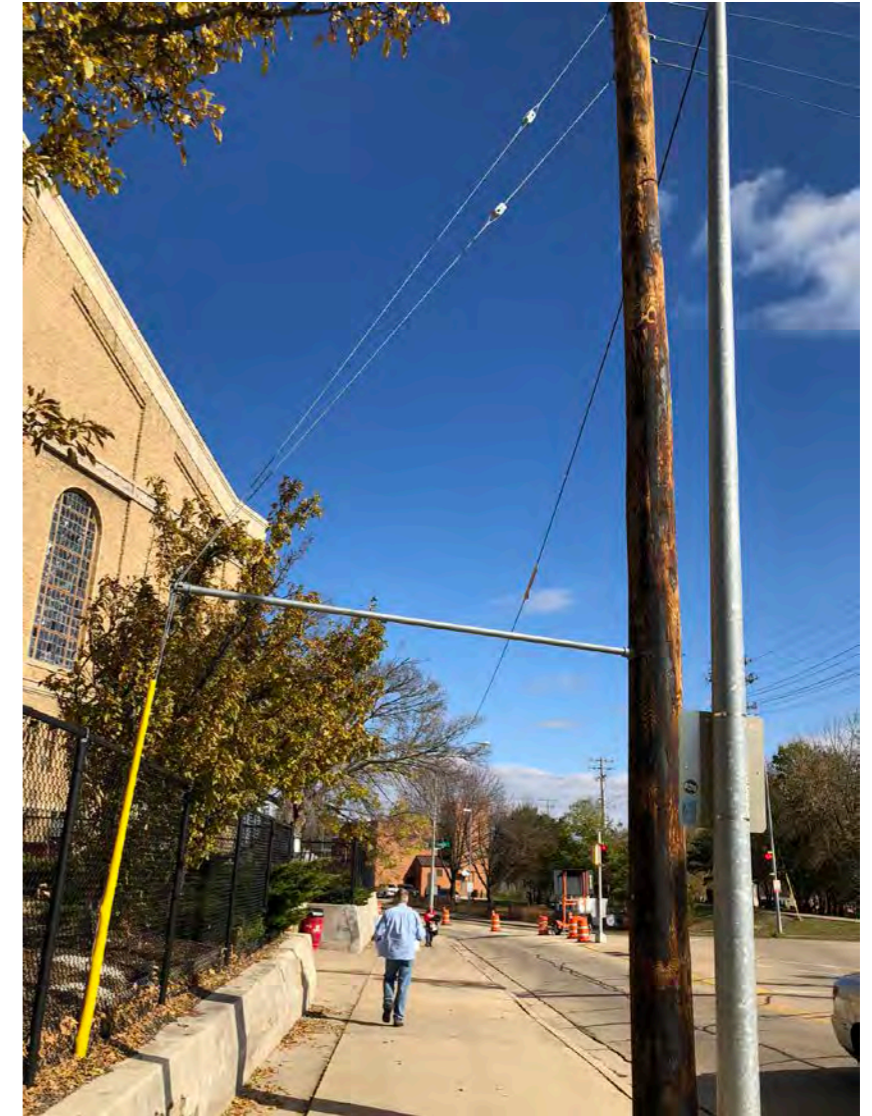
Utility Support Pole
