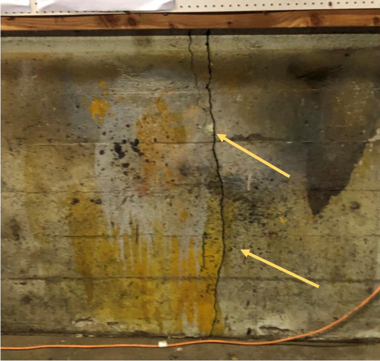
Image showing an unrepaired crack in the foundation wall separating the original building from the first addition along East Dayton Street
