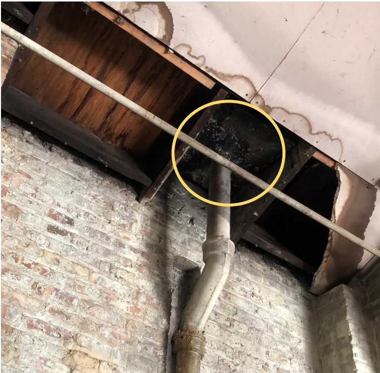
Image showing minor damage below roof pitch pocket drain pan.
