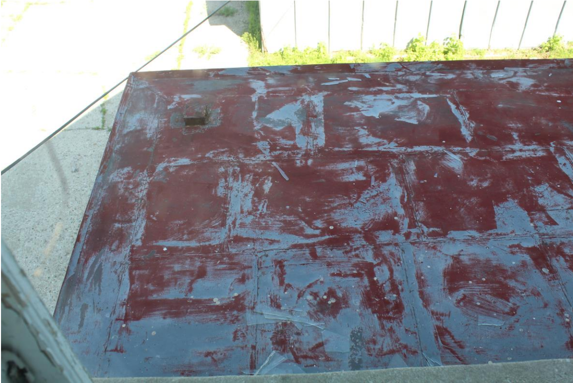
Looking down on original tin roof on rear porch. Tin with folded joints.
