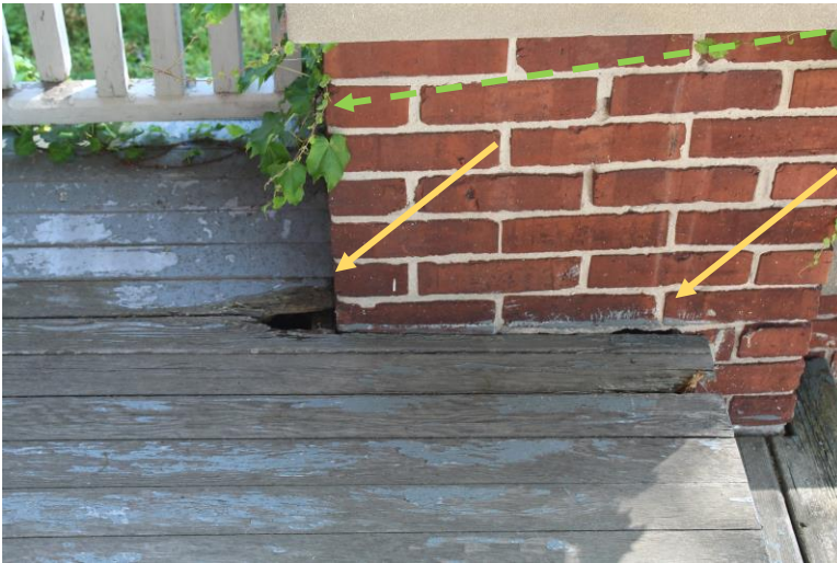
Deteriorate front porch floor and tilting brick column.
