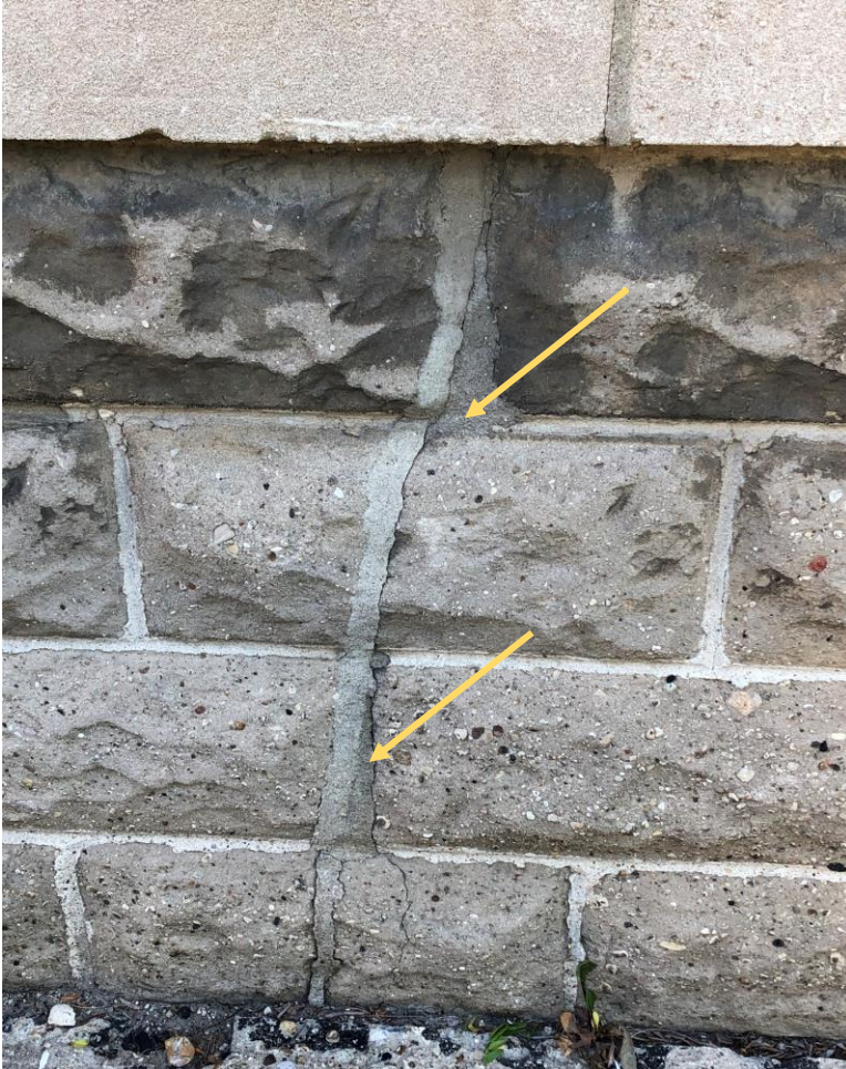
Crack through foundation wall, repaired with hard Portland mortar.
