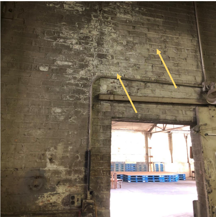
Image showing possible water infiltration from the roof in the form of calcium salt efflorescence.
