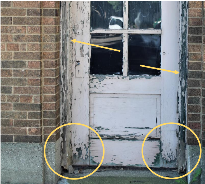
Deterioration of the right-side front door
