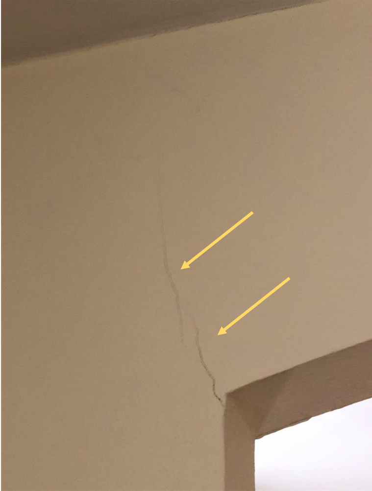
Image of crack in first floor plaster wall of living room.
