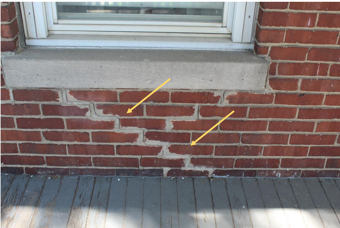
Step crack in brick masonry at corner of front porch. Inappropriate Portland mortar.
