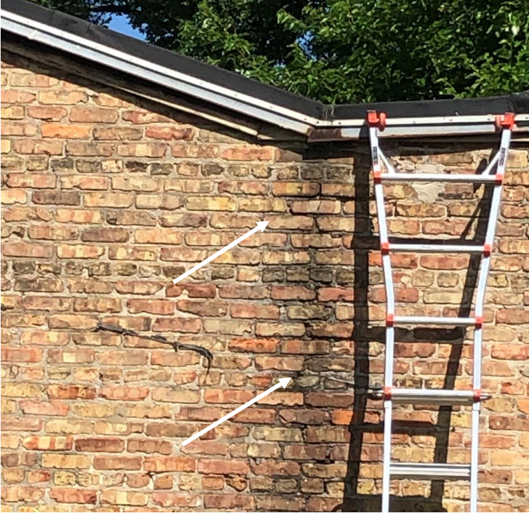
Mortar erosion along south wall of the original building.
