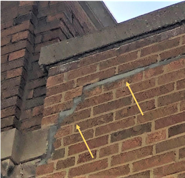
Juncture of original building and west addition along Dayton Street. Note structural crack and previous repairs.
