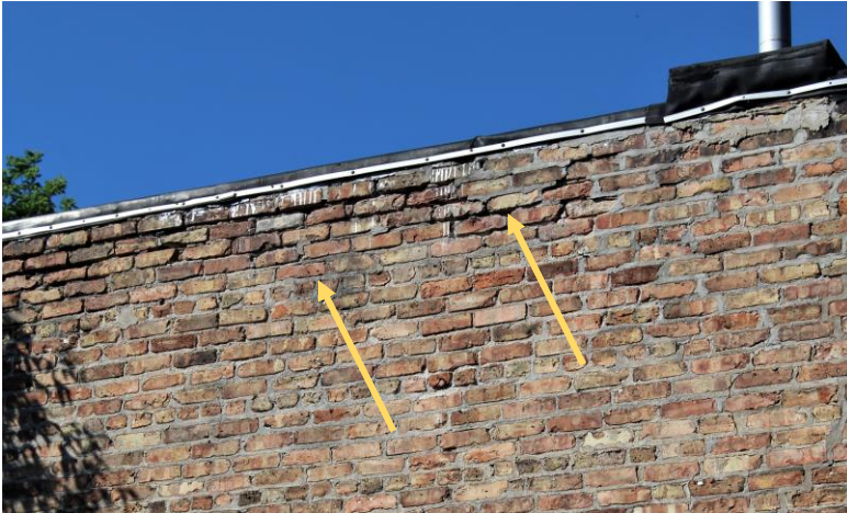
Deterioration of the east parapet. Common bond brick pattern.
