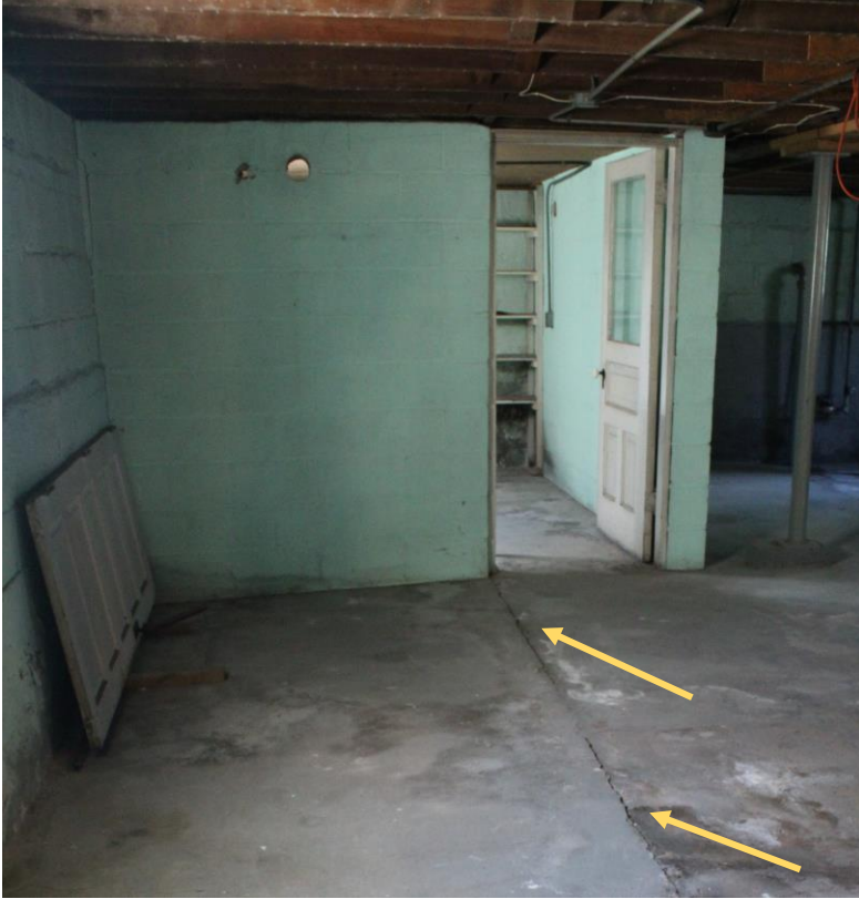
Unfinished basement area. Line of heaved floor slab shown.
