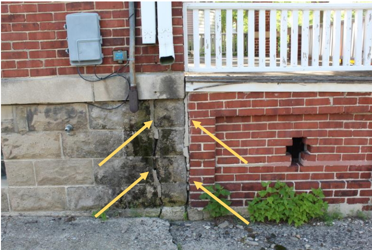
Area of settlement at southwest corner of house at junction with porch. Significant foundation cracking. Rain and snow melt water ponding here.
