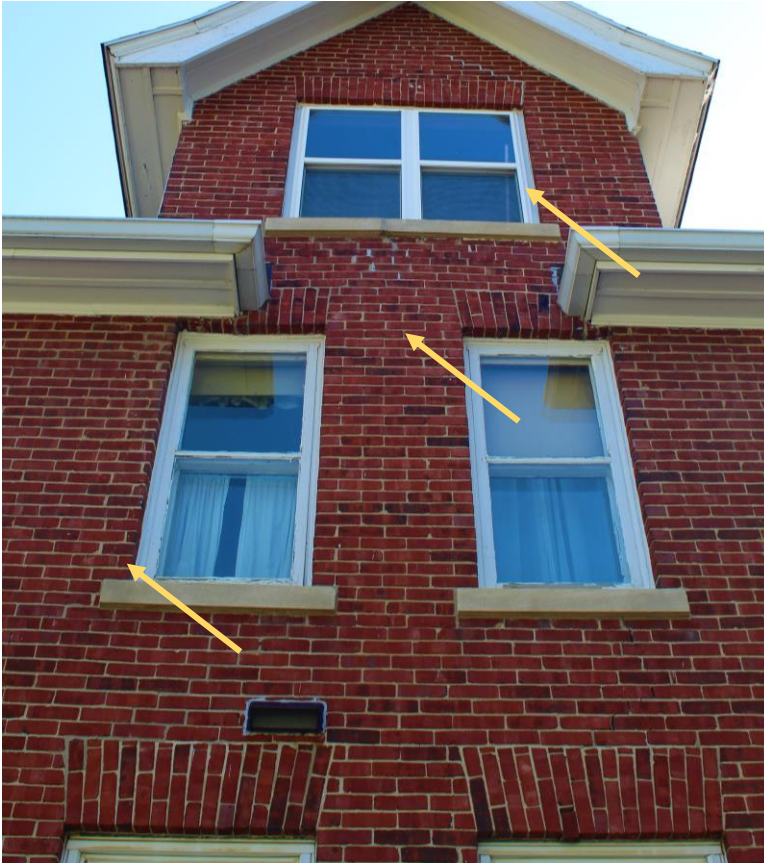
View of the east façade. Note flat brick arches over windows, decorative soffit treatment and original second floor windows. Areas of inappropriate repointing illustrated.
