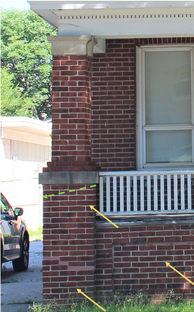
View of southeast corner of front porch. The limestone pier cap has rotated. Evidence of previous repairs of full mortar replacing brick.
