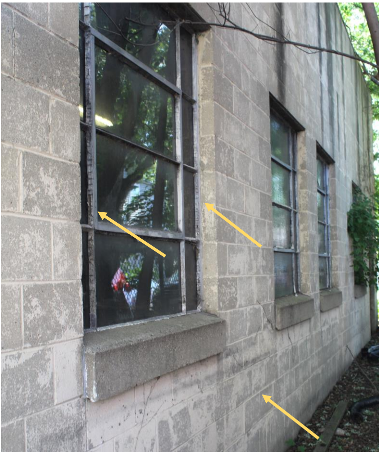
View of the west side of the west addition. Note the deteriorated steel window glazing and paint finish and the paint finish on the concrete block.
