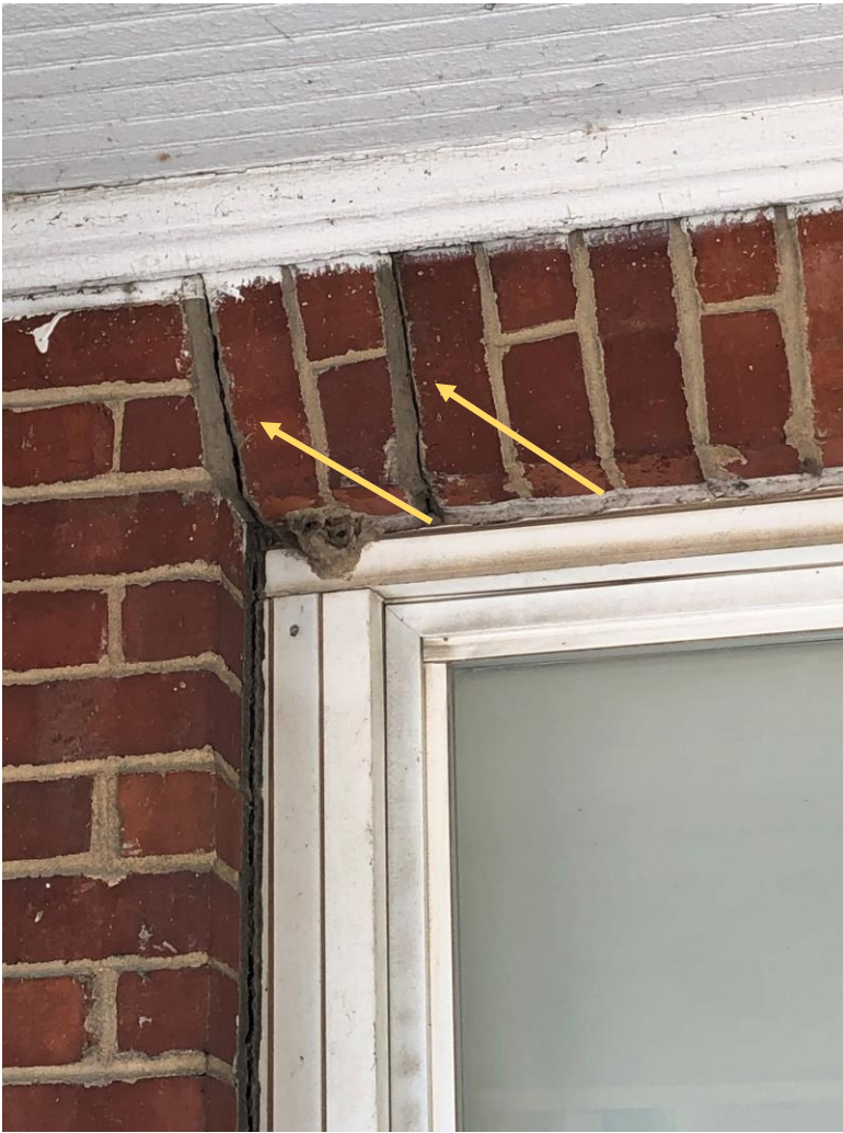
Typical open joints in flat arch over window.
