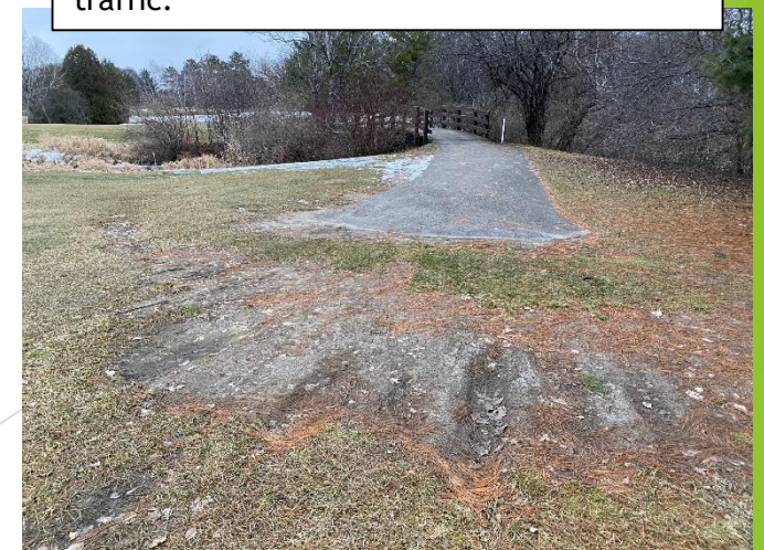
Deteriorating foot bridge and cart path - hole #16 Odana. Wear due to high cart traffic.
