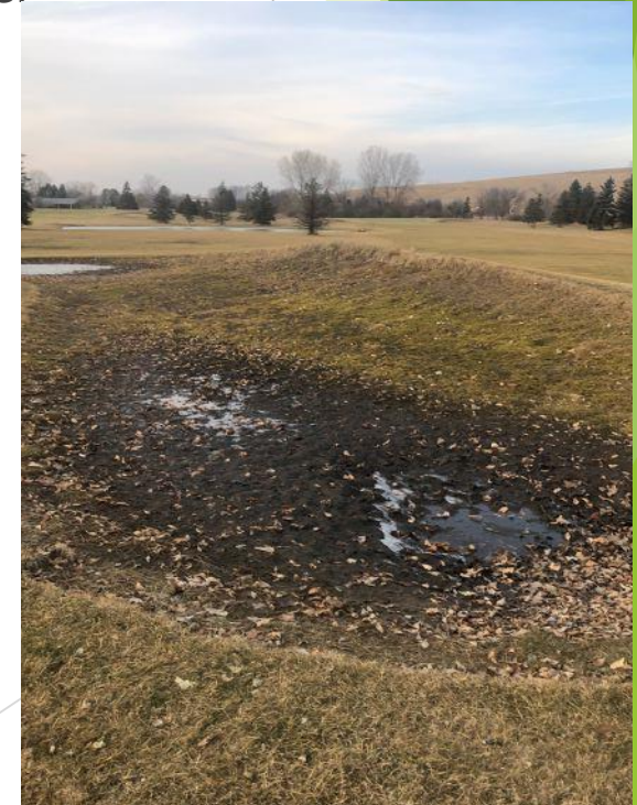
West #12 bunker drainage collapse, resulting in compaction, poor drainage and excessive weed growth.
