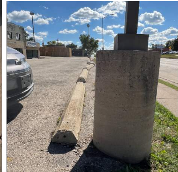
LOT LIGHTING PIERS
