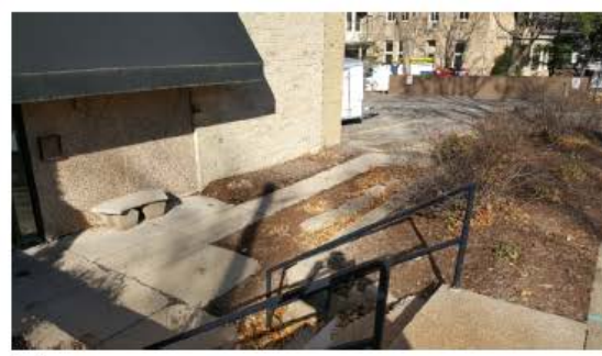
2 SCOPE OF WORK IN PHOTOS 1 - 2 - 3: REPLACE GLASS ENTRY OF BUILDING LOBBY - ADD NEW WINDOW TO LEFT OF DOOR. REMOVE EXISTING AWNING AND REBUILD ORIGINAL CANOPY TO ALIGN WITH NEW ENTRY GLASS. REMOVE AND REPLACE EXISTING CONCRETE STEPS AND WALK. REMOVE AND REPLACE EXISTING GARDEN WALLS AND LANDSCAPE.
