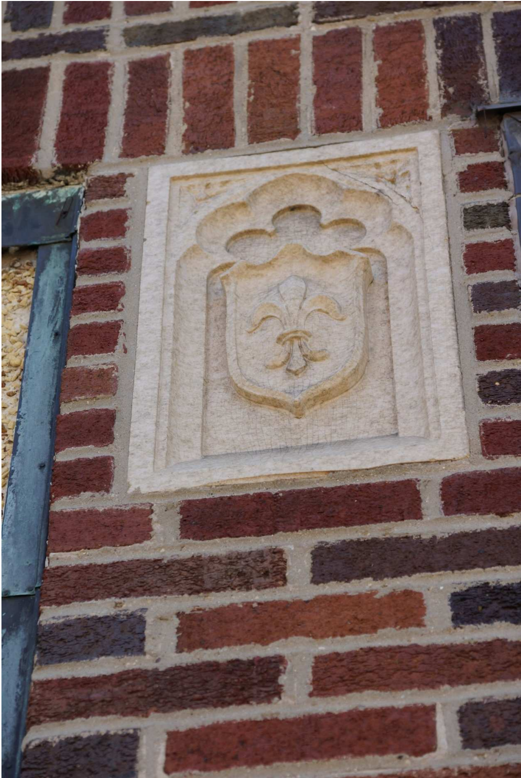
Fig. 19. Cracked corner Stone
