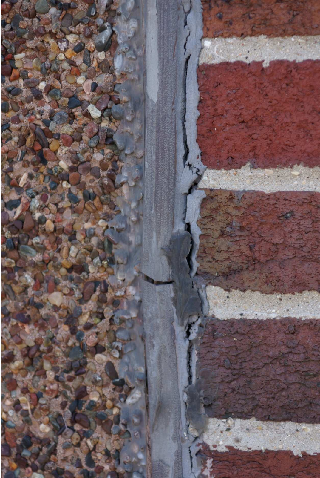
Fig. 17. Crack at flashing and caulk
