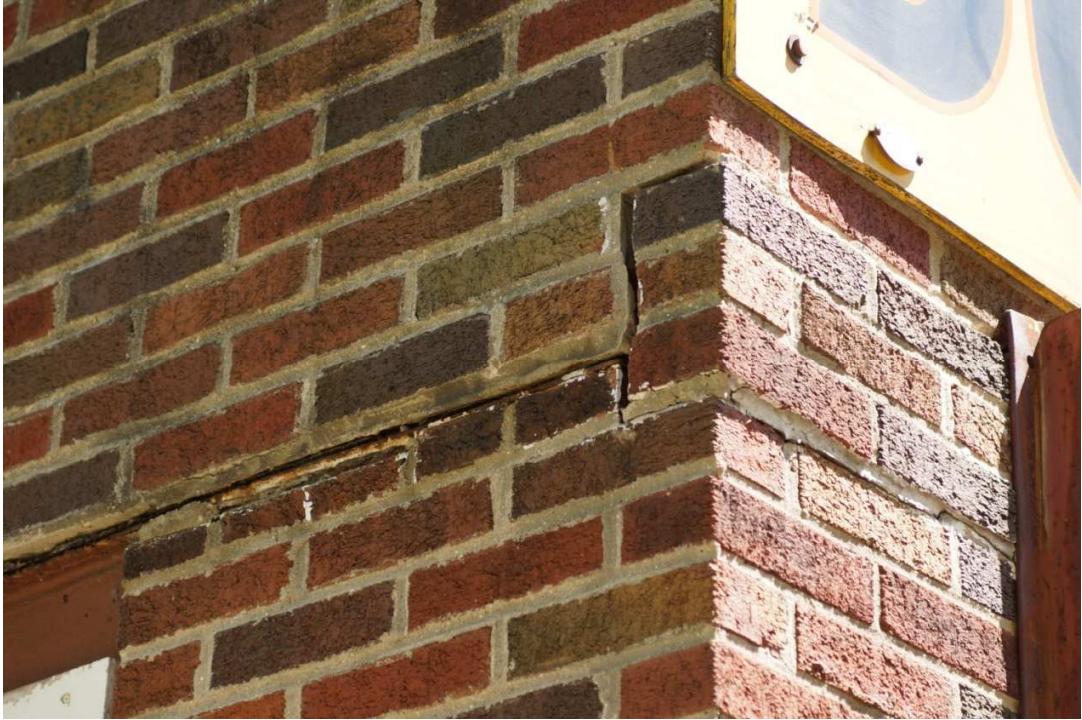
Fig. 11. Displaced brick at the side facade
