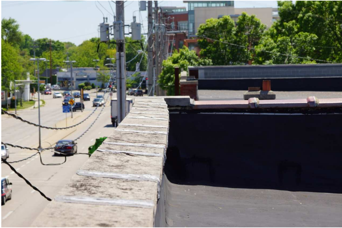
Fig. 5. Front wall displacement
