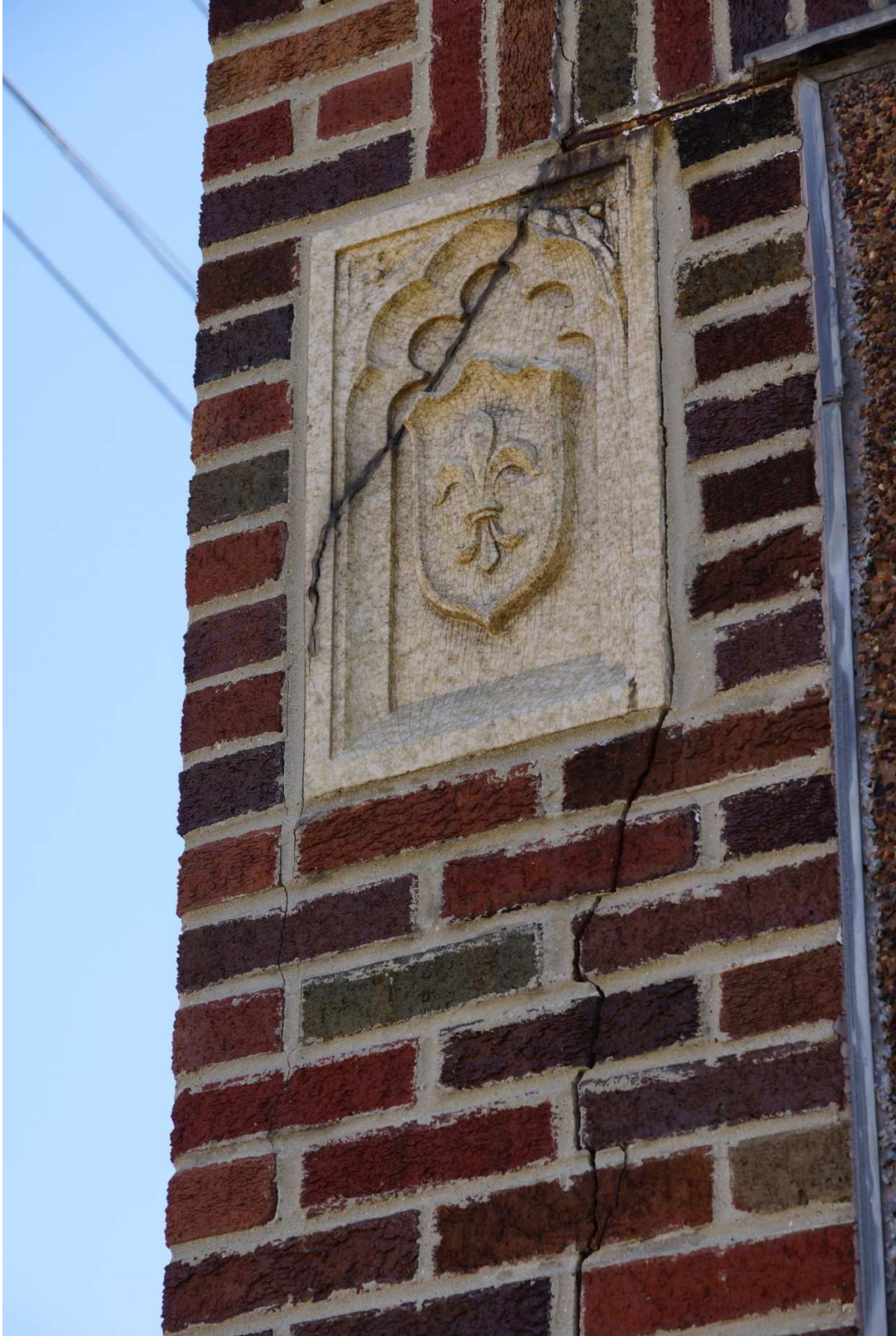
Fig. 15. Cracked corner stone.
