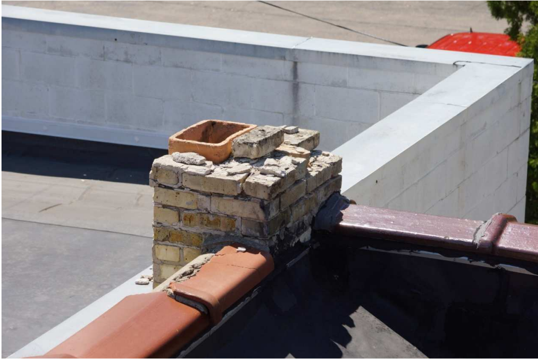
Fig. 7. Deteriorated Chimney Brick
