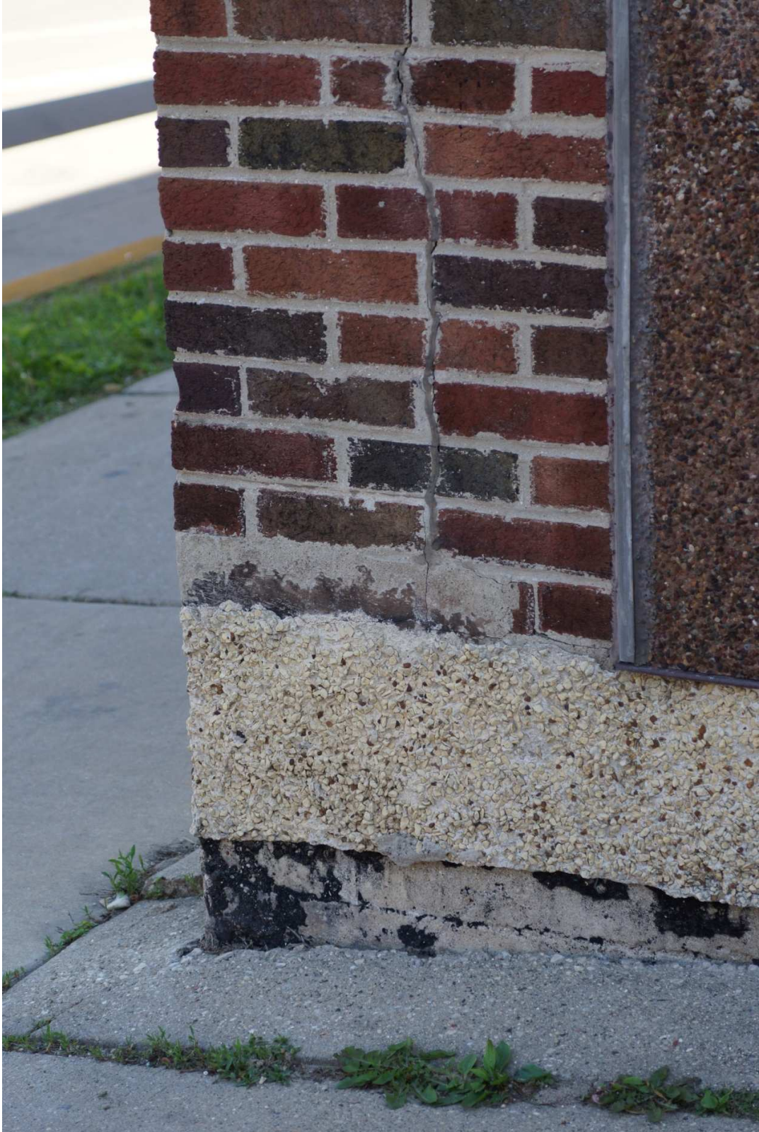
Fig. 16. Vertical wall crack
