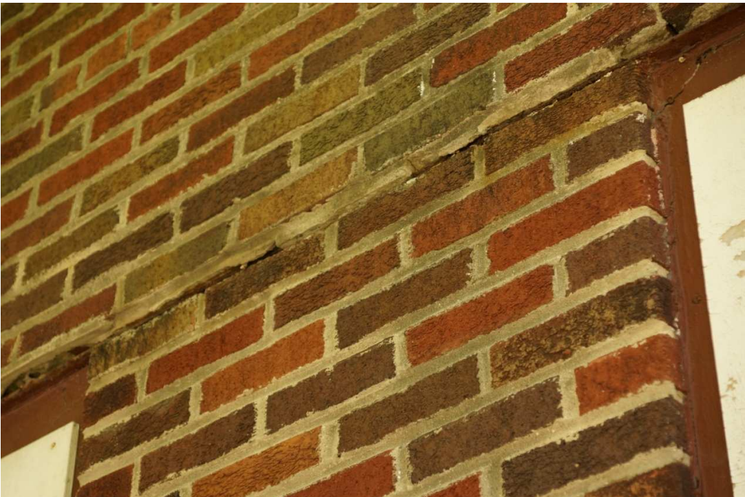
Fig. 12. Cracked mortar joint at the side façade
