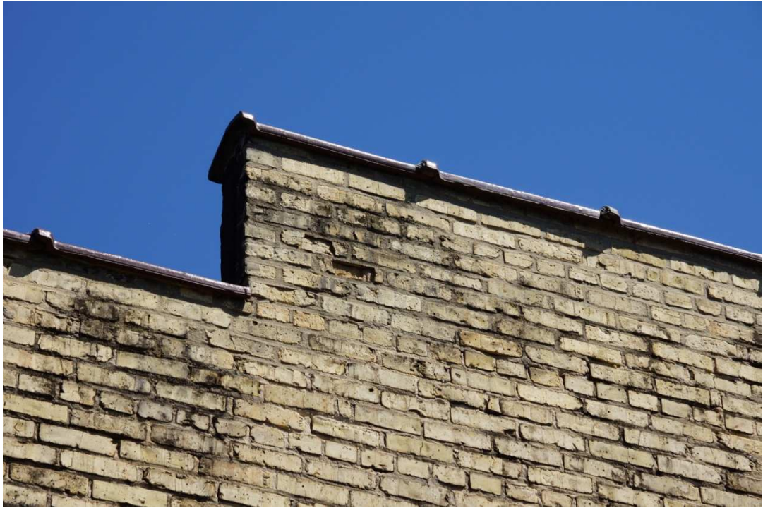
Fig. 9. Deteriorated brick at the back wall
