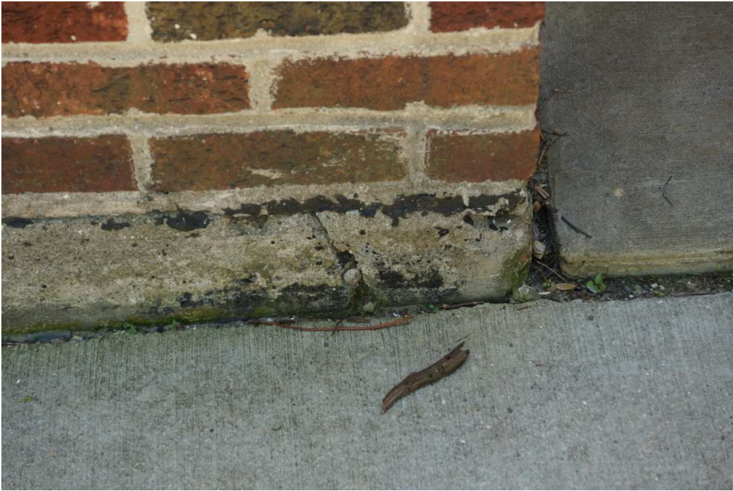
Fig. 13. Cracked foundation wall
