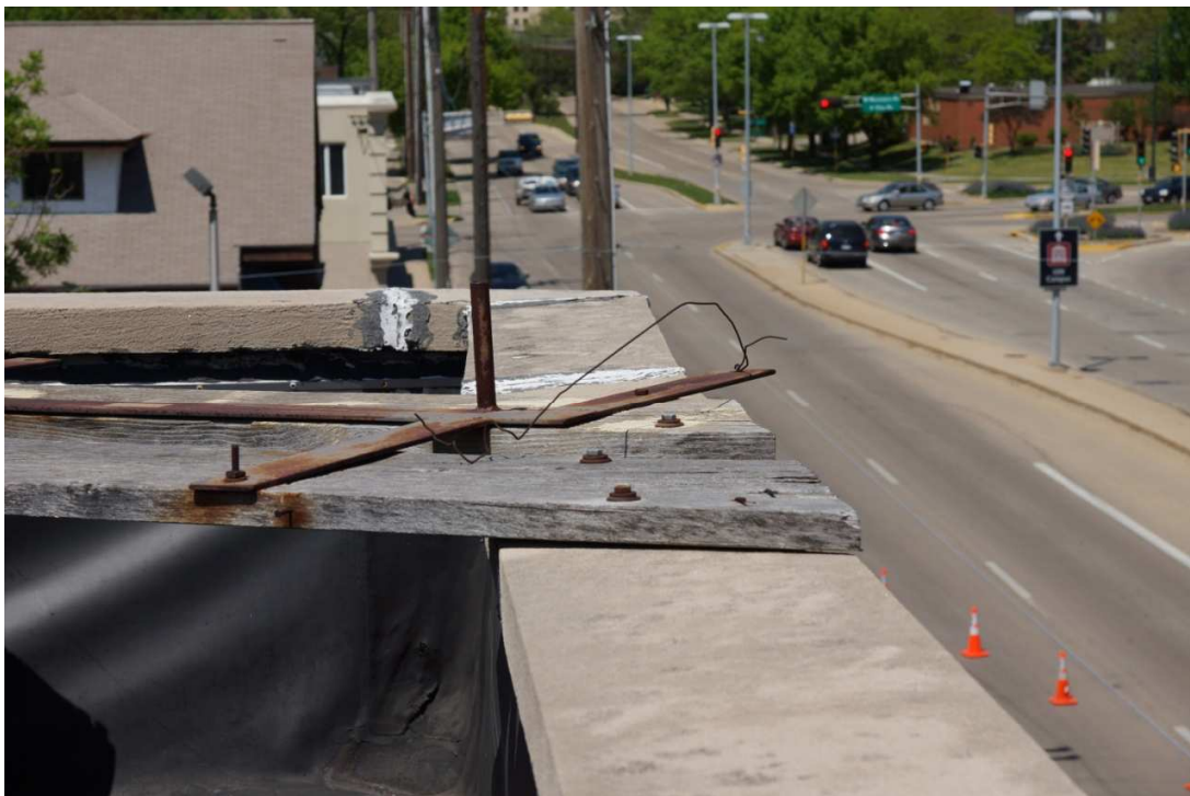
Fig.6. Front wall Displacement
