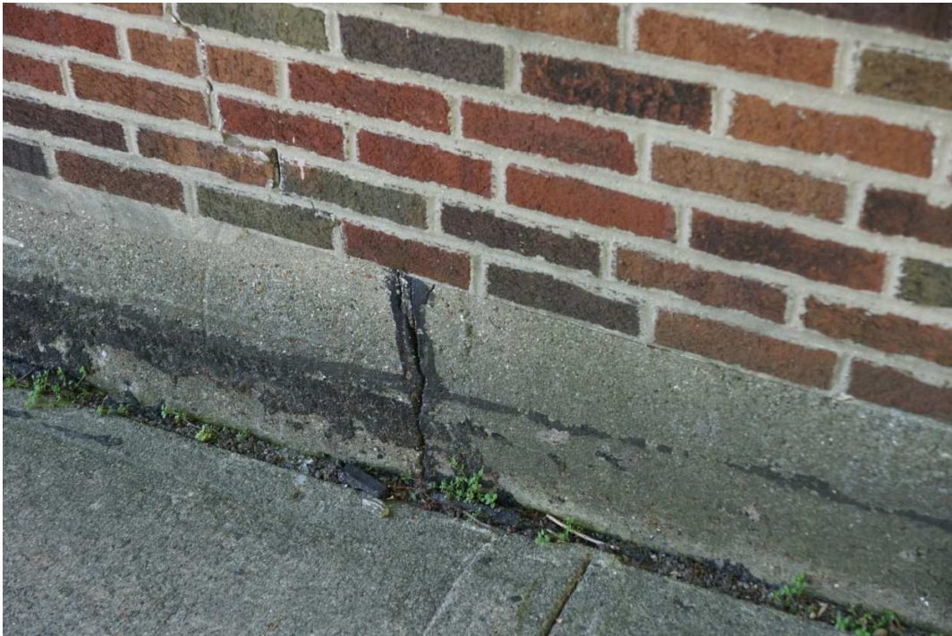
Fig. 14. Cracked foundation wall
