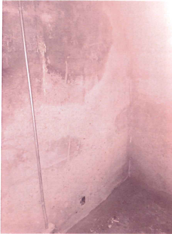
4. South west corner of basement with exposed aggregate and deteriorating cement.
