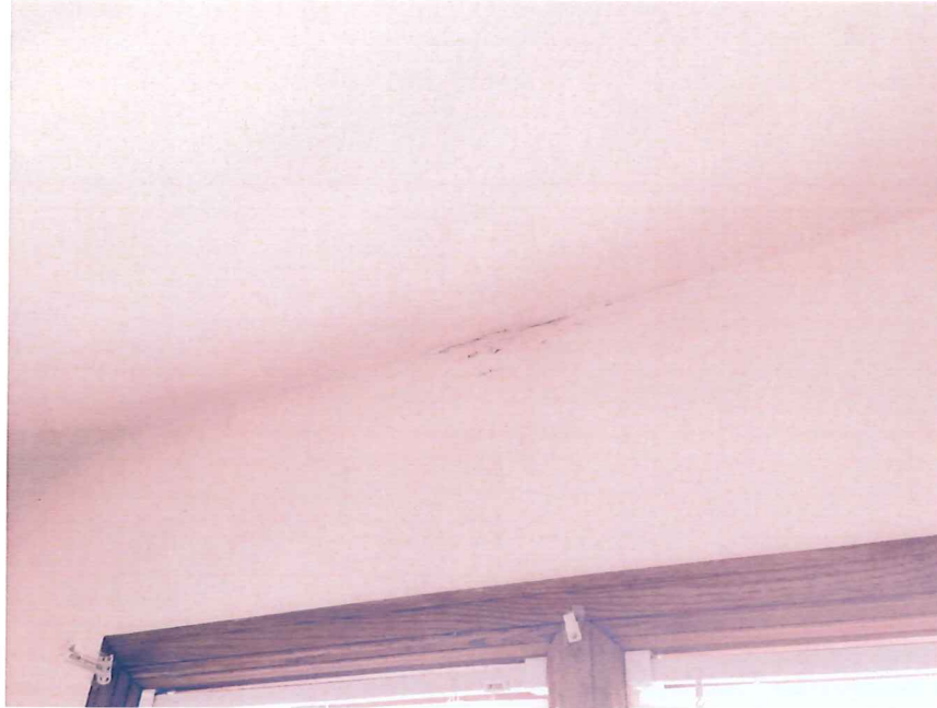
6. Water damage at interior ceiling. 7.
