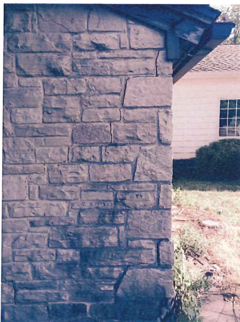
3. Diagonal crack at back corner of garage due to settling of foundation.
