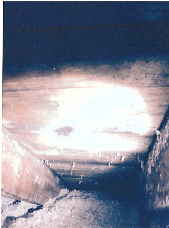
8. Evidence of mold on roof deck and joists in attic.
