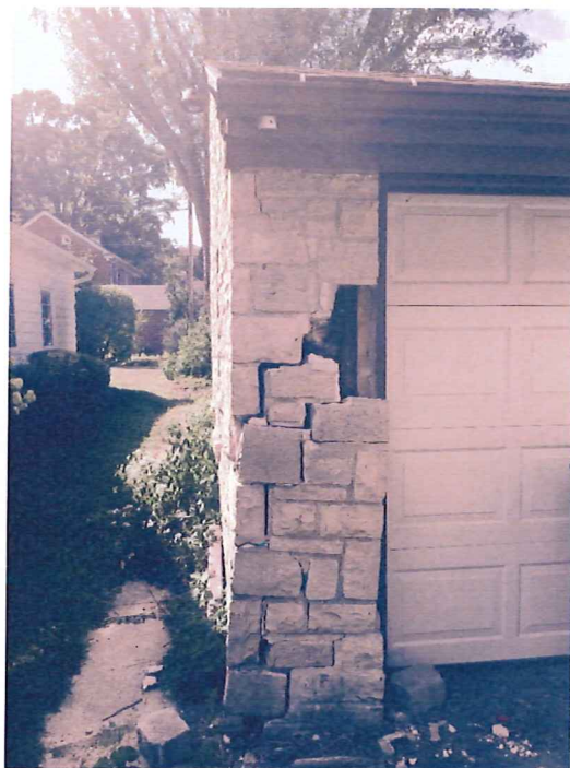
2. Exterior stone settling and falling off front corner of garage.
