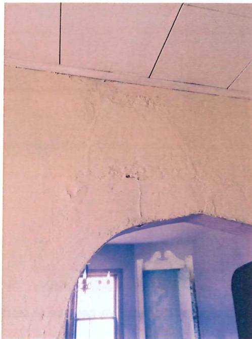
5. Interior water damage at first floor arch.
