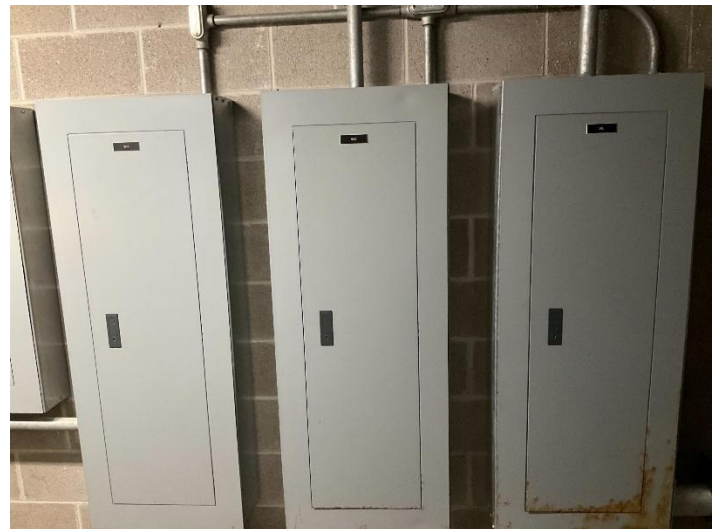
Existing Electrical Controls to be Replaced
