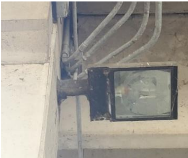
Existing RR Luminaires to be Replaced
