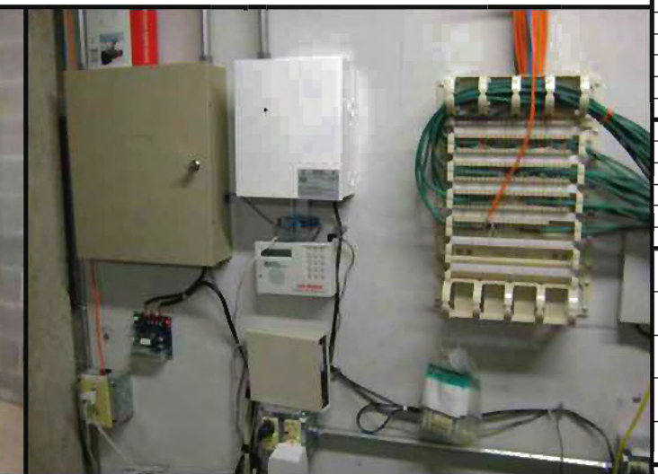
EXISTING TELCO BOARD IN UTILITY ROOM
