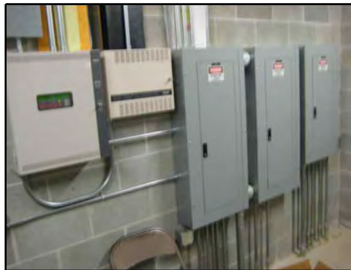
EXISTING AC ELECTRIC PANELS IN UTILITY ROOM
