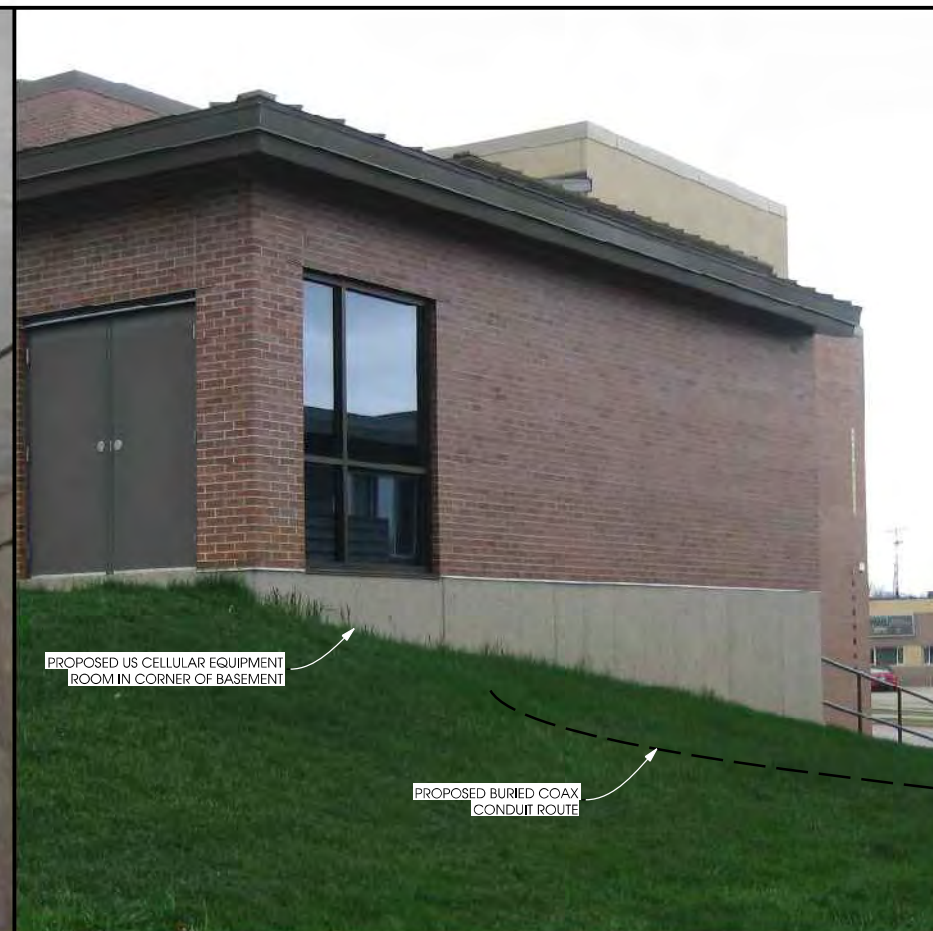
OUTSIDE EQUIPMENT ROOM
