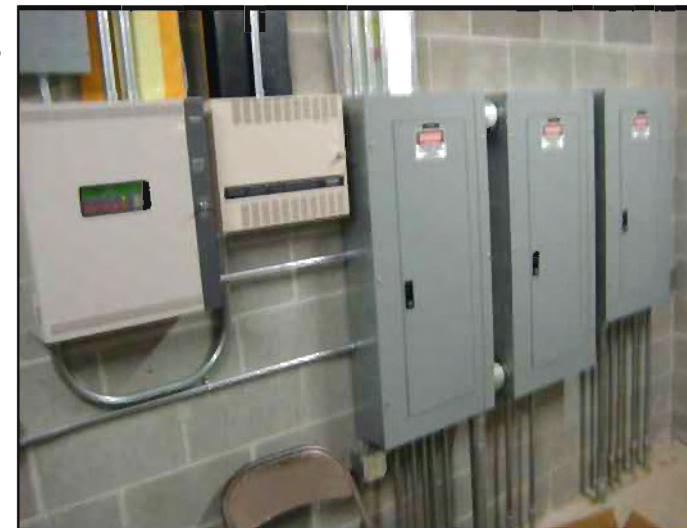
EXISTING AC ELECTRIC PANELS IN UTILITY ROOM
