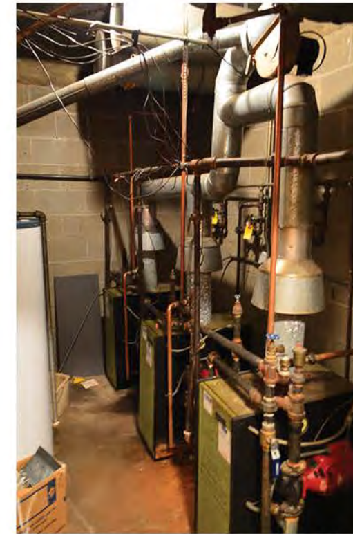
Mechanical room within original building
