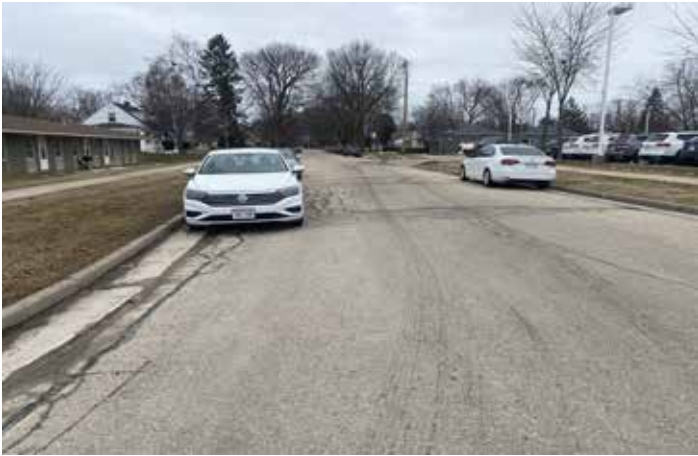
Concord Rd, near N Stoughton Rd (fair condition, crack)
