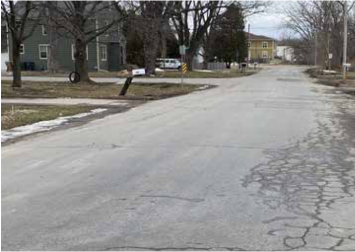
Rowland Ave (fair condition, crack, pothole)
