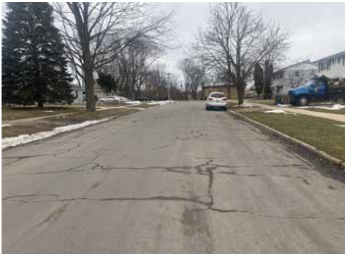
Prairie Av, near N Stoughton Rd, (good condition, but minor cracking)
