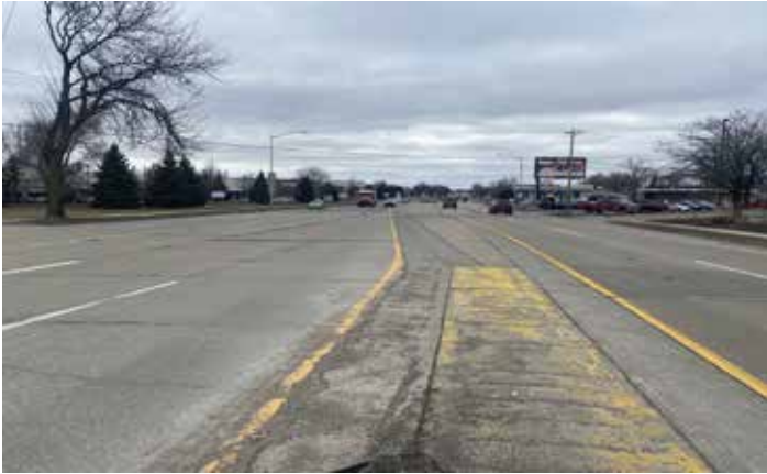
N Stoughton Rd, (fair to good condition, some cracking)
