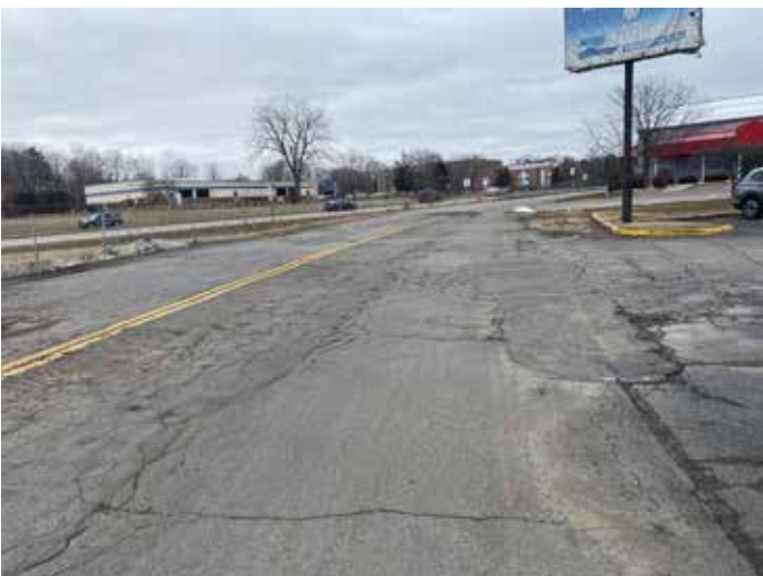
N Stoughton Rd, Service Rd, (fair condition, crack, uneven surfaces)
