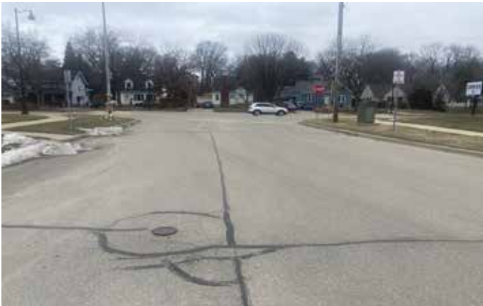
Lexington Ave, off E Washington Ave ( good condition )
