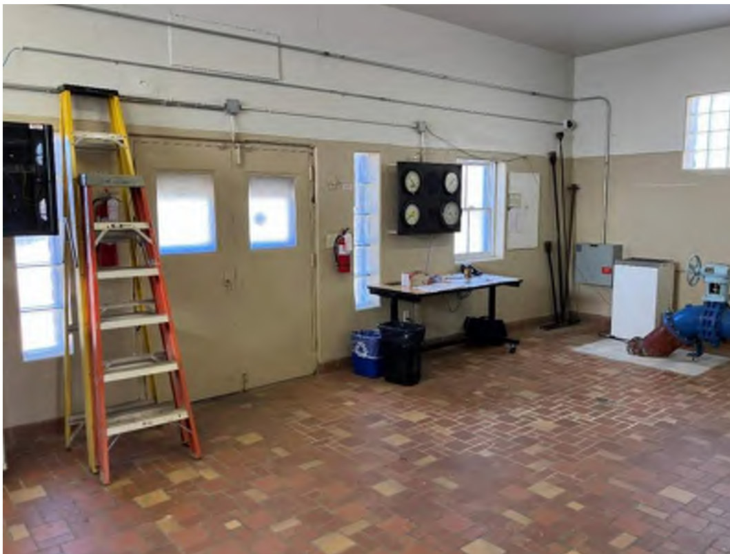
Interior of existing Wellhouse.
