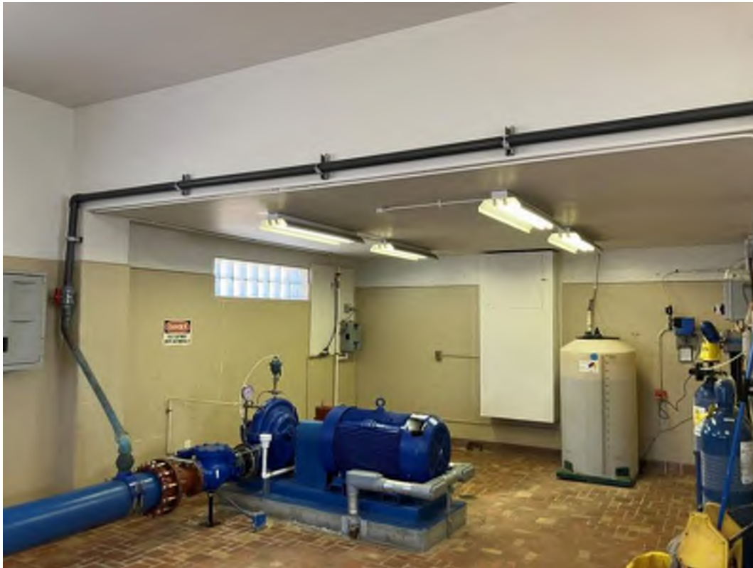
Interior of existing Wellhouse.
