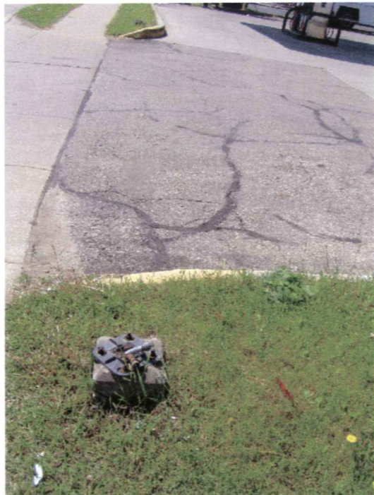
2200 South Park Street Obsolete sign base and cracked driveway May 25, 2003
