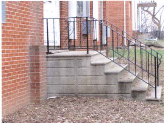
2306 Badger Parkway Uneven porch October 25, 2003
