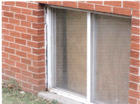
2306 Badger Parkway Deteriorated window frame October 25, 2003
