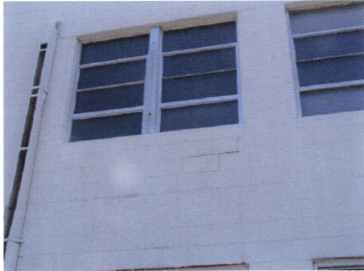
2216 South Park Street Cracked Wall May 25, 2003
