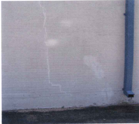
1818 South Park St Cracked Wall October 25, 2003
