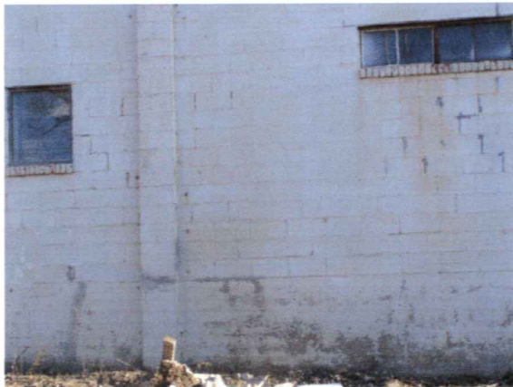
1818 South Park Street Cracked wall and foundation October 25, 2003
