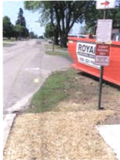
Perry Street Missing Sidewalk July 7, 2005
