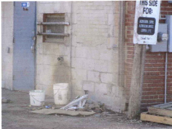
1818 South Park Street Trash and cracked wall, deteriorated door and window October 25, 2003
