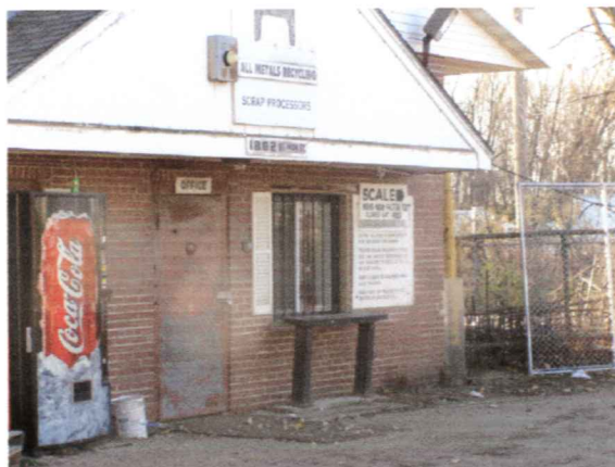
1818 South Park Street Deteriorated door October 25, 2003
