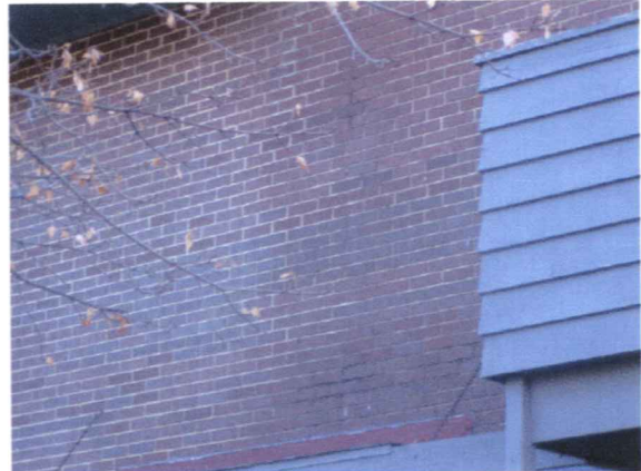
1850 Beld Street Cracked wall with water damage October 25, 2003
