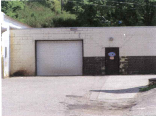
2431 South Park Street Cracked wall, blighted parking lot May 25, 2003
