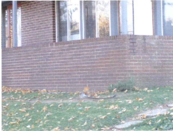
1850 Beld Street Cracked wall October 25, 2003
