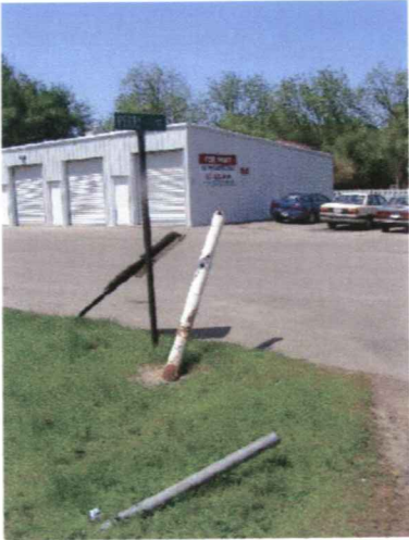
2505 South Perry St Bent Posts May 25, 2003
