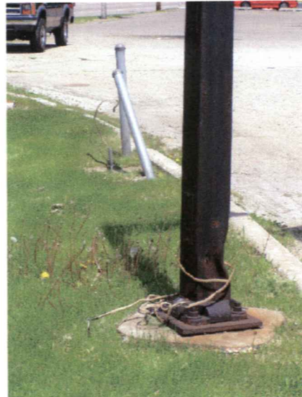
2421 South Park Street Exposed wiring, bent and dented posts May 25, 2003
