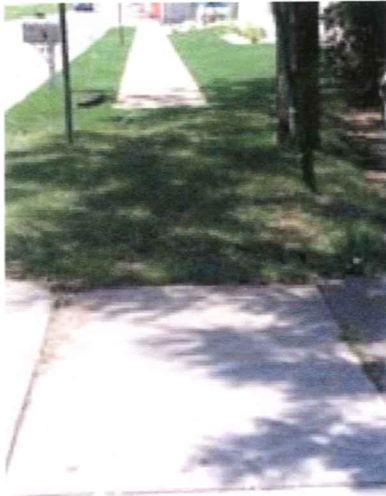
Perry Street Missing Sidewalk July 7, 2005
