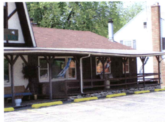
2465 South Perry Street Sagging Roof May 25, 2003
