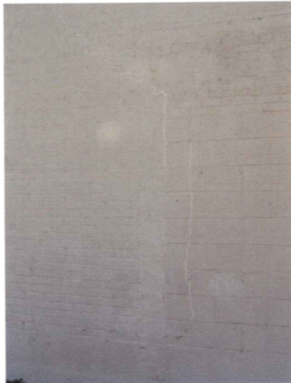
1818 South Park St Cracked Wall October 25, 2003
