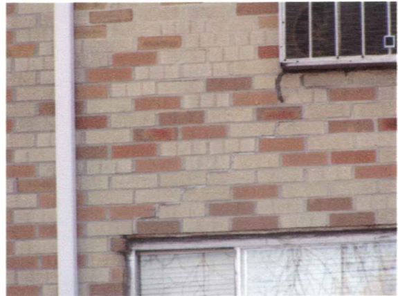
1114 Ann Street Cracked Wall October 25, 2003
