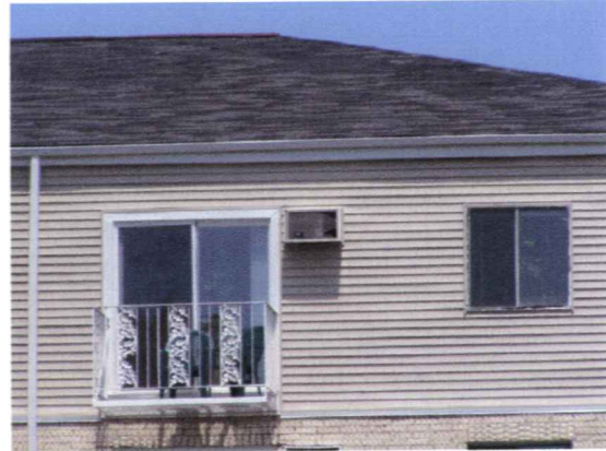
700 West Badger Road Deteriorated roof and window frame May 25, 2003
