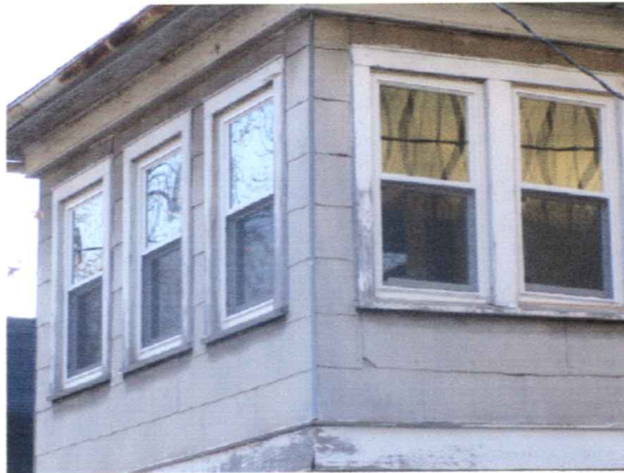
1810 Beld Street Deteriorated windows October 25, 2003
