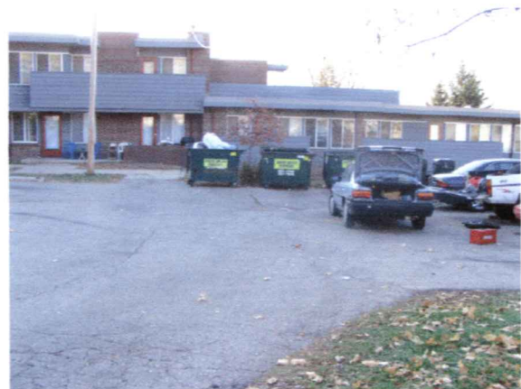
1850 Beld Street Cracked drive, unscreened trash containers October 25, 2003
