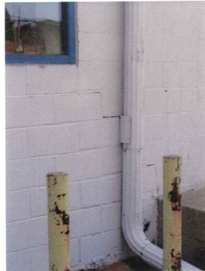
2216 South Park St Cracked Wall May 25, 2003
