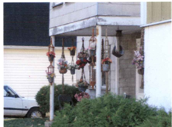
1810 Beld Street Rotted porch October 25, 2003
