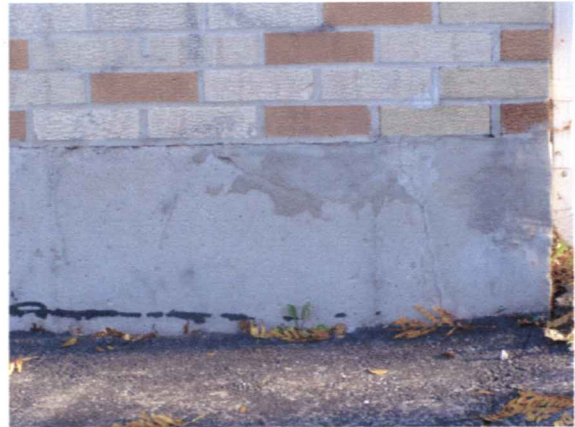
1114 Ann Street Cracked foundation October 25, 2003
