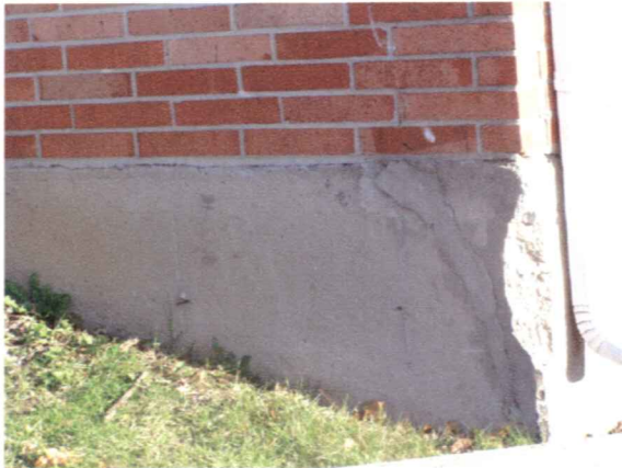
1114 Ann Street Cracked foundation October 25, 2003
