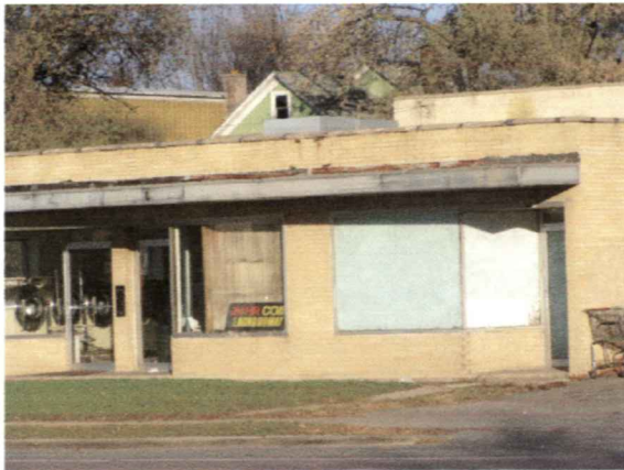
1817 South Park Street Deteriorated roof October 25, 2003
