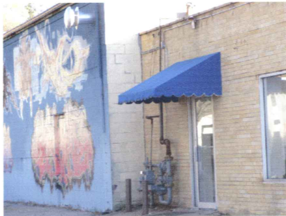
1817 South Park Street Cracked wall October 25, 2003
