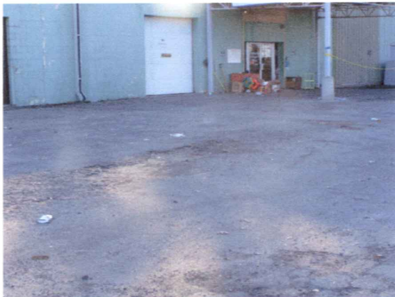
1500 South Park Street Deteriorated drive October 25, 2003
