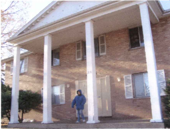
1114 Ann Street Deteriorated porch posts October 25, 2003
