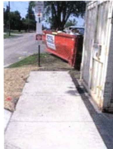
Missing Sidewalk Perry Street July 7, 2005
