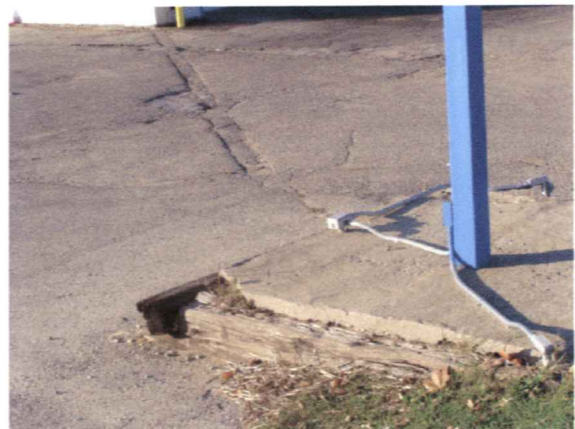
1824 South Park Street Deteriorated sign base October 25, 2003
