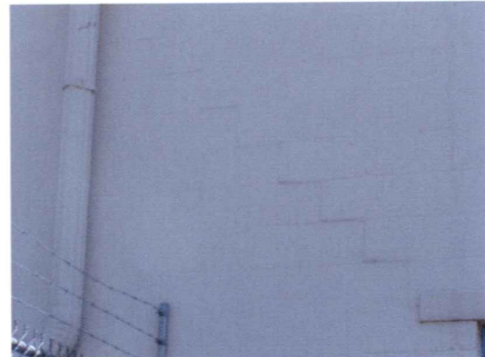
1818 South Park Street Cracked Wall October 25, 2003
