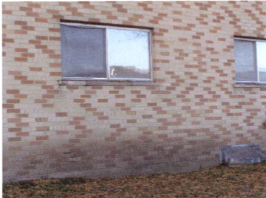
1114 Ann Street Water damaged wall October 25, 2003
