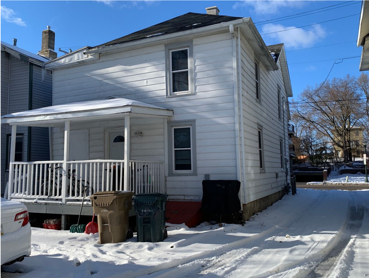
Photo 2 633 East Johnson Street, SE (rear) and NE facades Photographer: Elizabeth L. Miller Date: December 20, 2024
