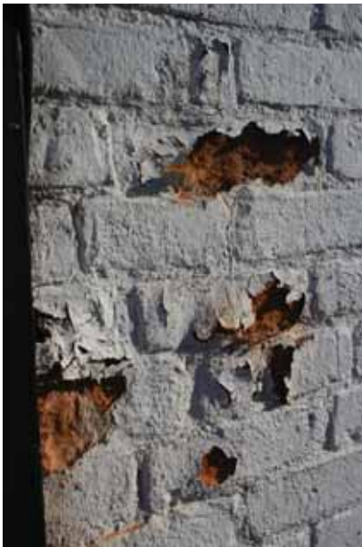
Exterior: View of damaged brick veneer
