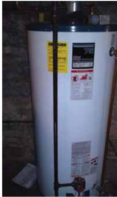
New water heater
