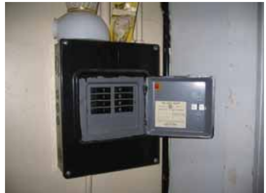
Electrical panel on 2 nd floor.
