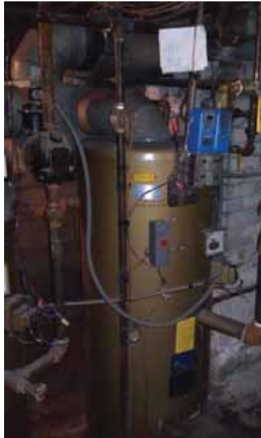
Hot water boiler
