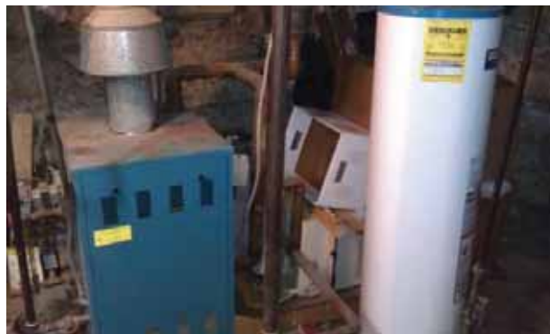
Hot water boiler and water heater
