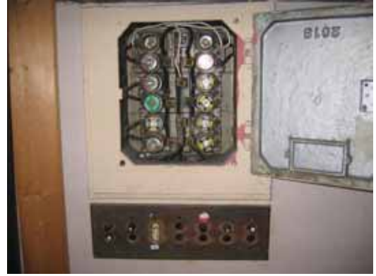
Electrical fuse panel on 1 st floor.
