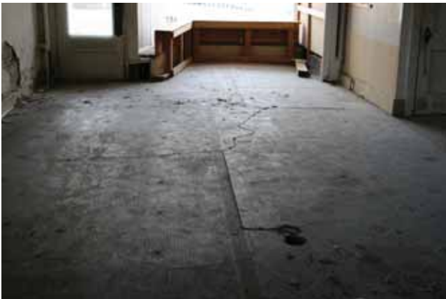
First Floor: View toward Mifflin Street entry showing multiple cracks in floor tiles
