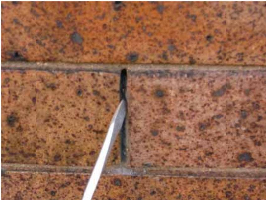
Figure 4. Occasional open mortar joints were observed.
