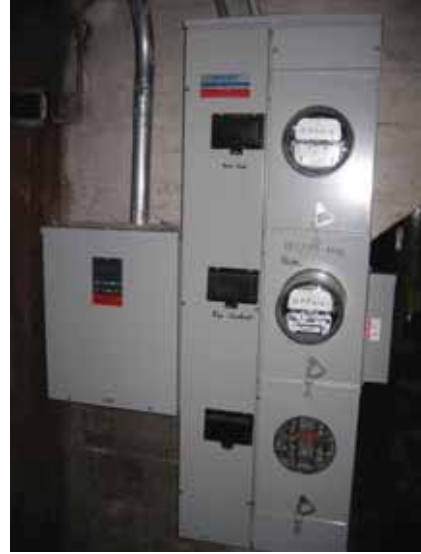
The newer electrical meters in the Basement.
