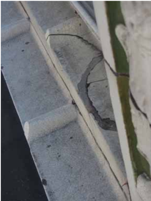
Figure 3. One cracked terra cotta window sill.
