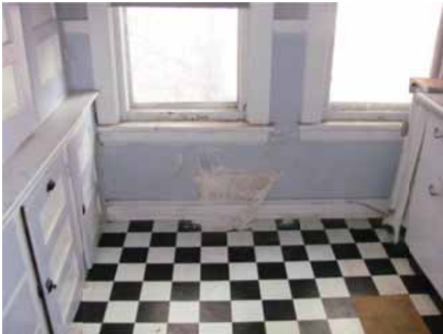
Figure 18. Plaster damage at the rear wall at the second floor of the building.
