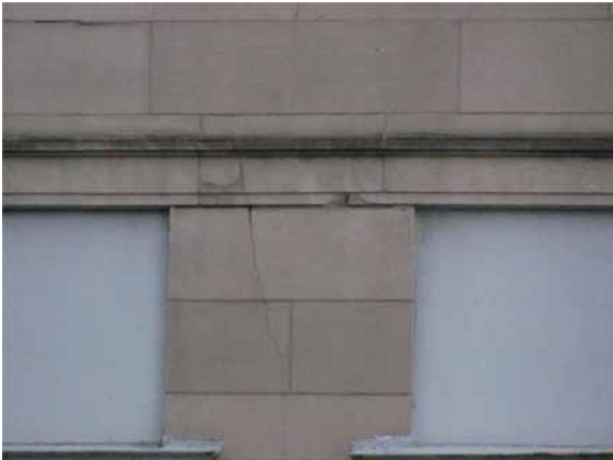
Figure 5. Cracking and spalling of limestone masonry at the head of a first floor window opening.
