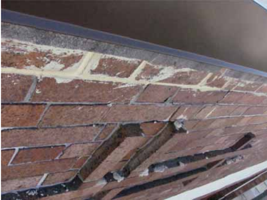
Figure 3. Portions of the top of the parapet wall were previously repointed.
