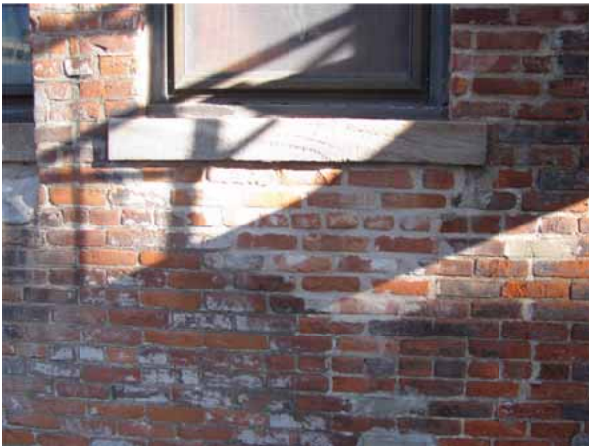
Figure 12. Localized areas of brick masonry appear to have been rebuilt previously.
