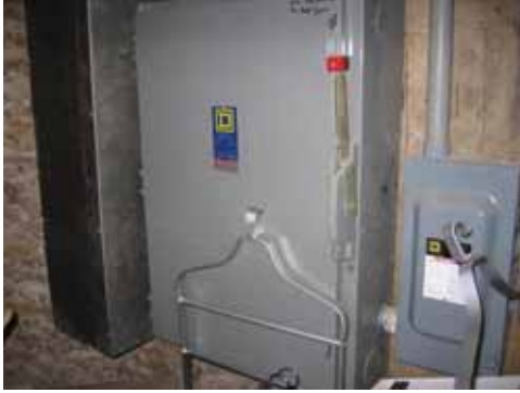
Building main disconnect.
