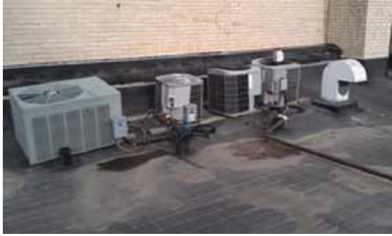
Condensing units serving the furnaces
