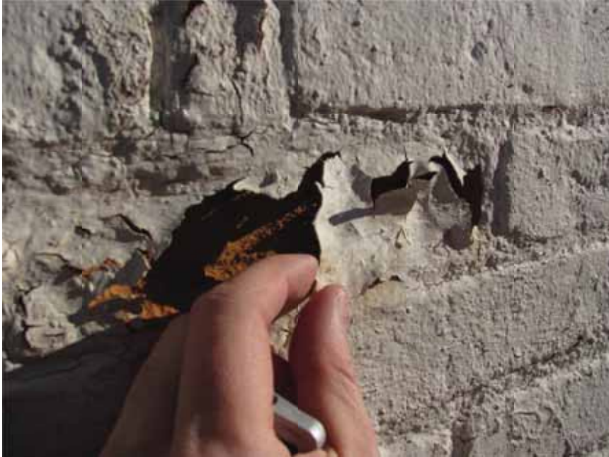
Figure 3. Loss of the coating reveals severely deteriorated brick units.
