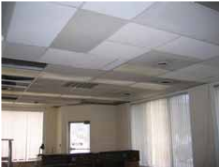
First floor lights.
