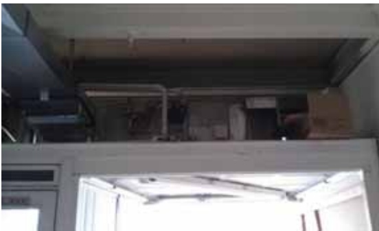
Furnace above entrance
