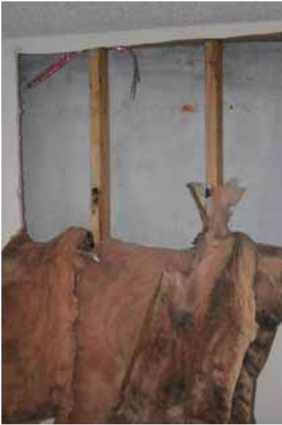
Third Floor: Section of exterior wall exposed showing back of brick and moisture within the insulation space
