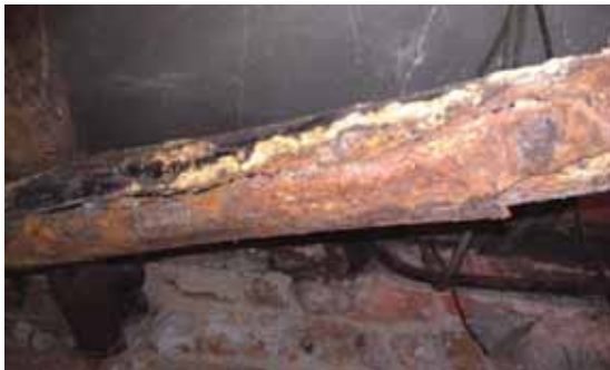
Deteriorated sanitary pipe
