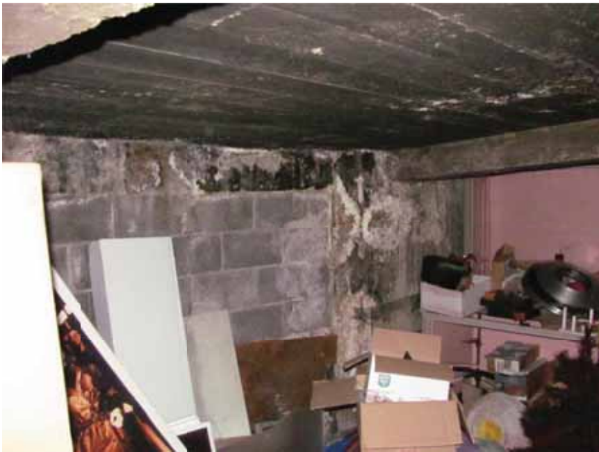
Figure 22. Efflorescence and water staining at the basement level below the entrance storefront.
