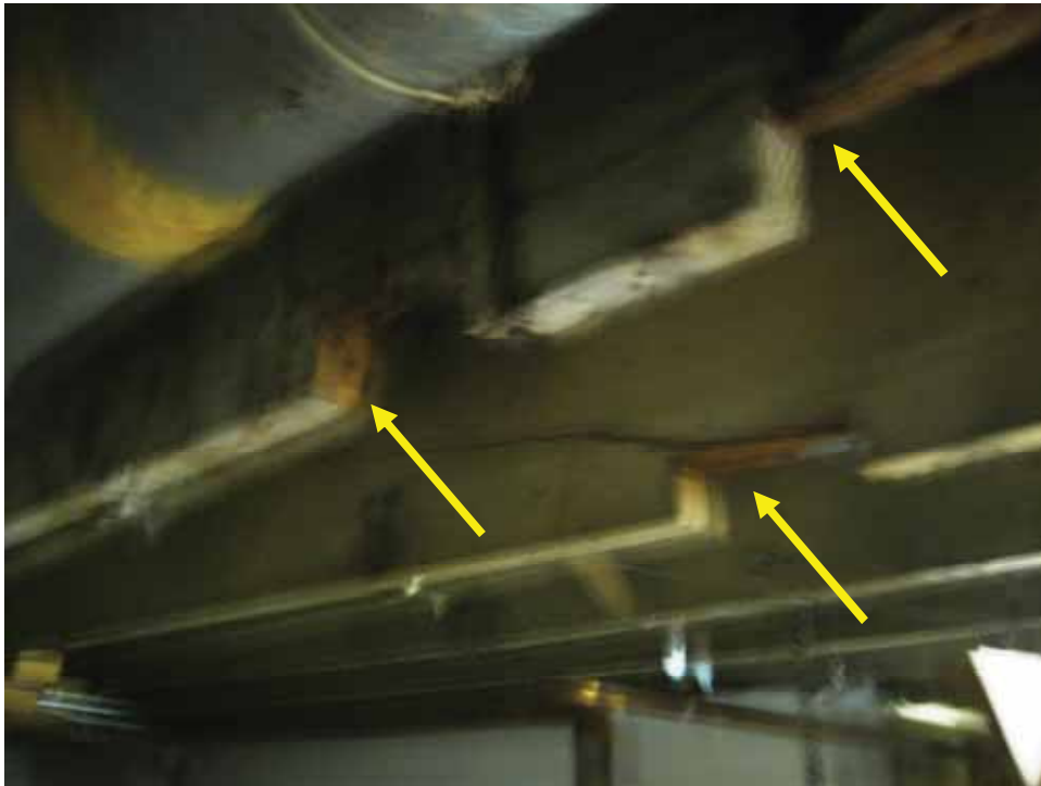
Photo 6 – Notched 1 st floor joists
