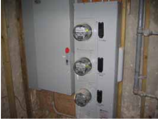
Electrical service in the basement.
