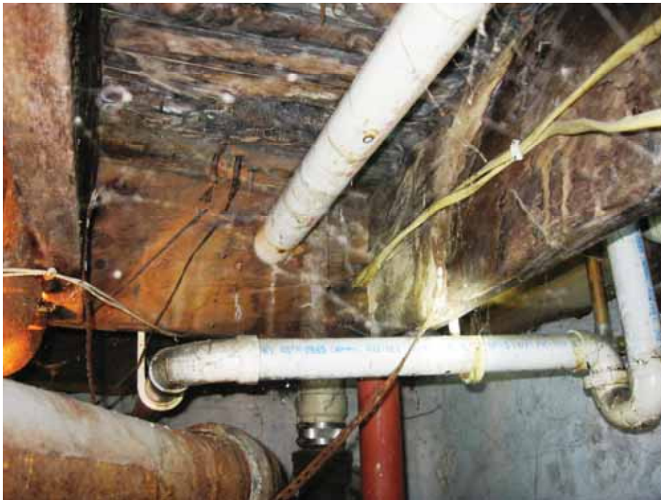
Photo 7 – 1 st floor framing with water damage
