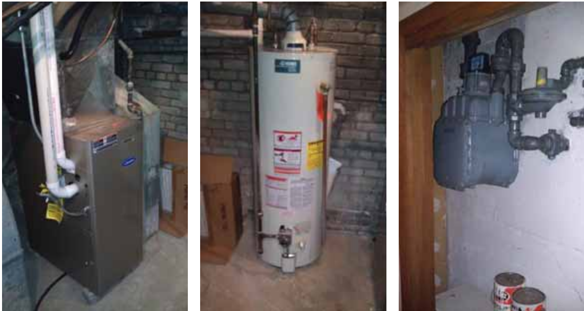
One of four identical furnaces, the water heater, and gas meter
