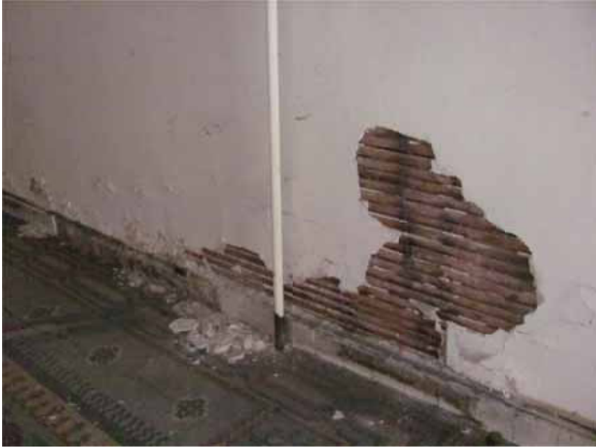
Figure 15. Damage to interior plaster wall finish.
