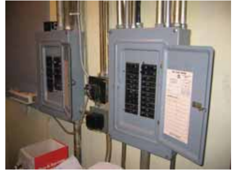
Electrical panels on 2 nd floor.
