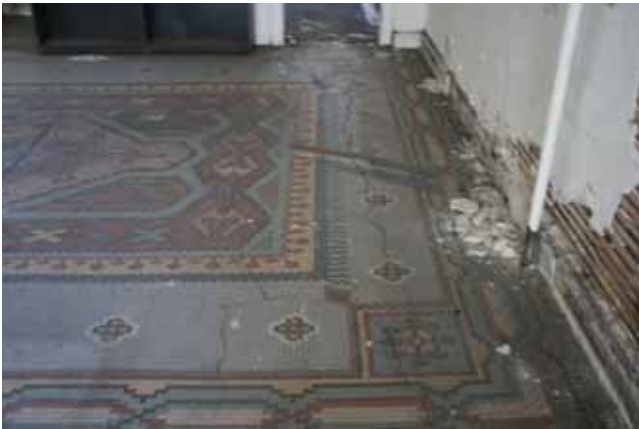
First Floor: View toward back exit showing multiple cracks in floor tile
