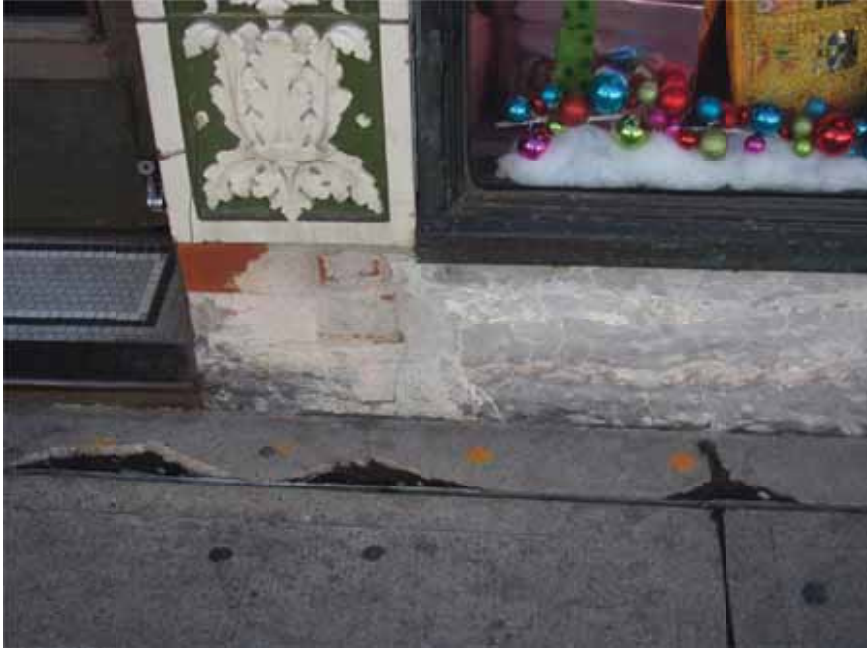
Figure 2. Marbleized cast stone and brick masonry at the base of the State Street facade.
