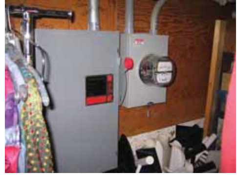
Basement electrical meter and disconnect.
