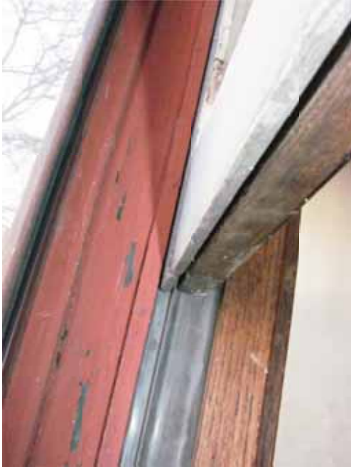
Figure 9. The original wood windows appeared intact and have been routed to receive galvanized metal weatherstripping.
