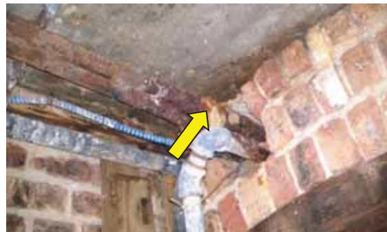
Deteriorated gas pipe
