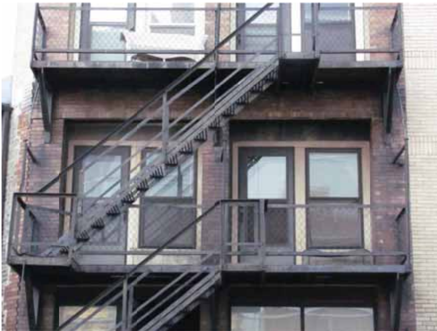
Figure 12. The balconies and fire escapes appeared intact, with areas of paint loss and surface corrosion.
