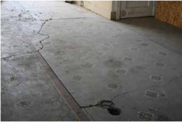
First Floor: View toward basement stair showing multiple cracks in tile floor
