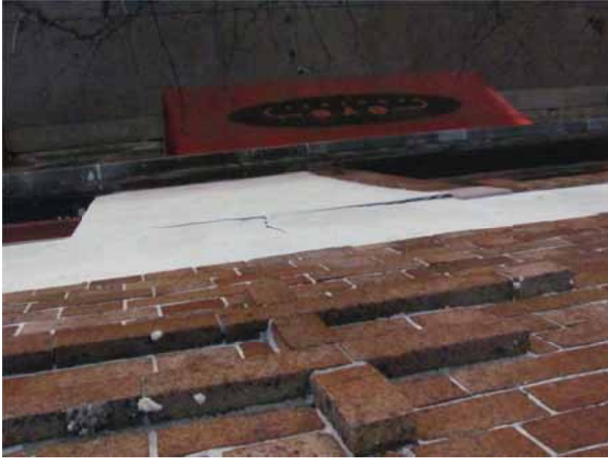
Figure 5. View from the roof of one especially large delaminated area of stucco observed near the middle of the facade.
