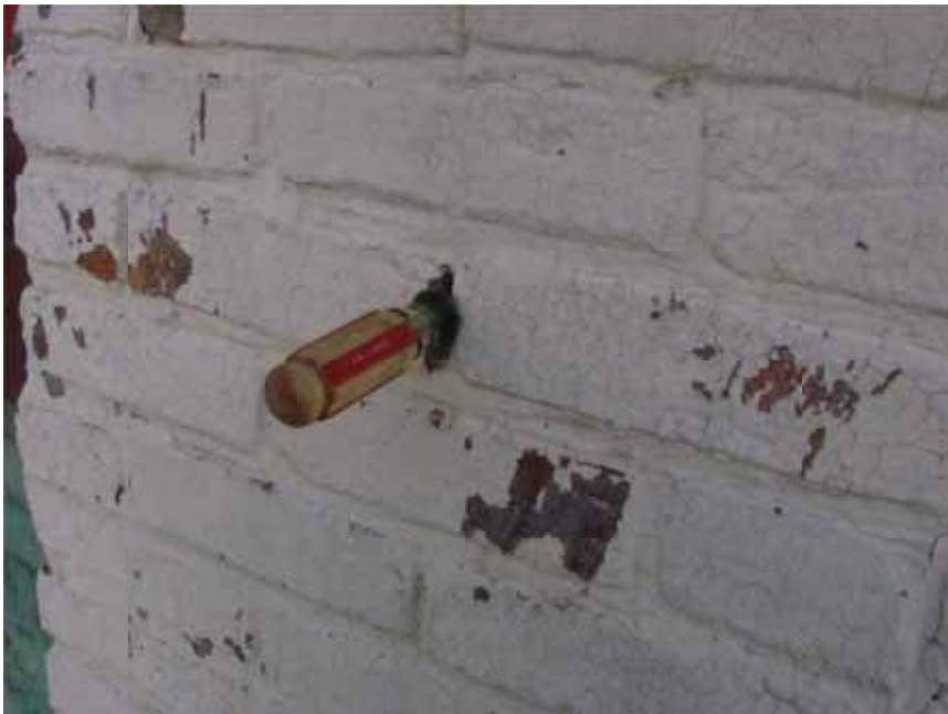
Figure 6. Mortar behind the coating layers has disintegrated, resulting in voids within the masonry construction.
