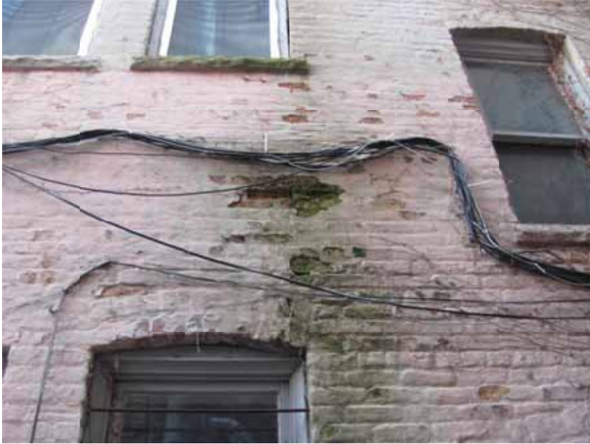
Figure 6. Deterioration of brick masonry at the rear facade.
