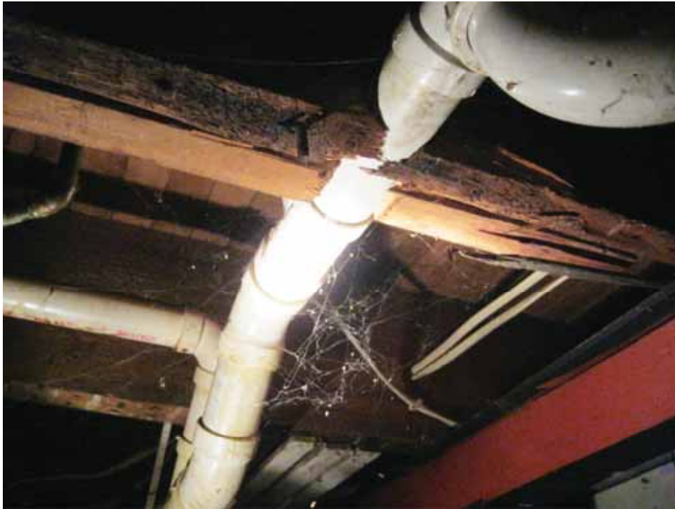
Photo 8 – 1 st floor framing notched for plumbing
