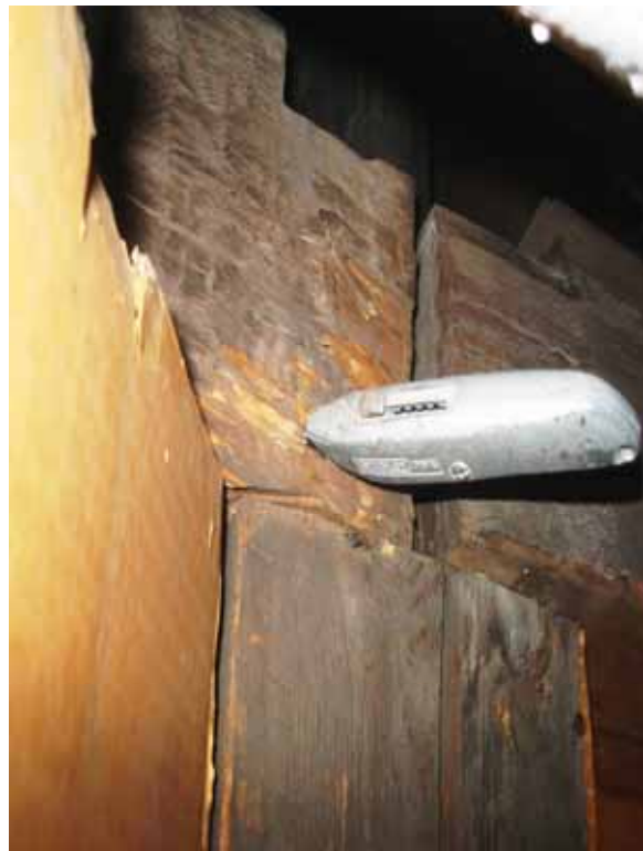
Photo 2 – Poor fit up and wood density at 1 st floor beams and column
