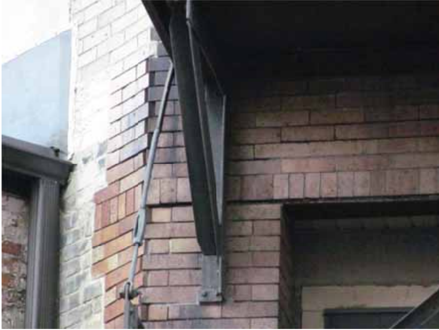
Figure 13. Surface corrosion and minor displacement of masonry associated with the bearing points of the lintels was observed.
