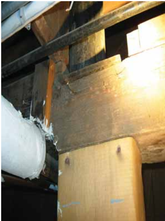
Photo 1 – Notched 1 st floor beam requiring replacement
