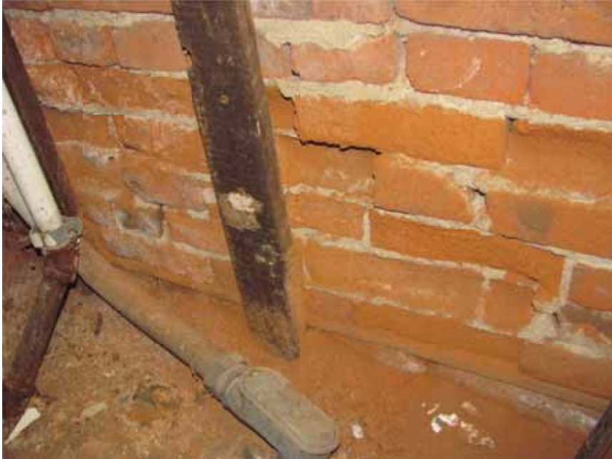
Figure 7. Deterioration of the back-up masonry at the interior of the building.
