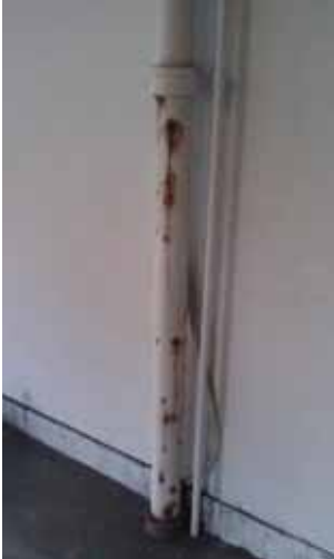
Leaking sanitary pipe
