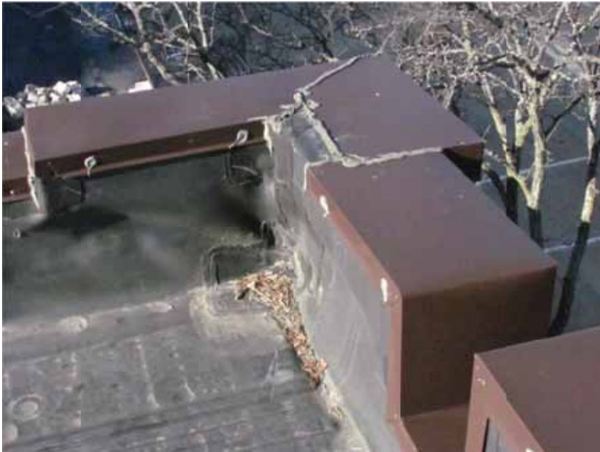
Figure 16. The sheet metal coping has numerous laps and splices that are surface-sealed with untooled sealant.
