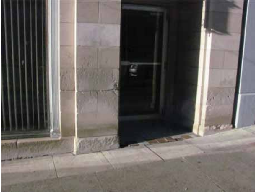
Figure 4. Portions of the limestone masonry near grade exhibit erosion and pitting of the face.
