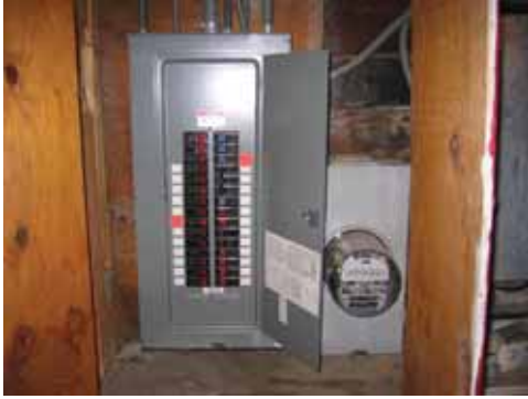
Part of the electrical service in a constructed cabinet.
