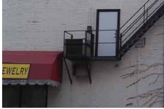
Apartment condensing unit
