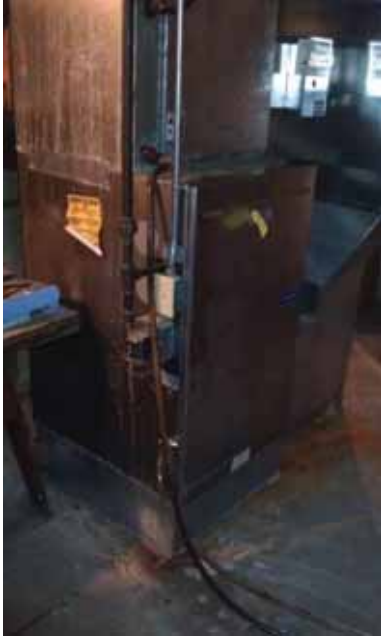
First floor furnace
