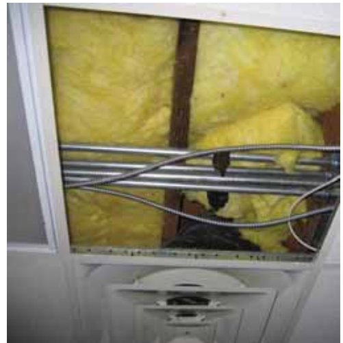
Conduits above ceiling on 3 rd floor.
