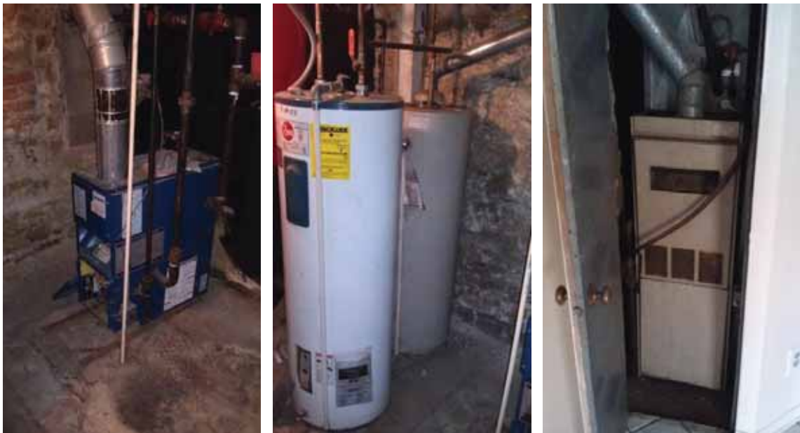
Boilers, water heaters, and furnace
