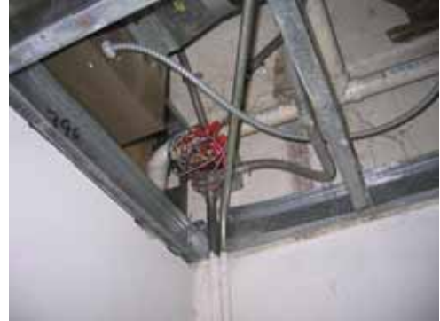
Wiring in 129 State Street.
