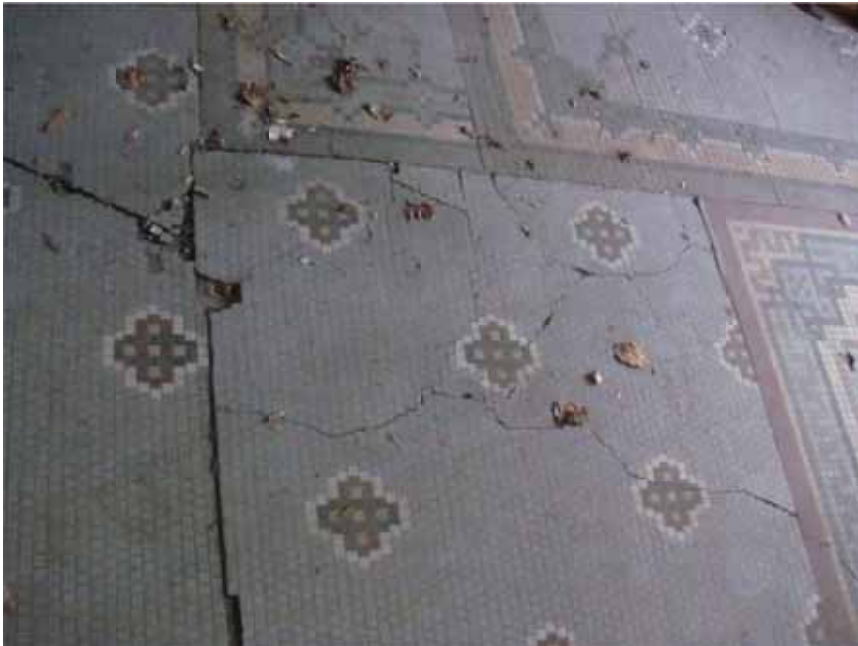
Figure 14. There is elaborate mosaic tile flooring at the first floor; the flooring has suffered extensive cracking and displacement.
