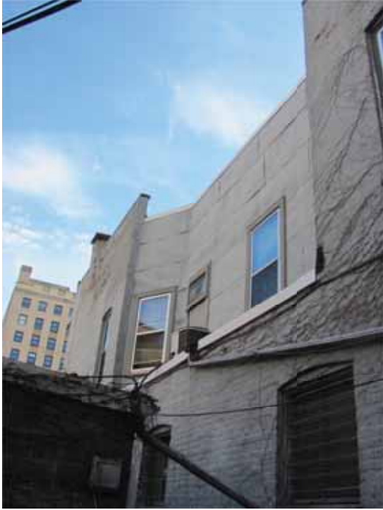
Figure 9. A portion of the side wall is recessed at the second floor and is clad with painted sheet metal.
