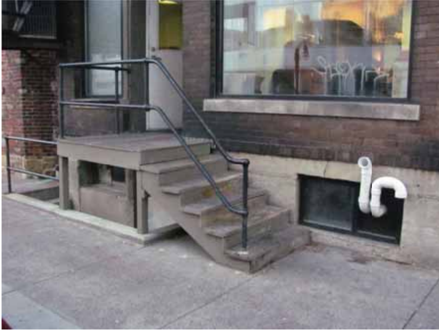
Figure 11. A painted wood stair and platform provide access to a first floor entrance door; there is a sunken well with an entrance door to the basement directly below.
