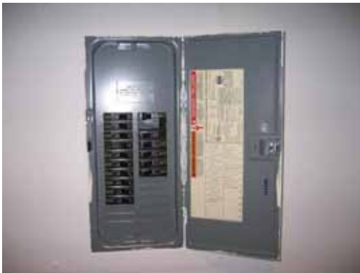
Electrical panel on 1 st floor retail.
