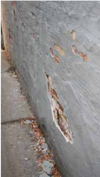
Exterior: View in the alley showing a section of delaminated parging
