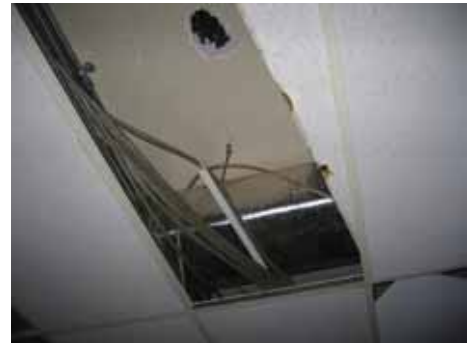
Electrical cables on 2 nd floor.
