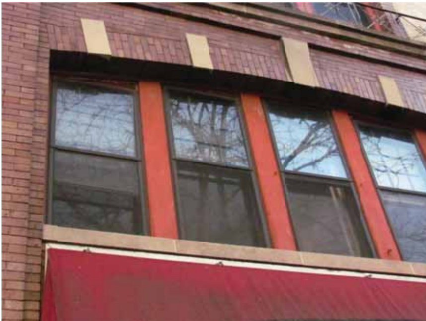
Figure 8. The upper floors of the building typically have original double-hung nine-over-one wood windows, covered by aluminum triple-track exterior storm windows.
