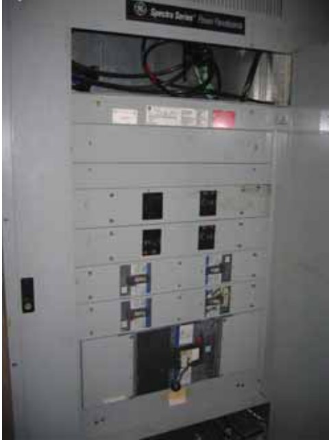
Distribution panel in the basement.
