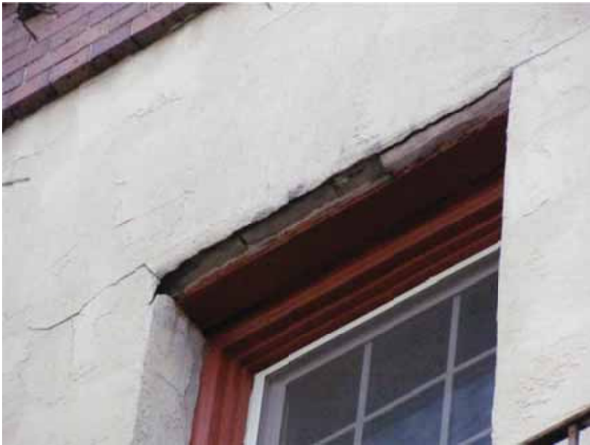
Figure 6. A portion of stucco has previously spalled at the head of the center third floor window.
