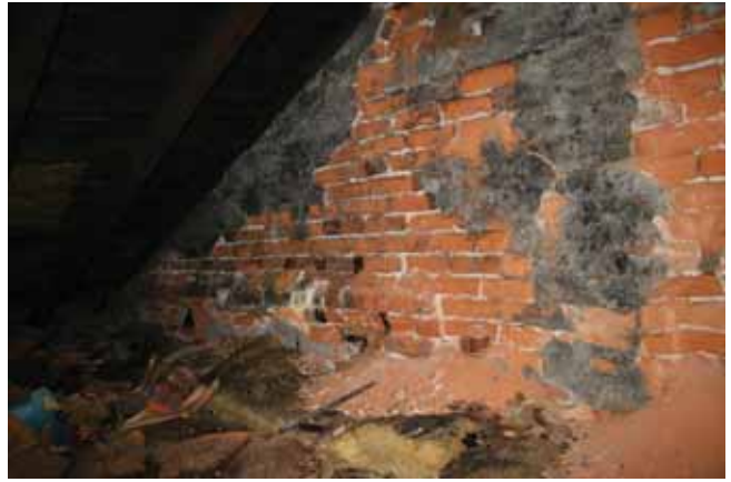
Attic: View toward wall between 127-129 state street and the castle and doyle building showing significant damage to existing brick
