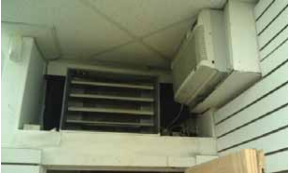
Corner retail heating and cooling
