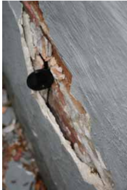
Exterior: View in the alley showing the delamination of the parging system from the brick veneer
