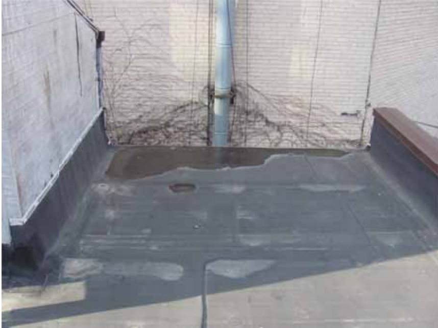
Figure 11. Ponding on the roof near the gutter.
