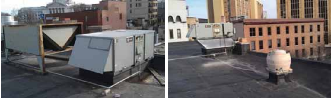
Existing rooftop equipment
