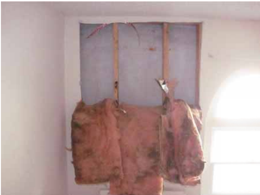
Figure 12. Staining and evidence of moisture penetration was observed on the batt insulation and plaster at an inspection opening created at the third floor during the site visit.
