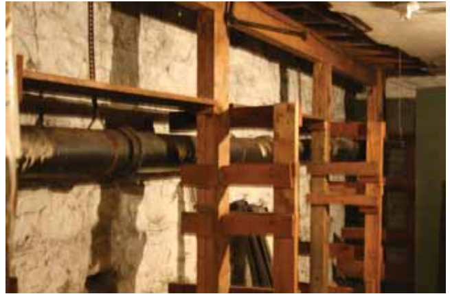
Basement view showing stormline routing storm water from adjacent building(s) through the basement of 120 West Mifflin Street
