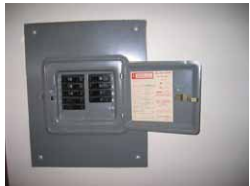
Electrical panel 125 1/2 State Street (2 nd floor apartment).
