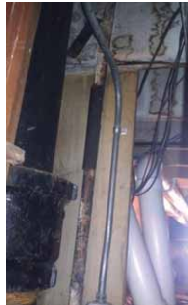
Failing storm main support
