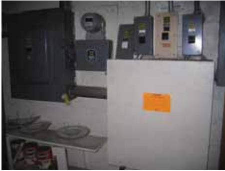
Electrical service in the basement.
