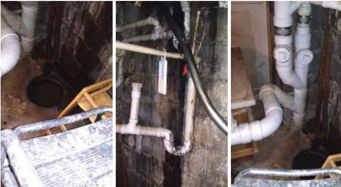
Poor condition of sanitary piping
