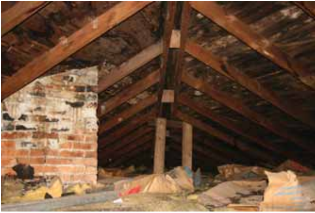
Attic: View toward flat iron corner showing damage to chimney
