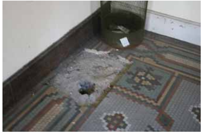
First Floor: View at back of room where the floor has been removed
