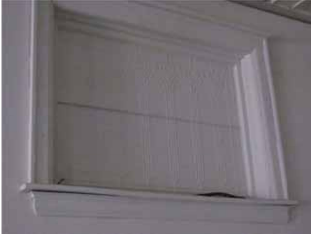
Figure 17. Leaded glass window, which has been painted over, at the southwest party wall.
