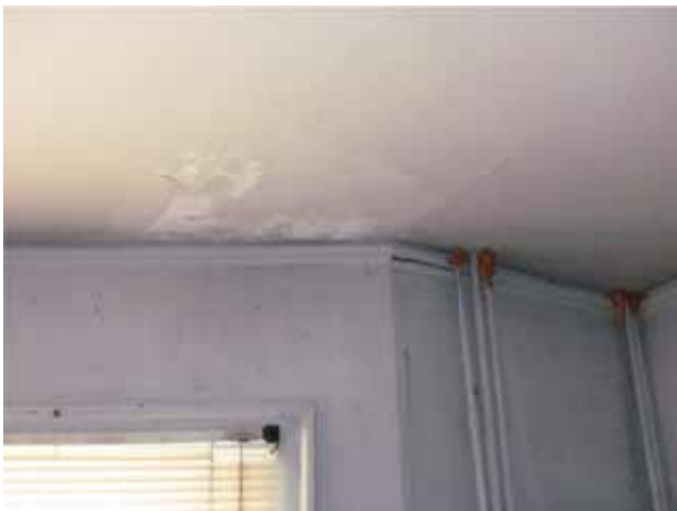
Figure 19. Moisture damage to plaster finishes at the second floor.
