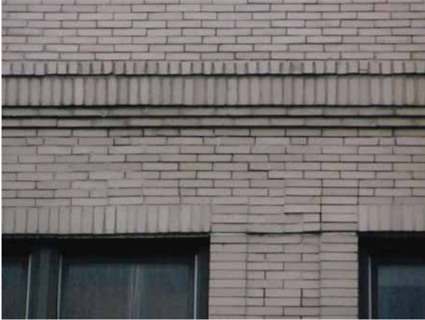
Figure 5. Cracking and displacement of brick masonry above window heads.
