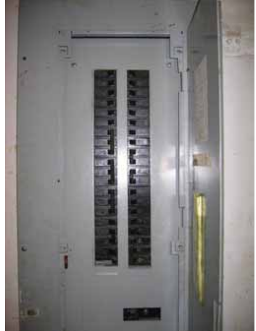
Electrical panel on 1 st floor restaurant.
