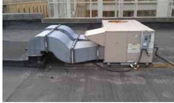
One of two packaged rooftop units
