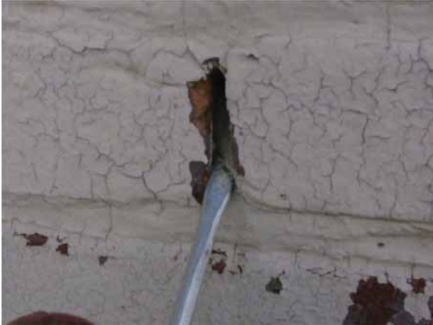
Figure 5. Mortar behind the coating layers is friable and has disintegrated.
