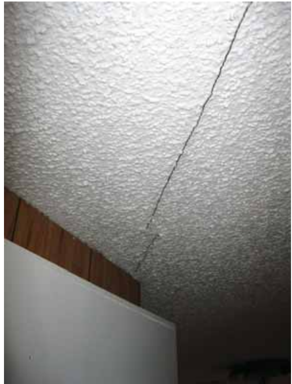
Photo 13 – Ceiling finish distress beneath roof
