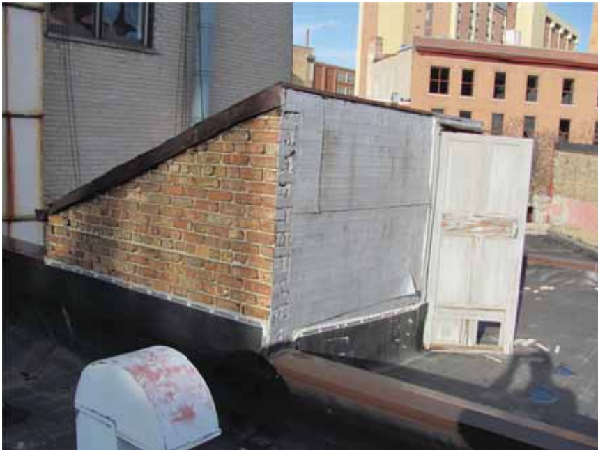
Figure 12. View of the penthouse walls constructed of brick masonry and painted sheet metal.
