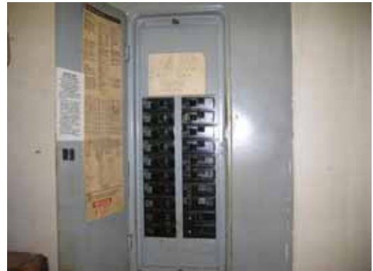
Electrical panel in 127 State Street (First Floor).
