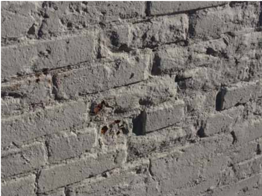
Figure 4. The coating layers were applied over unrepaired deteriorated masonry.
