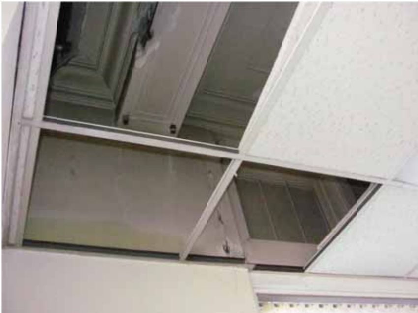
Figure 9. The original plaster ceiling and cornice are present above the suspended acoustical ceiling system. Also note the original transoms at the first floor storefront.
