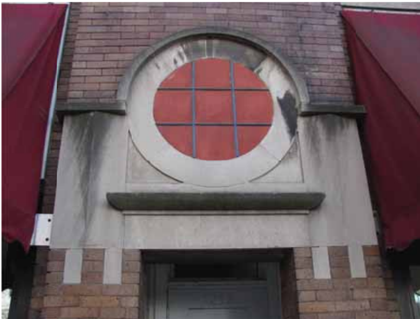
Figure 2. A circular opening above the entrance door to the apartments has been infilled with painted plywood.
