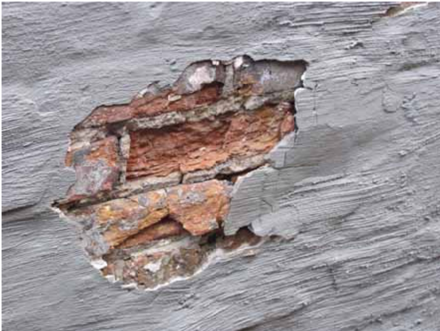
Figure 5. Failure of cementitious parge coat, revealing deteriorated brick masonry.
