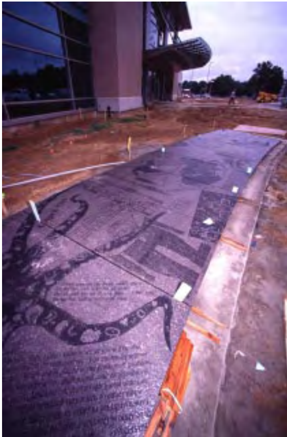
Example of granite scroll being installed in Memphis. Design by Brad Goldberg
