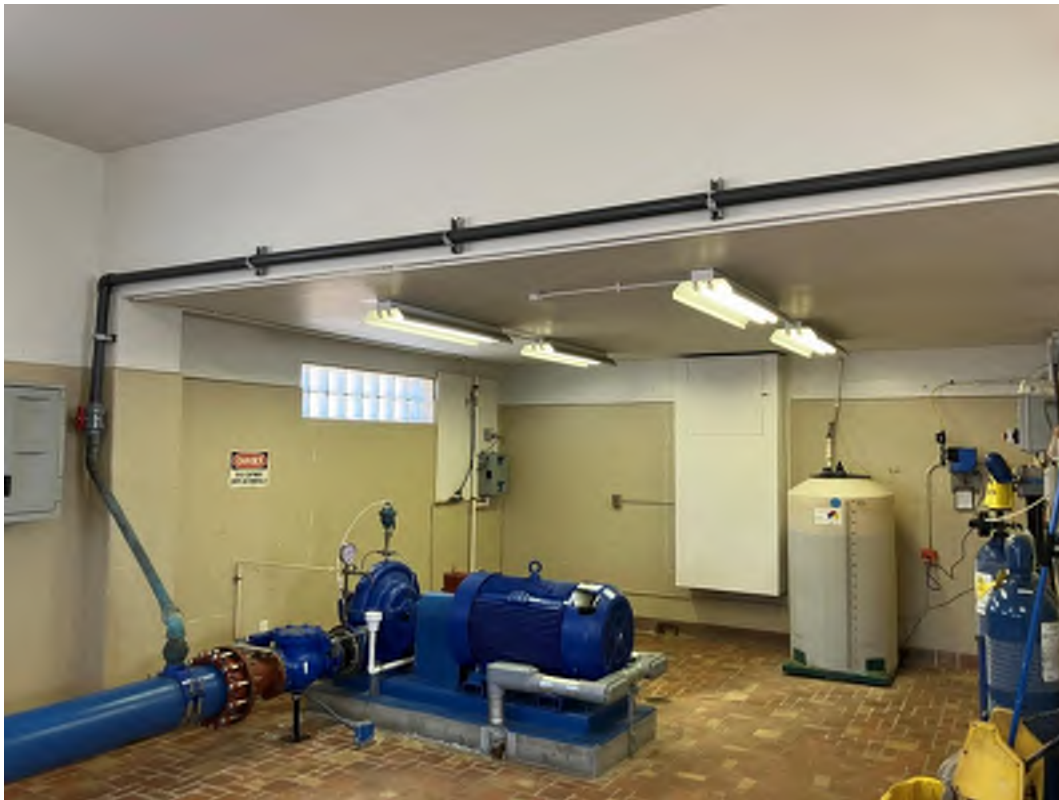
Interior of existing Wellhouse.
