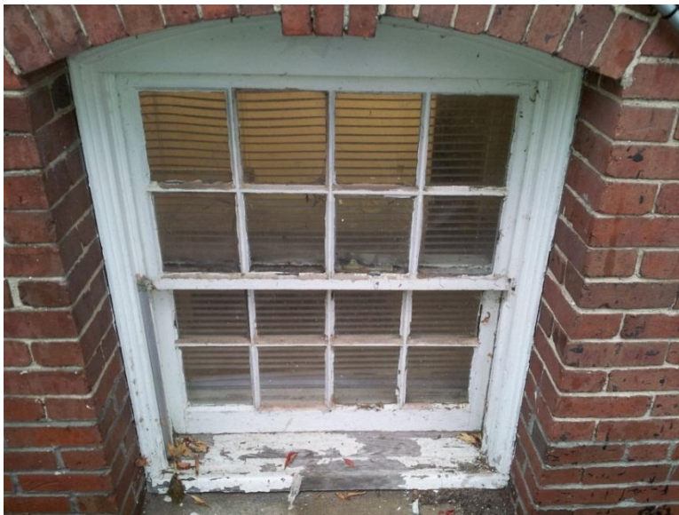
Image 1.26 Rapidly deteriorating wood windows without aluminum combination storms that have protected other windows from the elements.
