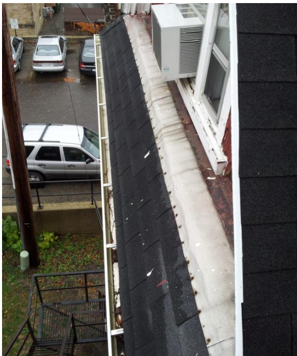
Image 1.9 Gutters and downspouts consist of prefinished sheet metal; they are sound. They appear newer and could possibly be reclaimed
