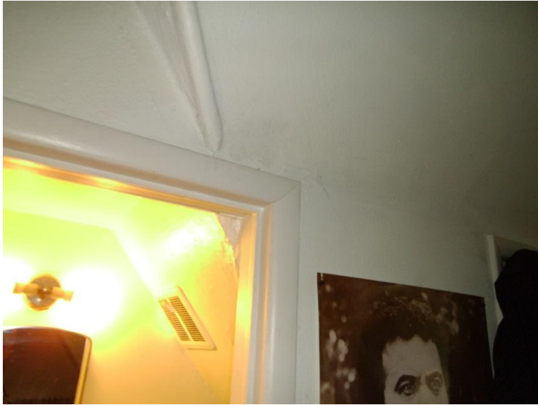
Image 1.10 View showing a valley rafter crossing an interior wall at a doorway. Note the doorway appears to cut through the bottom of the rafter.
