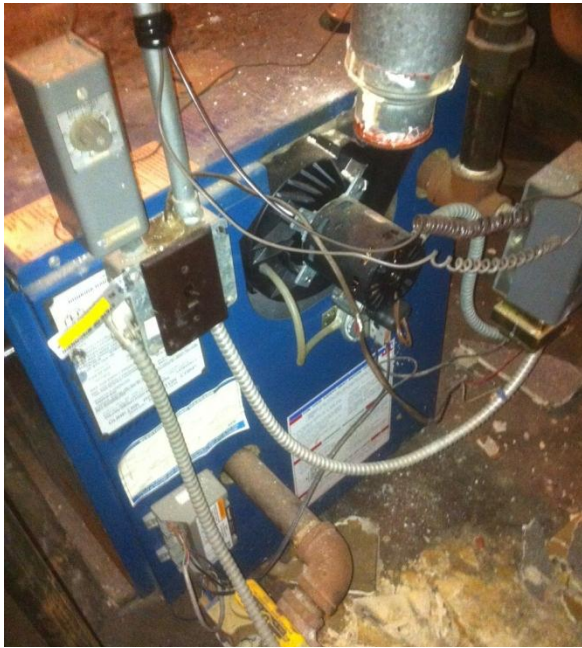
Image 1.17 Dunkirk boiler in the basement mechanical room.
