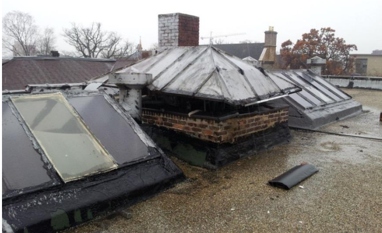
Image 1.28 Roof appurtenances and conditions. Glazing of the skylights is largely intact but fractured. Leaks to the interior were observed.
