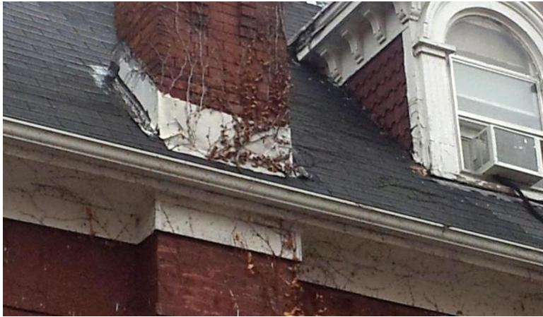
Image 1.6 The eave system consists of original painted (finished) wood members, including eave and rake boards (fascia), crown, and soffit. The condition is largely sound.
