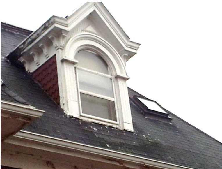
Image 1.4 The gables and dormer walls originally featured beaded board and shingle siding and major portions of these areas are presently exposed and functioning. Areas exposed to view appear to be rotting and otherwise deteriorating
