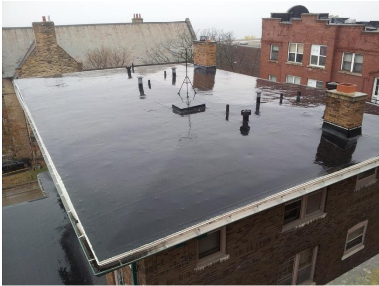
Image 1.43 The roof is a flat (low-slope), deep-eave design consisting of an exposed layer of EPDM (rubber) material, and it likely contains tapered rigid insulation beneath it, forming a hipped-roof surface for drainage.
