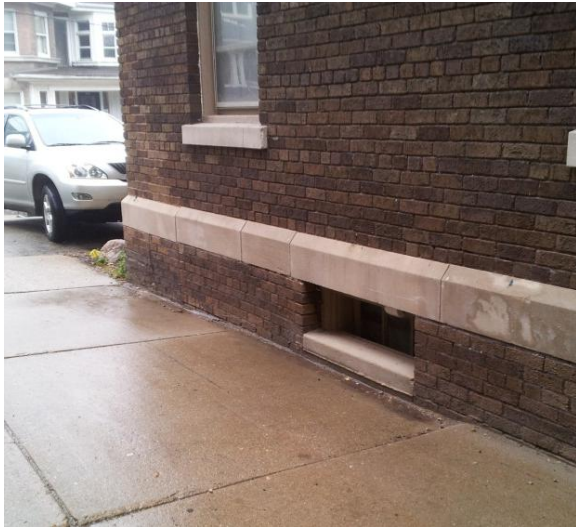
Image 1.39 View of concrete driveway pitched towards foundation wall allowing rain and snow melt water to enter basement area.
