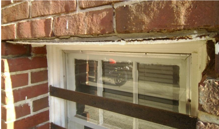
Image 1.22 View of one of the window lintels illustrating rust jacking.
