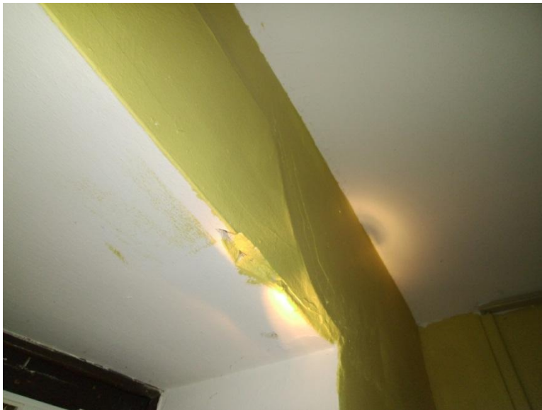
Image 1.29 View showing possible shear failure in a support lintel below the larger openings of the bay within an apartment. The side bay windows align and occur on each of levels 2 – 4.
