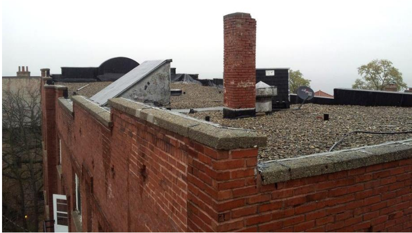
Image 1.59 The roof is a low-slope design consisting of a stone-ballasted EPDM (rubber) membrane bordered with continuous brick masonry parapets with precast concrete caps.
