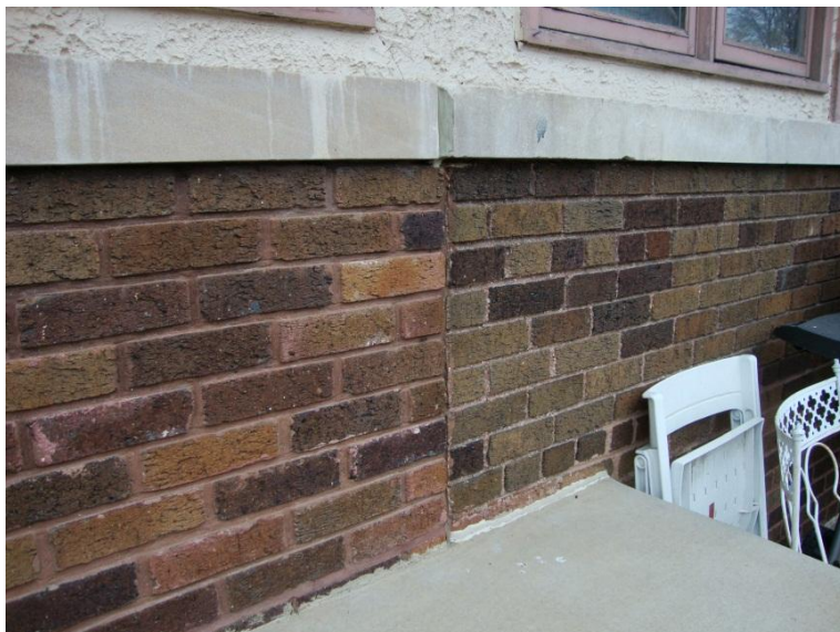
Image 1.41 View of infill brick at front porch. Enough evidence of original conditions remains to restore this porch if desired.
