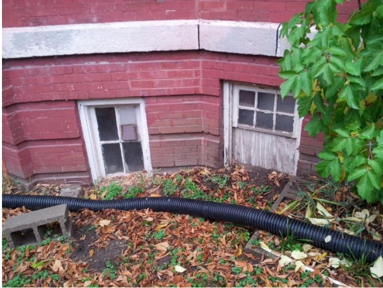
Image 1.2 View of the west side at grade. Moisture is penetrating the perimeter walls below-grade at this and other locations
