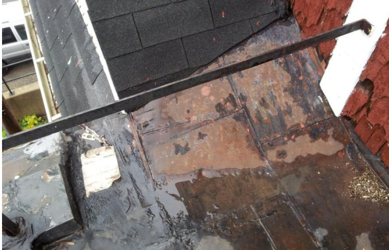
Image 1.8 A combination of roofing systems and wall cladding intersect here. The condition is unsound and moisture penetration is occurring
