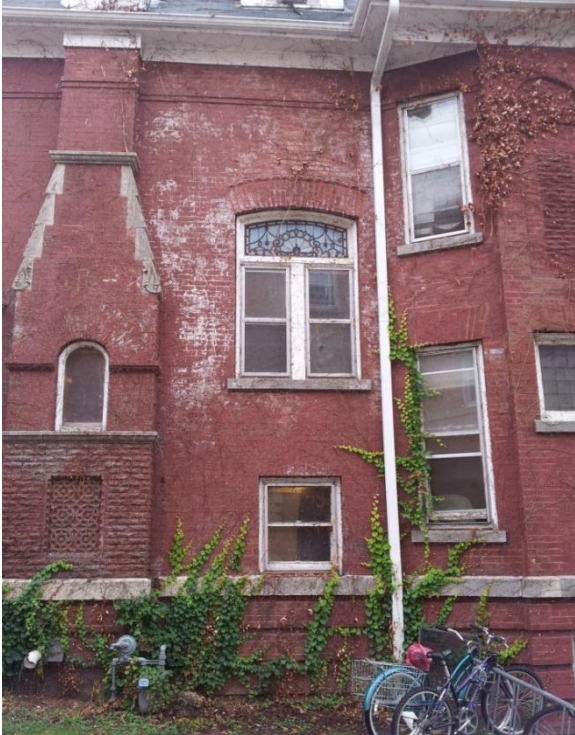
Image 1.3 The brick masonry observed is largely in good condition, but it contains evidence of minor instability in the form of step-cracking. There is also efflorescence at several locations indicating moisture penetration of the masonry.
