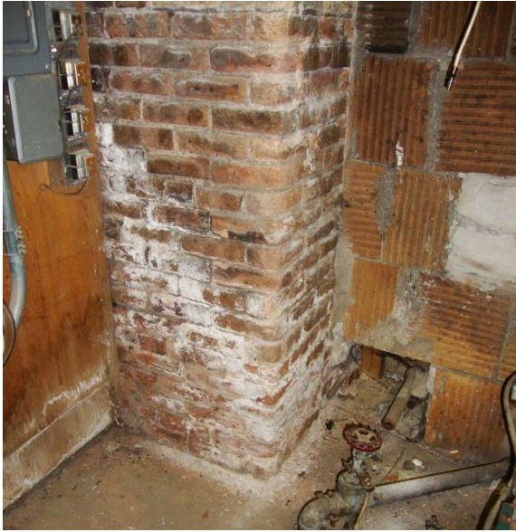
Image 1.38 View of efflorescence in the mechanical room along the exterior wall evidence of water penetration.
