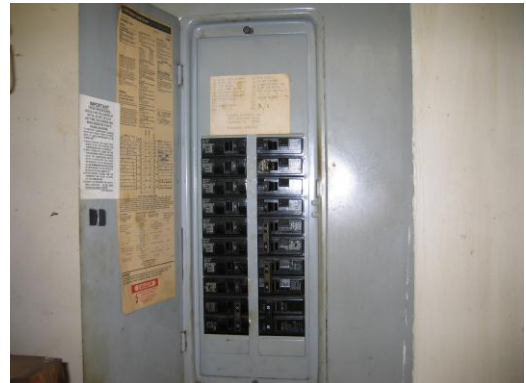
Electrical panel in 127 State Street (First Floor).
