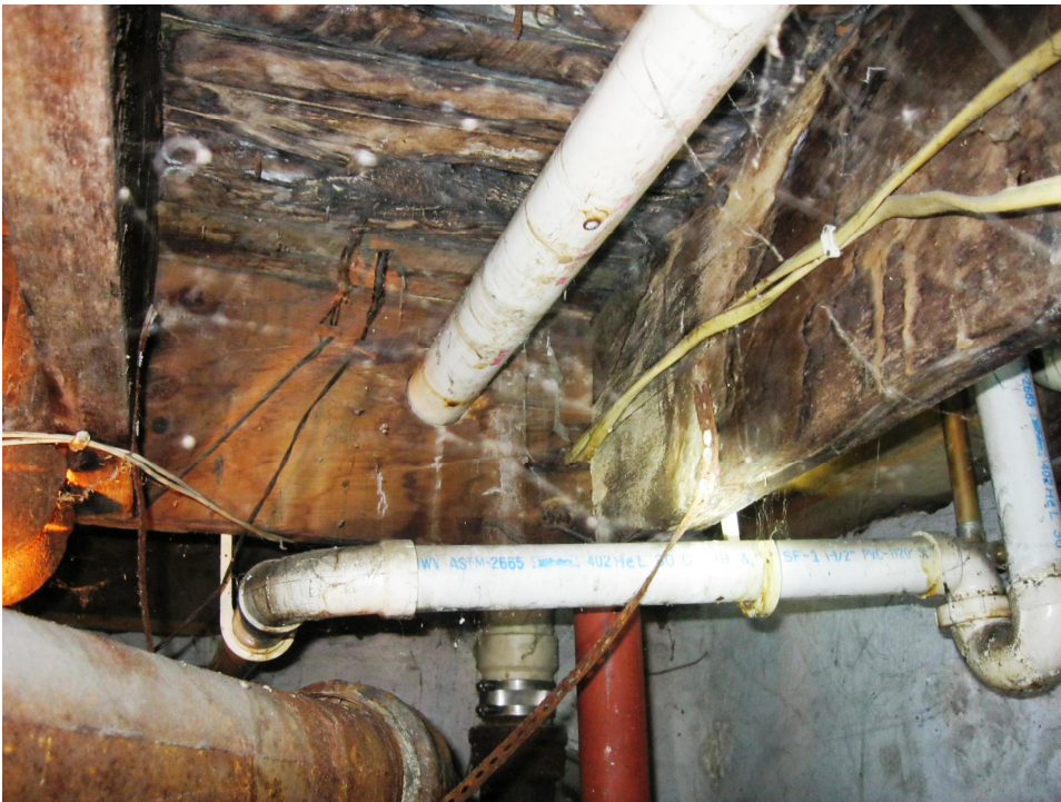
Photo 7 – 1 st floor framing with water damage
