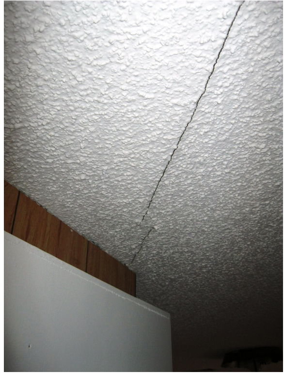
Photo 13 – Ceiling finish distress beneath roof
