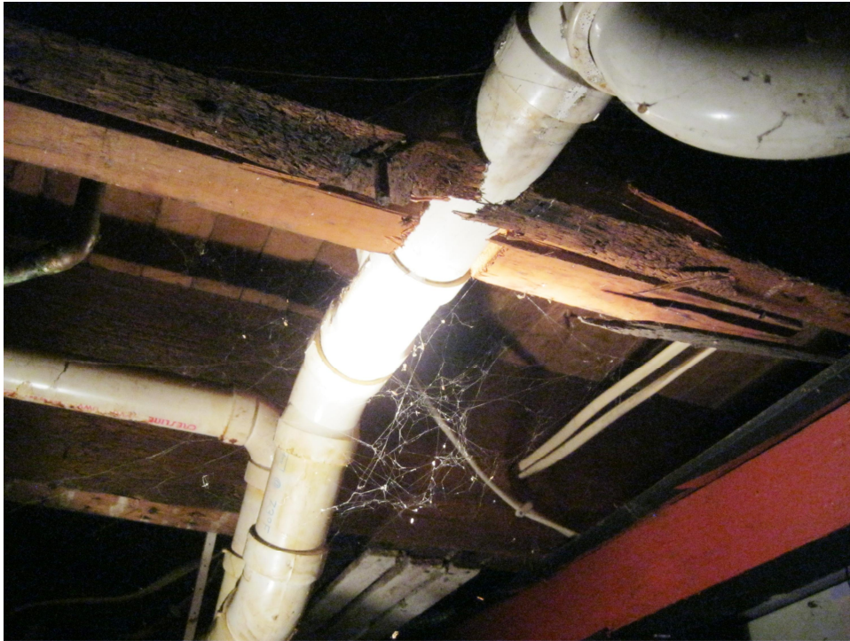
Photo 8 – 1 st floor framing notched for plumbing
