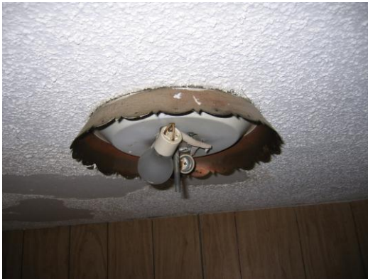
Light fixture in 119 North Fairchild Street (2 nd floor apartment.)
