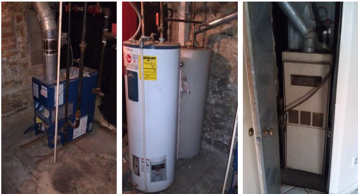
Boilers, water heaters, and furnace
