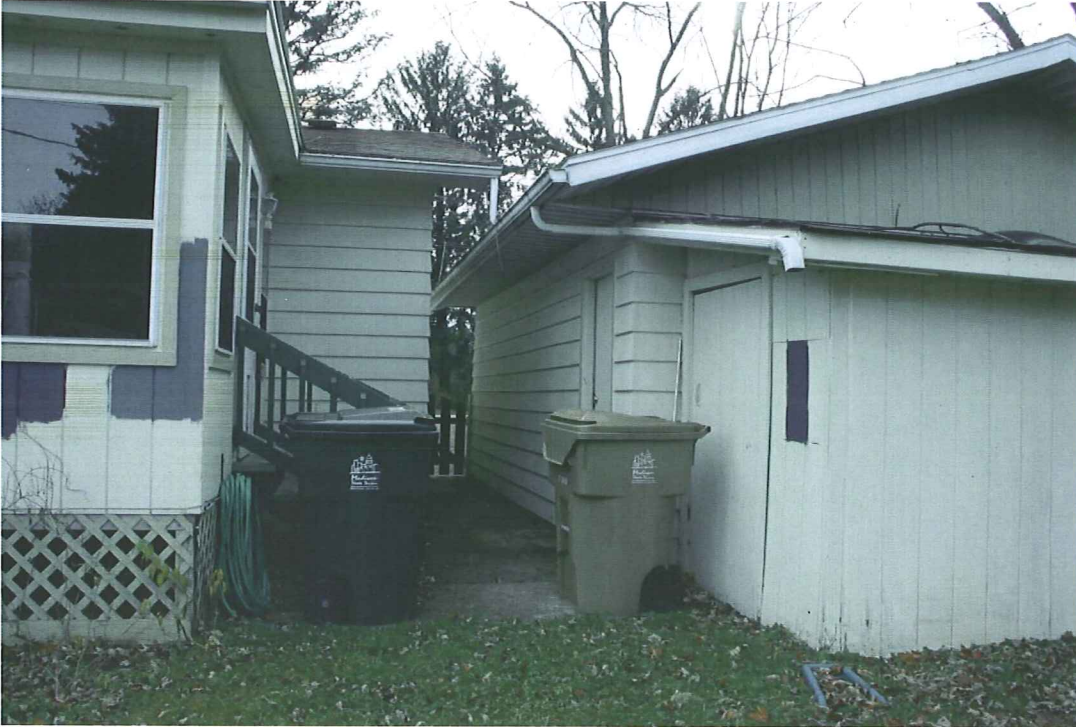
4908 Three season porch and garage (rear of building) Lean-to shed is in need of re-building
