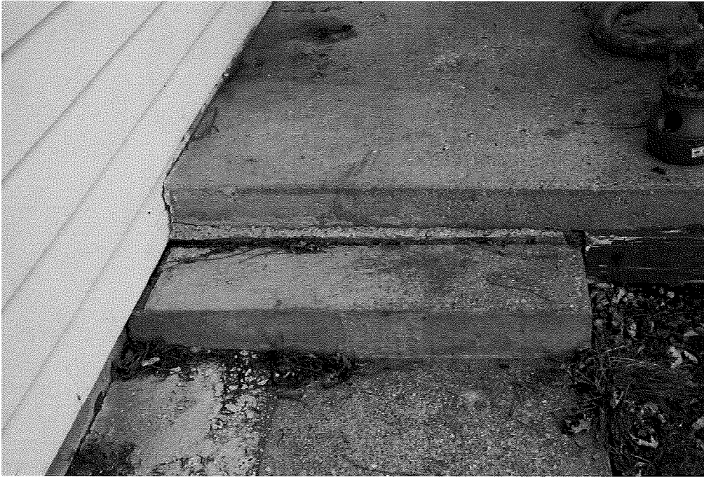
4908 Entrance steps and sidewalk – replacement is recommended
