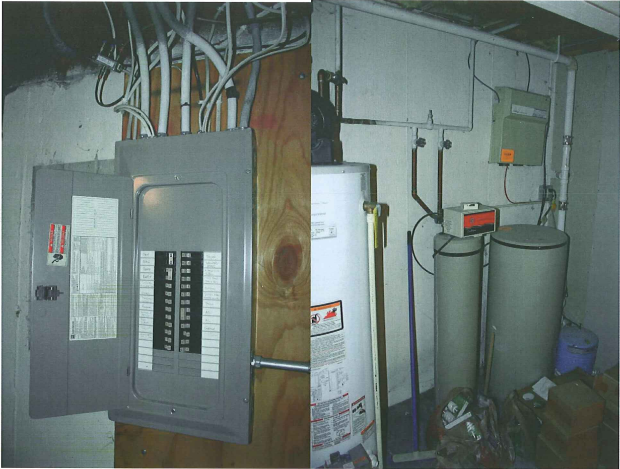
4908 Electrical service and water heater/softener
